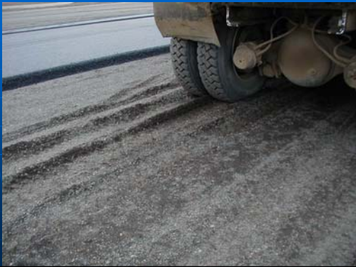
RAP base course rutting as trucks back up to paver.
