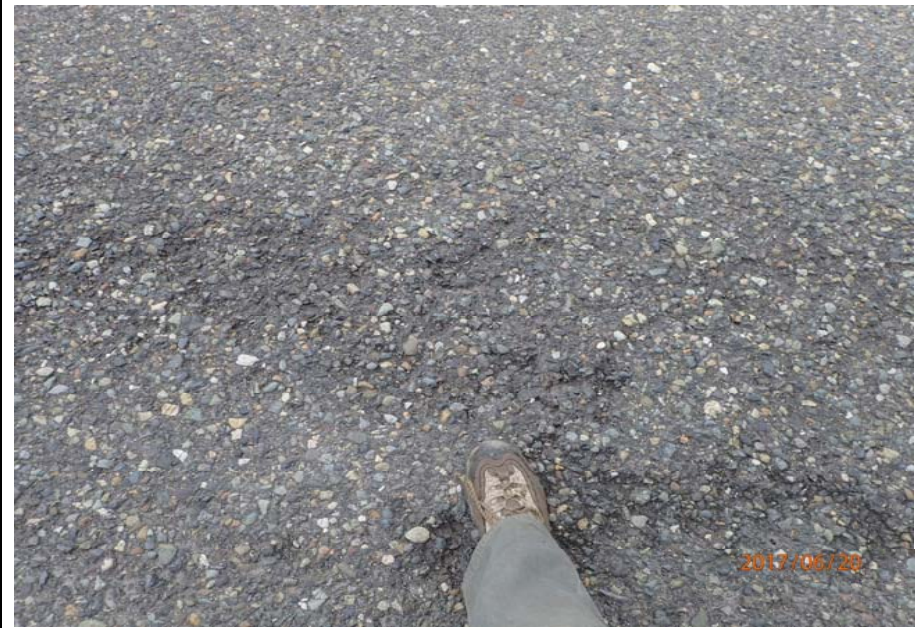
Bridge No. 0747 Br. Name Ward Creek Date 06/20/17 Inspector Manning / McRae Frame 6 Wearing surface condition in wheel lines, typical
