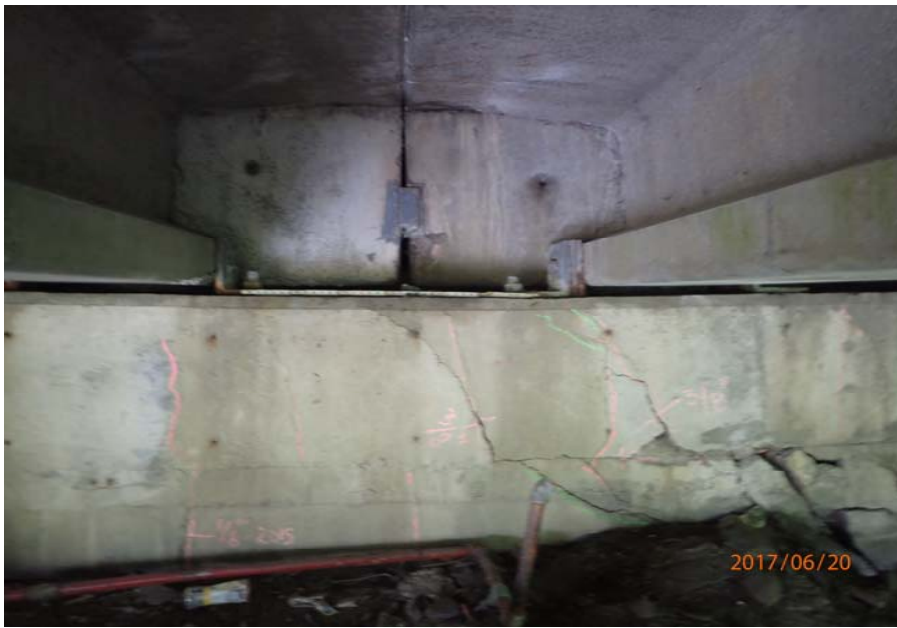
Bridge No. 0747 Br. Name Ward Creek Date 06/20/17 Inspector Manning / McRae Frame 21 FE abutment, 2nd bay from RT
