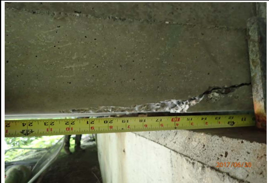
Bridge No. 0747 Br. Name Ward Creek Date 06/20/17 Inspector Manning / McRae Frame 24 FE abutment, 2nd bay from RT, G4 RT side crack in bottom flange
