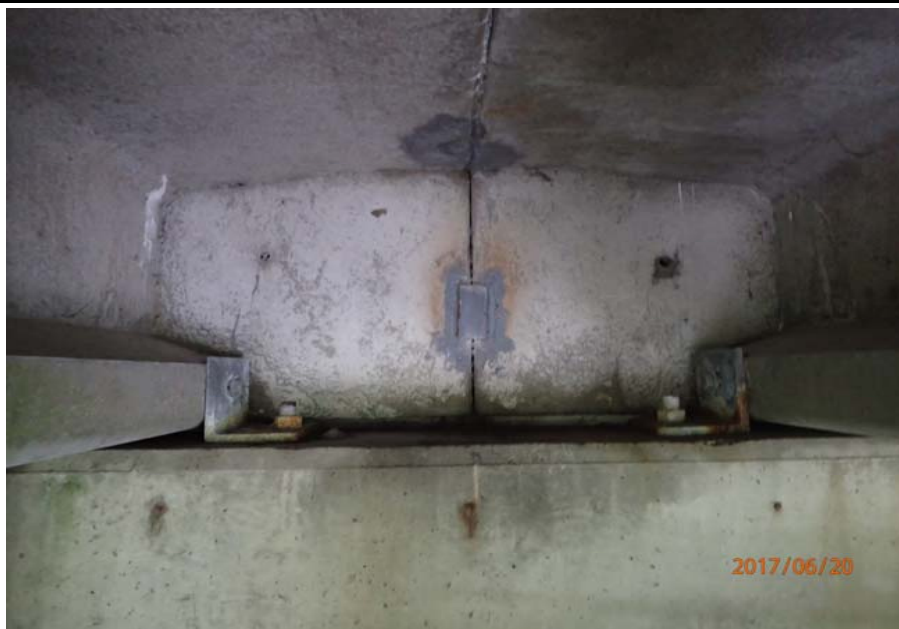
Bridge No. 0747 Br. Name Ward Creek Date 06/20/17 Inspector Manning / McRae Frame 27 FE, 4th bay from RT, spall in bottom of deck at backwall
