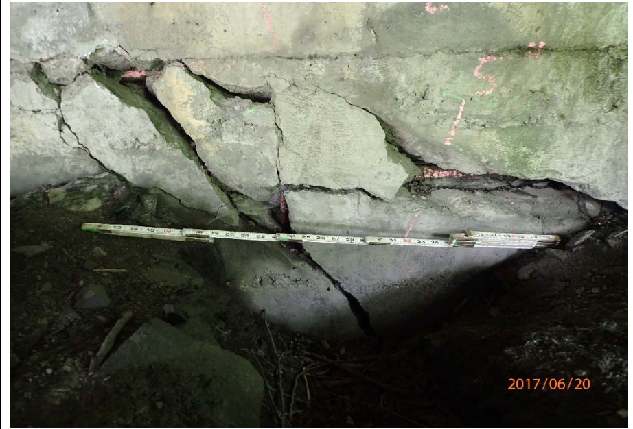
Bridge No. 0747 Br. Name Ward Creek Date 06/20/17 Inspector Manning / McRae Frame 18 FE abutment, RT bay, close up of cap damage, exposed rebar
