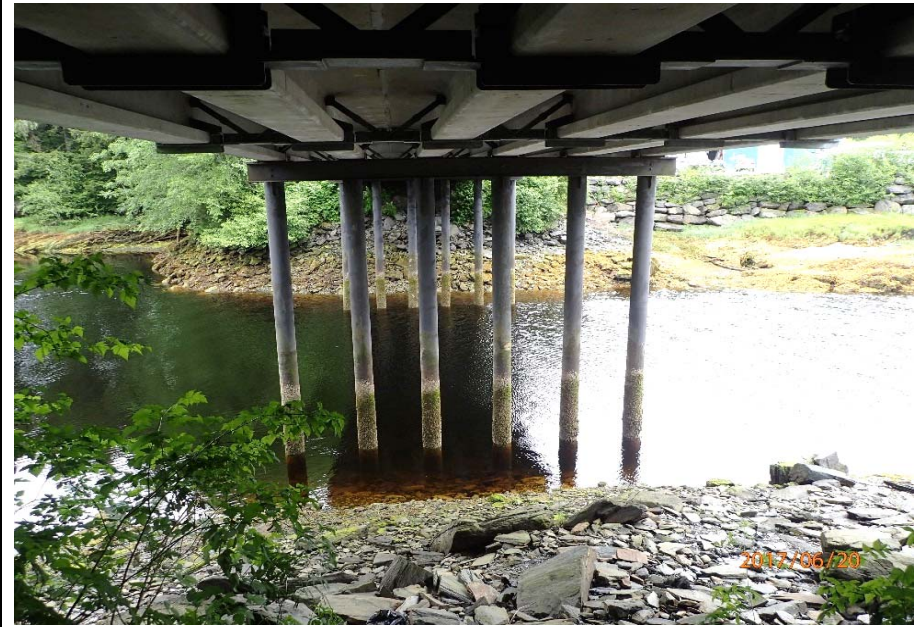
Bridge No. 0747 Br. Name Ward Creek Date 06/20/17 Inspector Manning / McRae Frame 10 FE Bent 3
