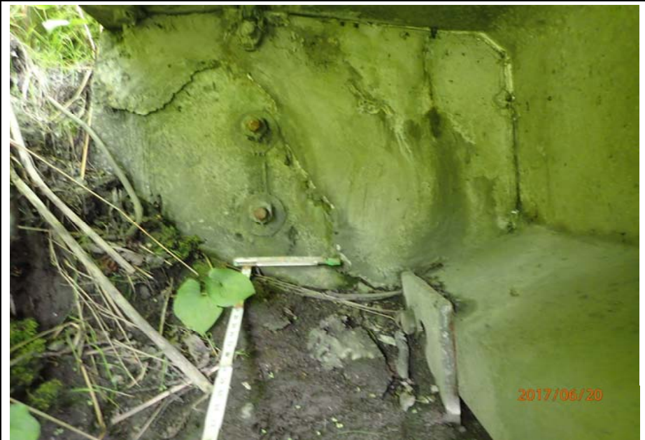
Bridge No. 0747 Br. Name Ward Creek Date 06/20/17 Inspector Manning / McRae Frame 32 NE RT corner, spalls in backwall
