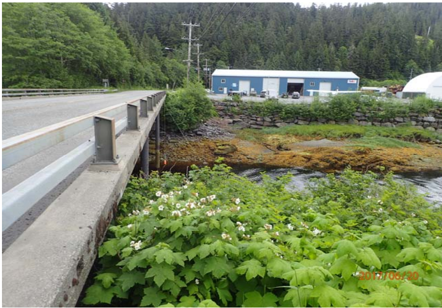
Bridge No. 0747 Br. Name Ward Creek Date 06/20/17 Inspector Manning / McRae Frame 5 LT elevation (FE LT looking NE)
