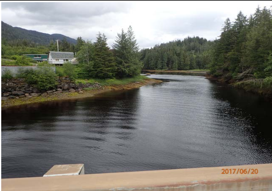
Bridge No. 0747 Br. Name Ward Creek Date 06/20/17 Inspector Manning / McRae Frame 3 Looking RT
