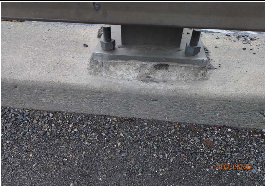
Bridge No. 0747 Br. Name Ward Creek Date 06/20/17 Inspector Manning / McRae Frame 35 Damaged grout pads, typical of span 2 LT
