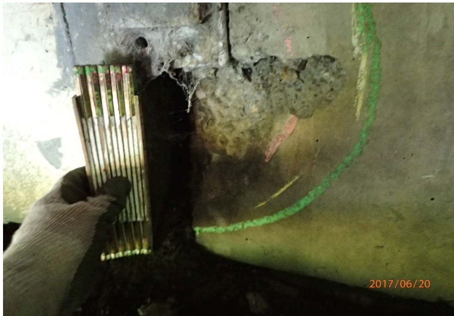
Bridge No. 0747 Br. Name Ward Creek Date 06/20/17 Inspector Manning / McRae Frame 25 FE abutment, 2nd bay from RT, spall in backwall
