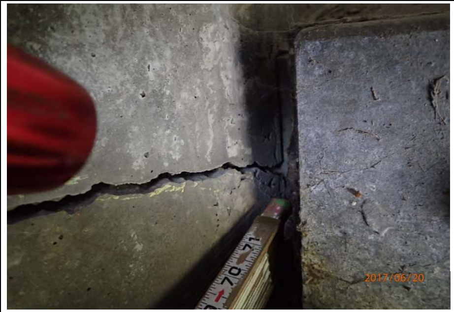
Bridge No. 0747 Br. Name Ward Creek Date 06/20/17 Inspector Manning / McRae Frame 20 FE abutment, RT bay, terminus of backwall crack behind girder bottom flange
