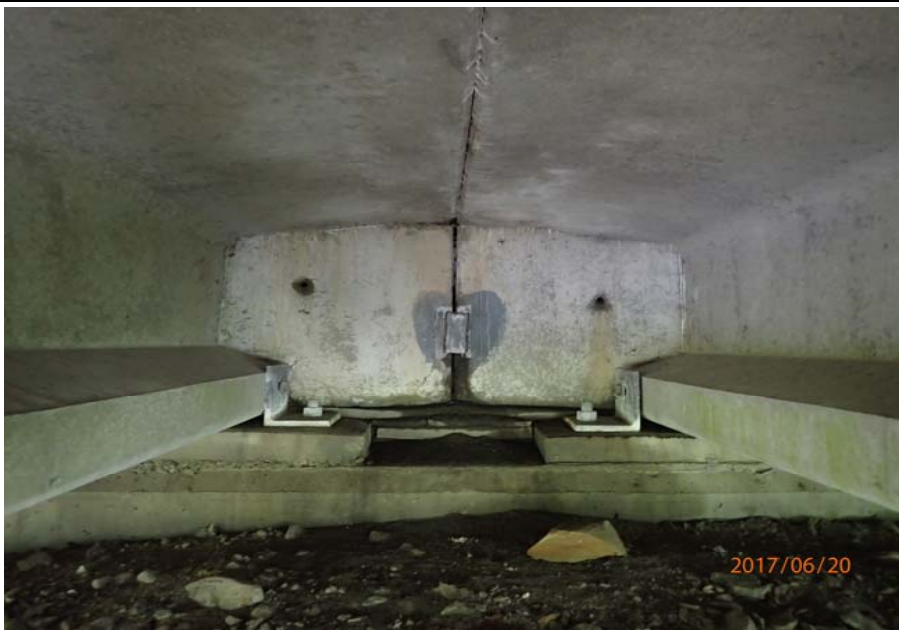
Bridge No. 0747 Br. Name Ward Creek Date 06/20/17 Inspector Manning / McRae Frame 11 Typical backwall (NE shown)
