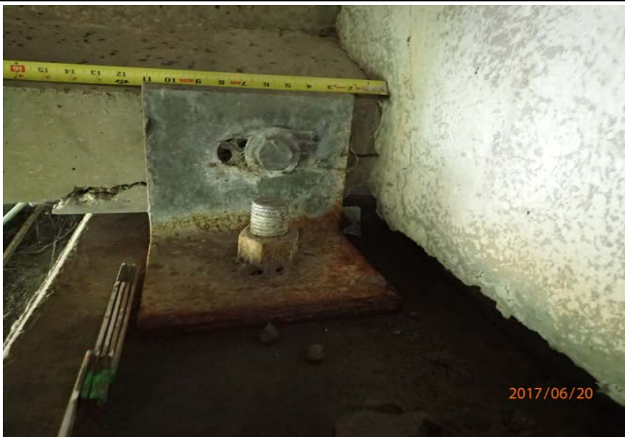
Bridge No. 0747 Br. Name Ward Creek Date 06/20/17 Inspector Manning / McRae Frame 23 FE abutment, 2nd bay from RT, G4 RT side crack in bottom flange
