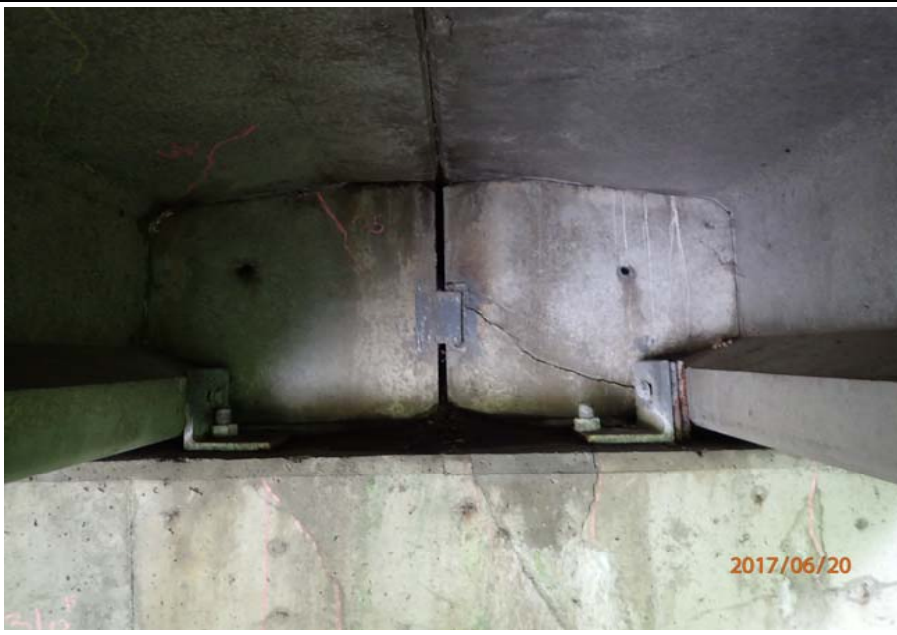
Bridge No. 0747 Br. Name Ward Creek Date 06/20/17 Inspector Manning / McRae Frame 19 FE abutment, RT bay, backwall
