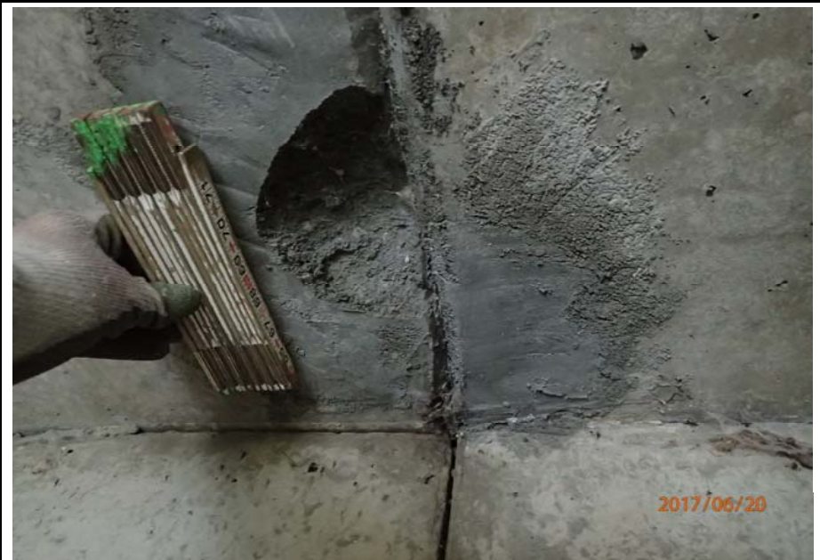
Bridge No. 0747 Br. Name Ward Creek Date 06/20/17 Inspector Manning / McRae Frame 28 FE, 4th bay from RT, spall in bottom of deck at backwall
