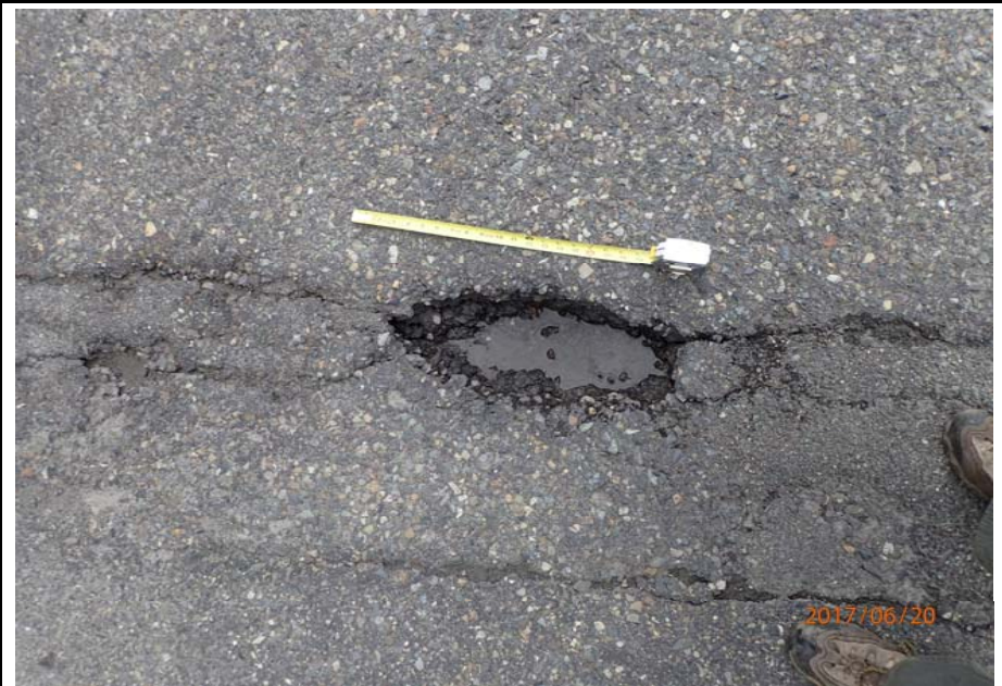
Bridge No. 0747 Br. Name Ward Creek Date 06/20/17 Inspector Manning / McRae Frame 36 FE LT lane, pothole at joint
