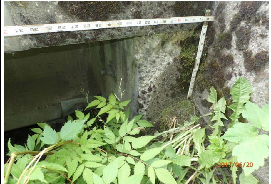
Bridge No. 0747 Br. Name Ward Creek Date 06/20/17 Inspector Manning / McRae Frame 30 FE RT spall in hider wall
