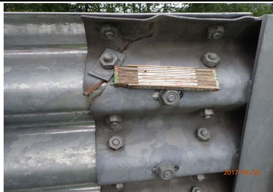
Bridge No. 0747 Br. Name Ward Creek Date 06/20/17 Inspector Manning / McRae Frame 16 FE LT transition rail damage
