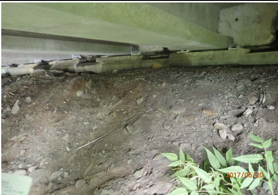
Bridge No. 0747 Br. Name Ward Creek Date 06/20/17 Inspector Manning / McRae Frame 7 NE abutment
