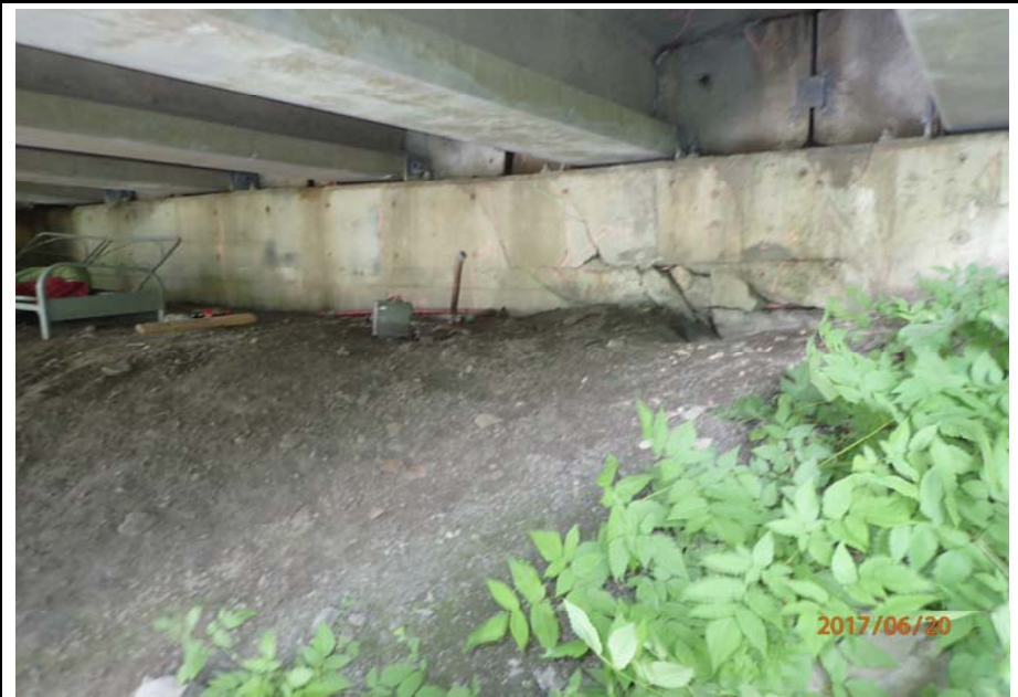
Bridge No. 0747 Br. Name Ward Creek Date 06/20/17 Inspector Manning / McRae Frame 8 FE abutment
