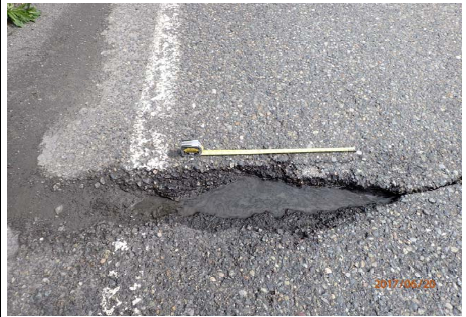
Bridge No. 0747 Br. Name Ward Creek Date 06/20/17 Inspector Manning / McRae Frame 34 NE RT lane, pothole at joint
