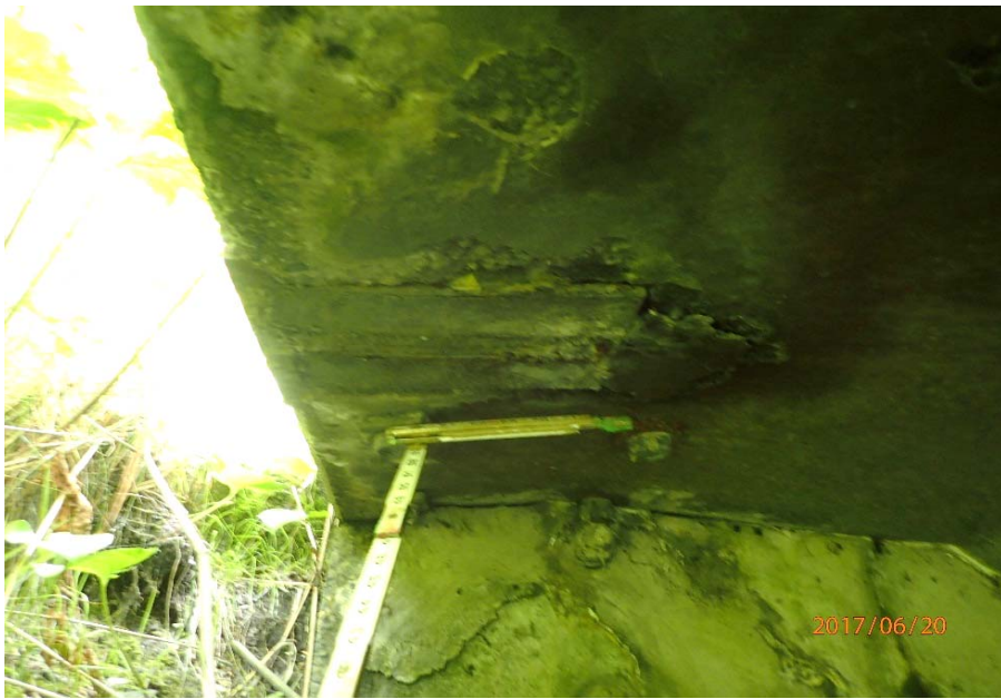
Bridge No. 0747 Br. Name Ward Creek Date 06/20/17 Inspector Manning / McRae Frame 33 NE RT corner, spall in soffit
