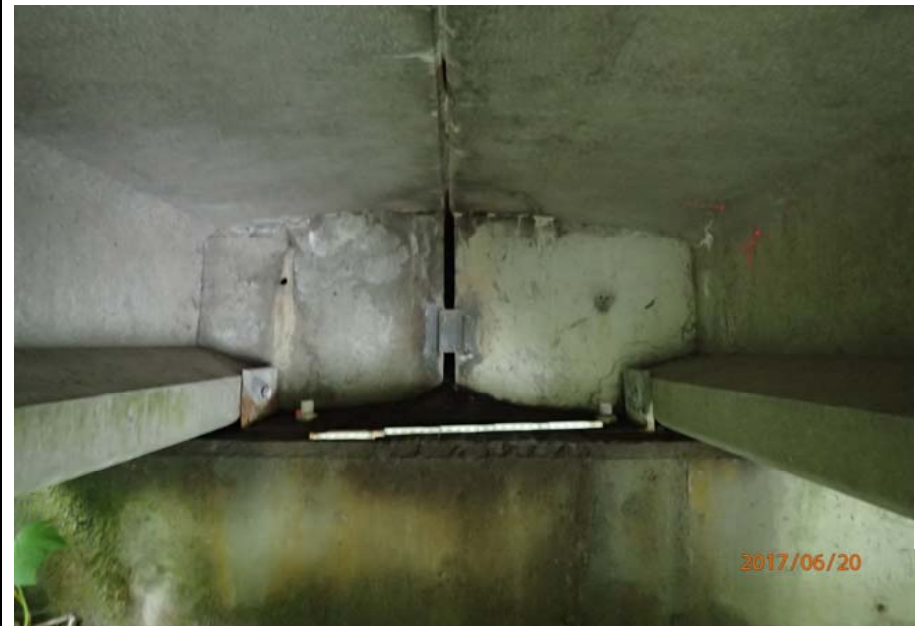
Bridge No. 0747 Br. Name Ward Creek Date 06/20/17 Inspector Manning / McRae Frame 26 Fill coming through backwall typical (FE abutment, LT bay shown)
