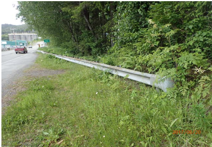
Bridge No. 0747 Br. Name Ward Creek Date 06/20/17 Inspector Manning / McRae Frame 13 NE RT end treatment buried in hill
