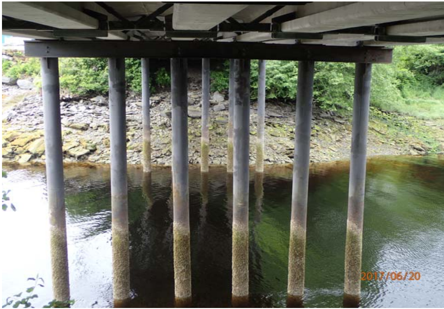
Bridge No. 0747 Br. Name Ward Creek Date 06/20/17 Inspector Manning / McRae Frame 9 NE Bent 2
