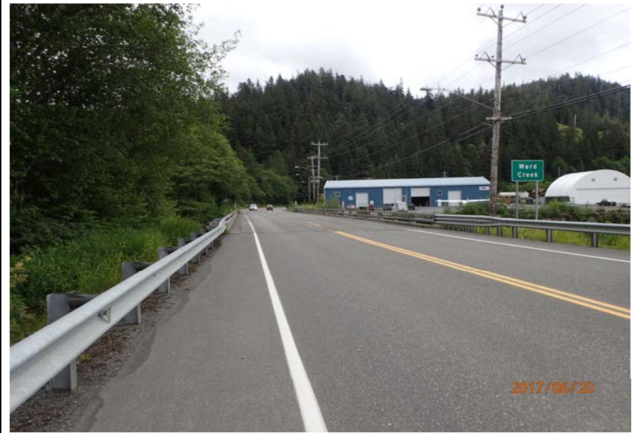
Bridge No. 0747 Br. Name Ward Creek Date 06/20/17 Inspector Manning / McRae Frame 2 Back at bridge
