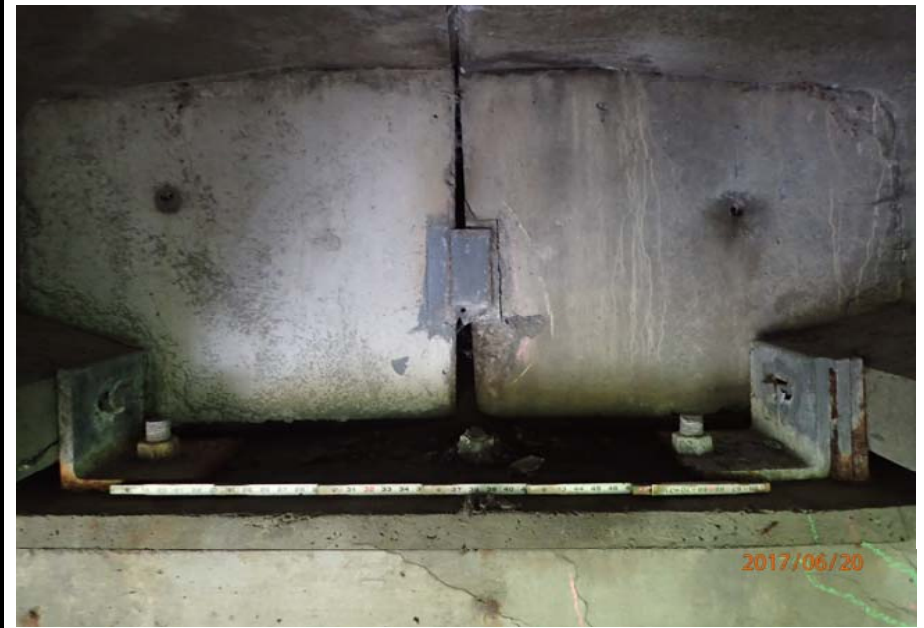
Bridge No. 0747 Br. Name Ward Creek Date 06/20/17 Inspector Manning / McRae Frame 22 FE abutment, 2nd bay from RT, backwall
