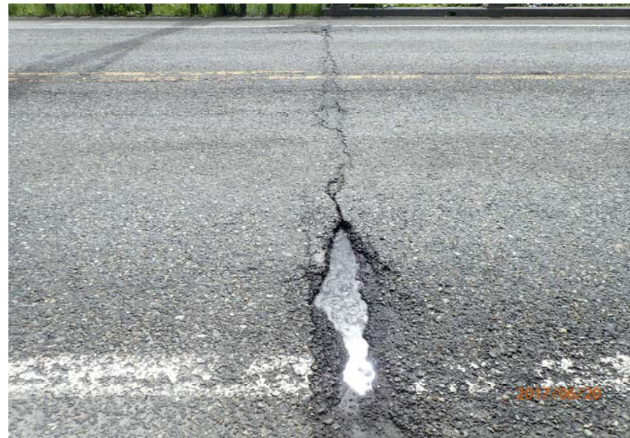
Bridge No. 0747 Br. Name Ward Creek Date 06/20/17 Inspector Manning / McRae Frame 14 NE joint, potholes in RT lane
