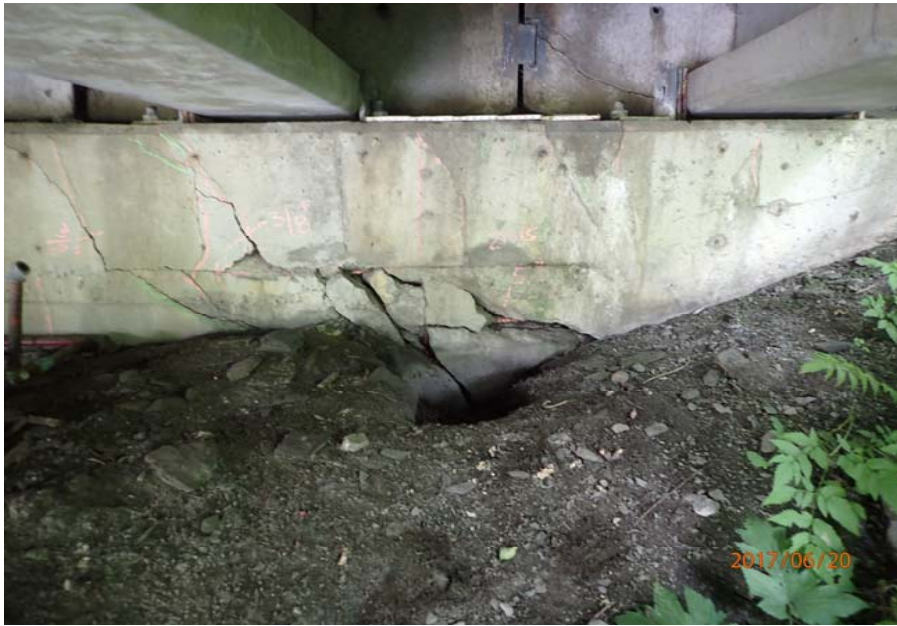
Bridge No. 0747 Br. Name Ward Creek Date 06/20/17 Inspector Manning / McRae Frame 17 Damage to cap and backwall at FE RT bay
