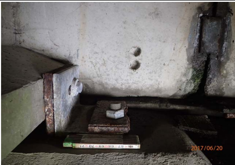
Bridge No. 0747 Br. Name Ward Creek Date 06/20/17 Inspector Manning / McRae Frame 31 NE RT girder anchor showing rust and section loss
