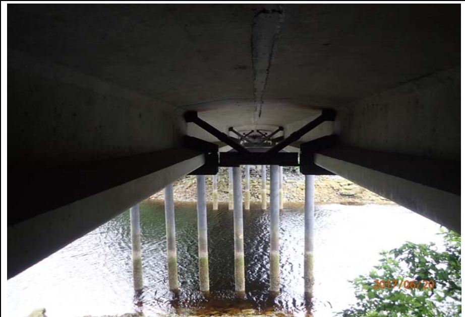
Bridge No. 0747 Br. Name Ward Creek Date 06/20/17 Inspector Manning / McRae Frame 12 Typical bay (FE shown)
