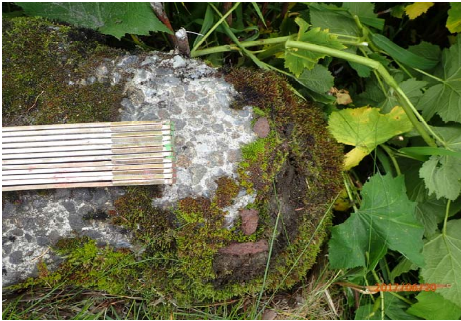
Bridge No. 0747 Br. Name Ward Creek Date 06/20/17 Inspector Manning / McRae Frame 29 FE LT wingwall spall with exposed rebar
