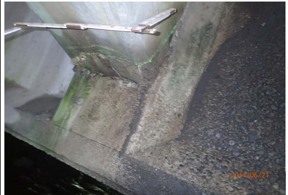
Bridge No. 0725 Br. Name Hoadley Creek Date 06/21/17 Inspector Manning / McRae Frame 34 Crack bottom US cantilever support #3 (RT/LT faces are sides # 5 & 6)
