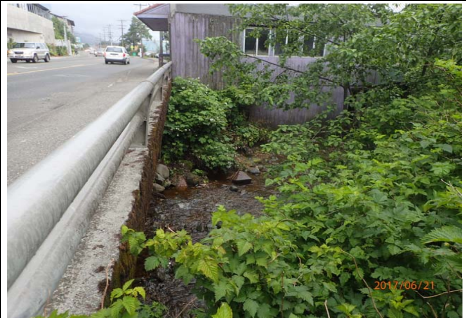
Bridge No. 0725 Br. Name Hoadley Creek Date 06/21/17 Inspector Manning / McRae Frame 48 Typical rail and NE DS bank
