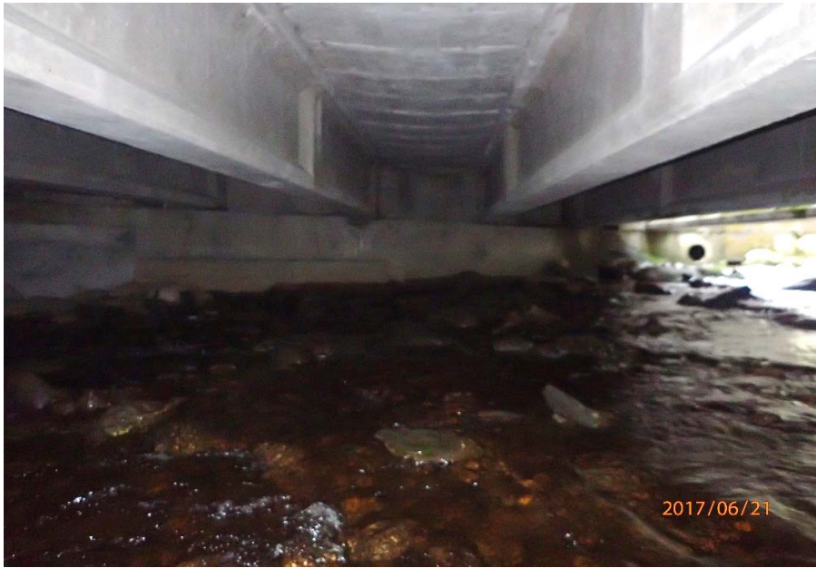
Bridge No. 0725 Br. Name Hoadley Creek Date 06/21/17 Inspector Manning / McRae Frame 13 FE abutment (US)
