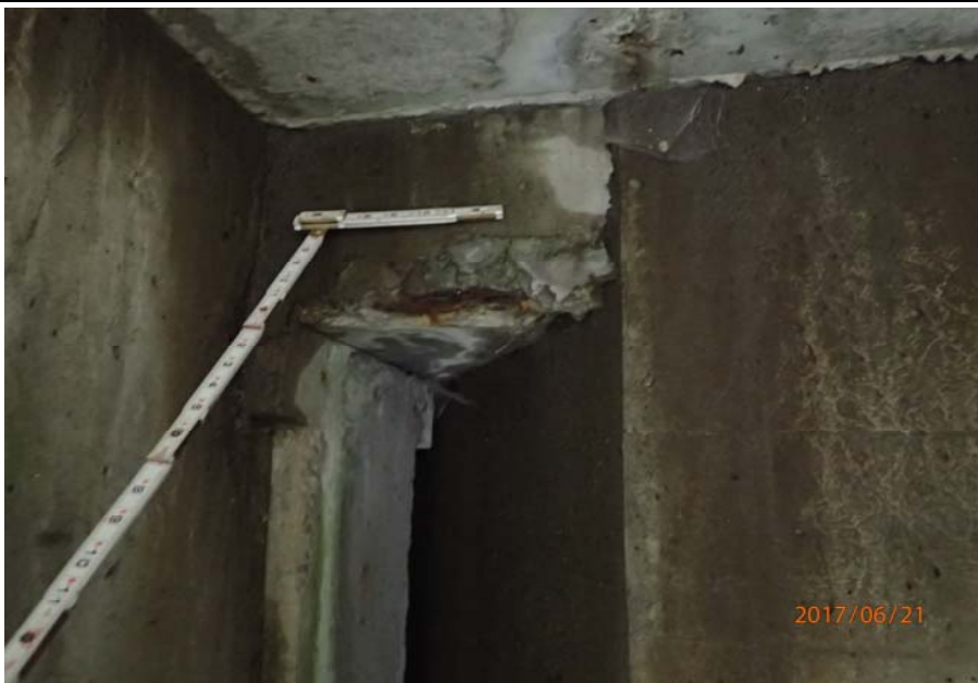
Bridge No. 0725 Br. Name Hoadley Creek Date 06/21/17 Inspector Manning / McRae Frame 19 FE US girder at abutment, spall with exposed rebar
