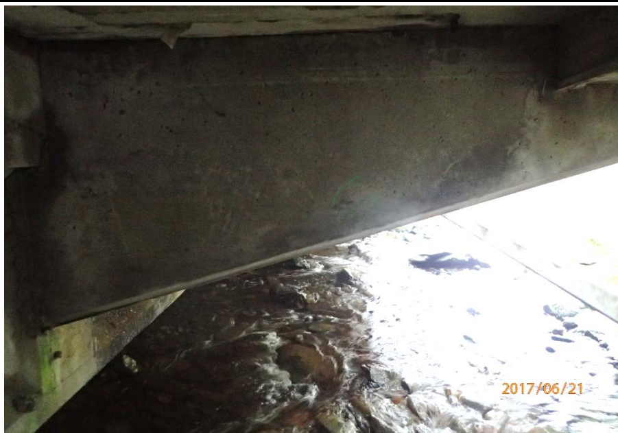
Bridge No. 0725 Br. Name Hoadley Creek Date 06/21/17 Inspector Manning / McRae Frame 35 US cantilever support side 6 overview
