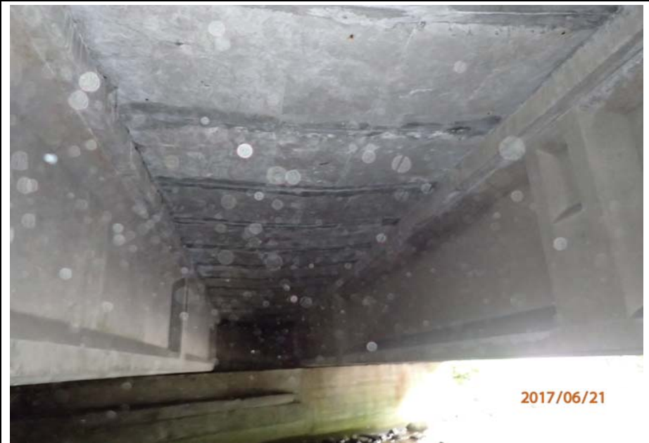
Bridge No. 0725 Br. Name Hoadley Creek Date 06/21/17 Inspector Manning / McRae Frame 8 Typical bay
