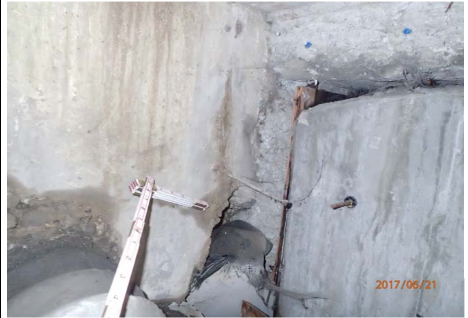
Bridge No. 0725 Br. Name Hoadley Creek Date 06/21/17 Inspector Manning / McRae Frame 18 FE US abutment spalls with exposed rebar
