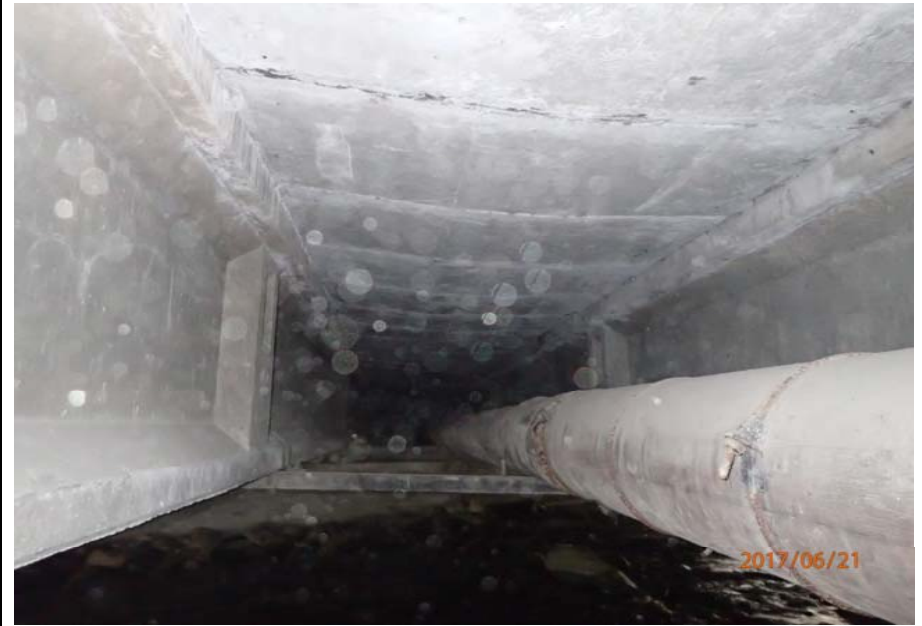
Bridge No. 0725 Br. Name Hoadley Creek Date 06/21/17 Inspector Manning / McRae Frame 46 Mid-span utility
