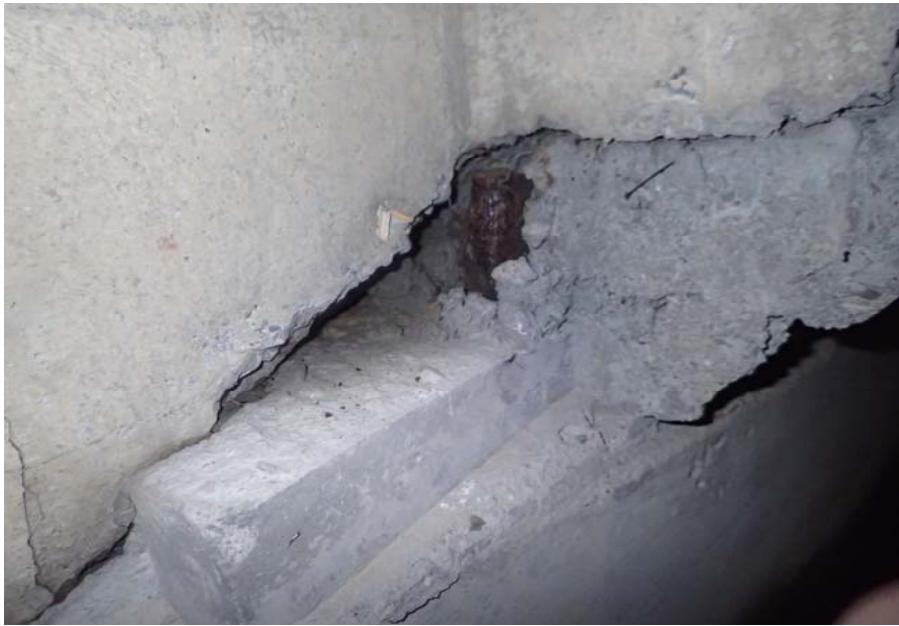
Bridge No. 0725 Br. Name Hoadley Creek Date 06/21/17 Inspector Manning / McRae Frame 45 NE abutment, 2nd bay from DS, void 22" deep x 9"
