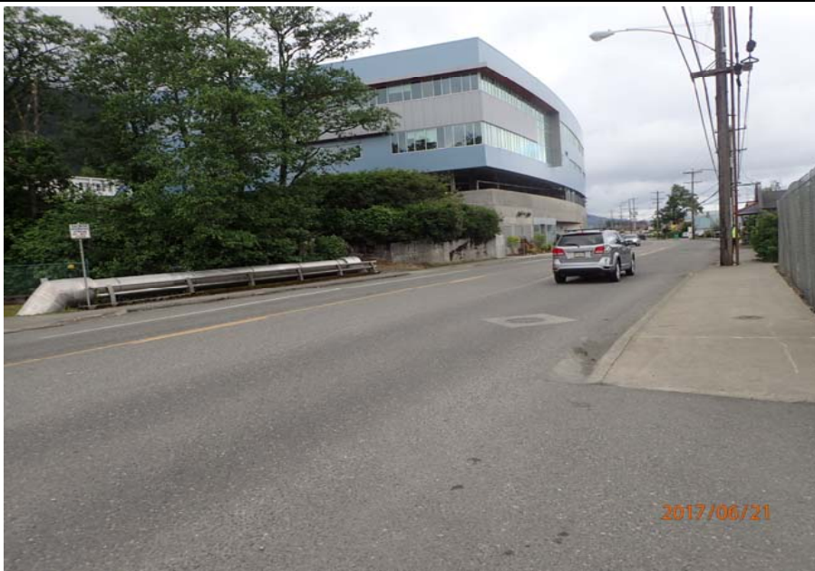
Bridge No. 0725 Br. Name Hoadley Creek Date 06/21/17 Inspector Manning / McRae Frame 7 Wearing surface condition
