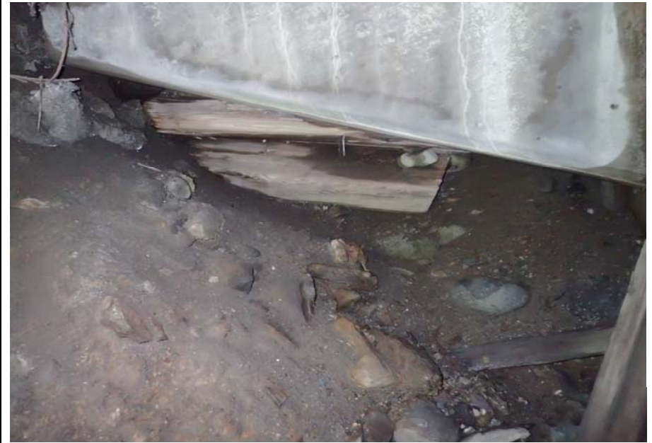
Bridge No. 0725 Br. Name Hoadley Creek Date 06/21/17 Inspector Manning / McRae Frame 38 FE DS material spilling around wingwall
