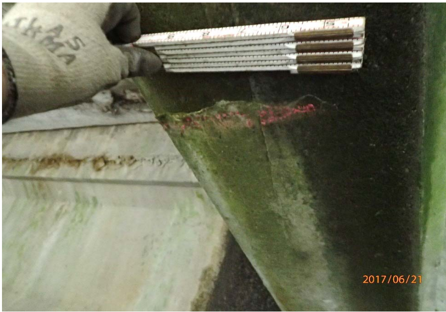
Bridge No. 0725 Br. Name Hoadley Creek Date 06/21/17 Inspector Manning / McRae Frame 29 Cracks bottom cantilever support #2 (RT/LT faces are sides 3 & 4)
