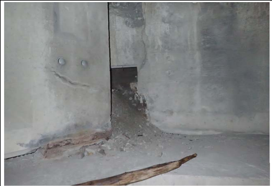
Bridge No. 0725 Br. Name Hoadley Creek Date 06/21/17 Inspector Manning / McRae Frame 44 Wet soil spilling through backwall and resting against girder ends
