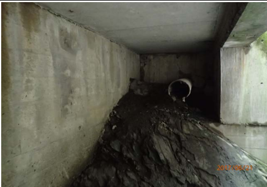
Bridge No. 0725 Br. Name Hoadley Creek Date 06/21/17 Inspector Manning / McRae Frame 15 FE US abutment
