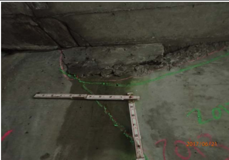
Bridge No. 0725 Br. Name Hoadley Creek Date 06/21/17 Inspector Manning / McRae Frame 31 US cantilever support side 4 crack and spall
