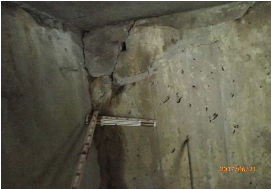
Bridge No. 0725 Br. Name Hoadley Creek Date 06/21/17 Inspector Manning / McRae Frame 17 FE US abutment spalls with exposed rebar
