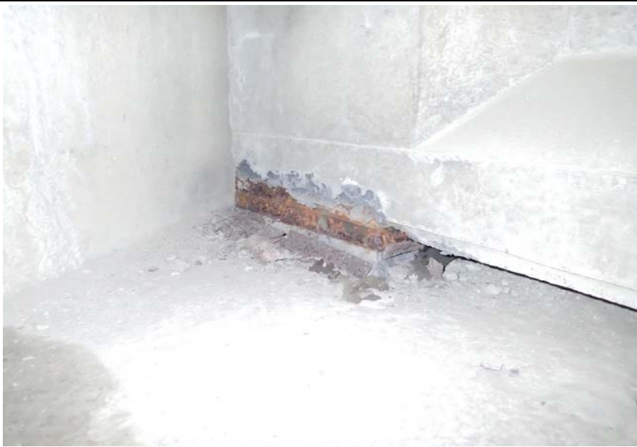
Bridge No. 0725 Br. Name Hoadley Creek Date 06/21/17 Inspector Manning / McRae Frame 43 Metal bearing surface rust and minor section loss typical
