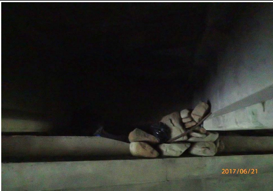
Bridge No. 0725 Br. Name Hoadley Creek Date 06/21/17 Inspector Manning / McRae Frame 47 Rocks on FE abutment
