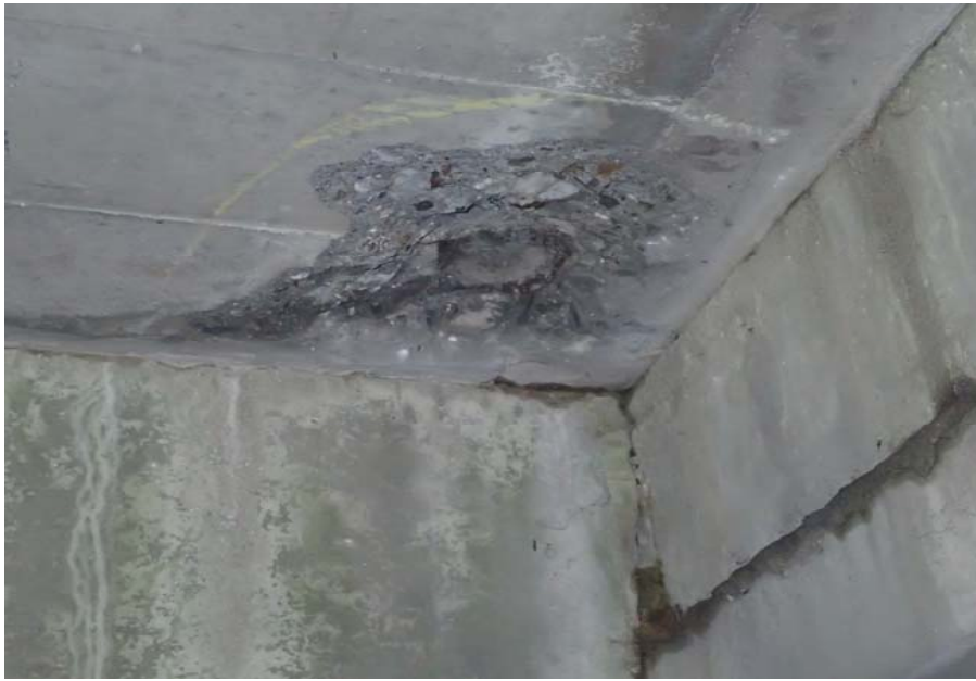
Bridge No. 0725 Br. Name Hoadley Creek Date 06/21/17 Inspector Manning / McRae Frame 41 FE DS 1 SF cantilever deck spall with exposed rebar
