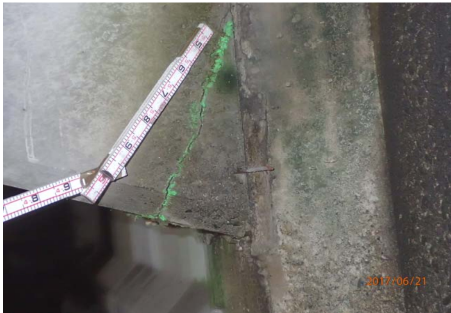
Bridge No. 0725 Br. Name Hoadley Creek Date 06/21/17 Inspector Manning / McRae Frame 33 US cantilever support side 5 crack
