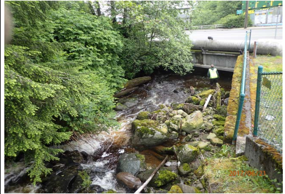
Bridge No. 0725 Br. Name Hoadley Creek Date 06/21/17 Inspector Manning / McRae Frame 6 Elevation Looking DS
