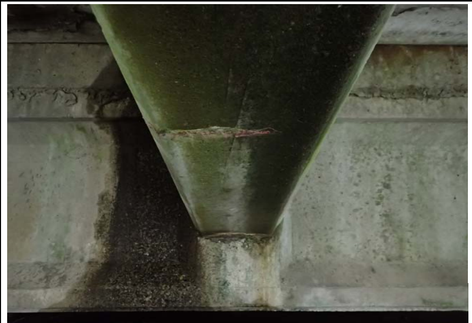
Bridge No. 0725 Br. Name Hoadley Creek Date 06/21/17 Inspector Manning / McRae Frame 36 US cantilever supports cracked on underside, typical
