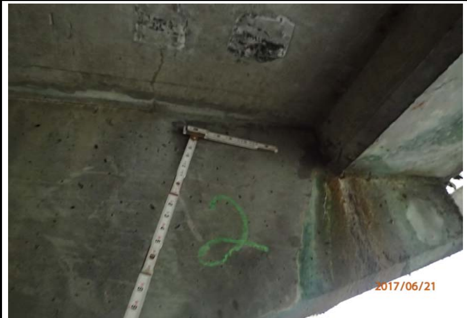
Bridge No. 0725 Br. Name Hoadley Creek Date 06/21/17 Inspector Manning / McRae Frame 24 US cantilever support side 2 rust stain, cracks
