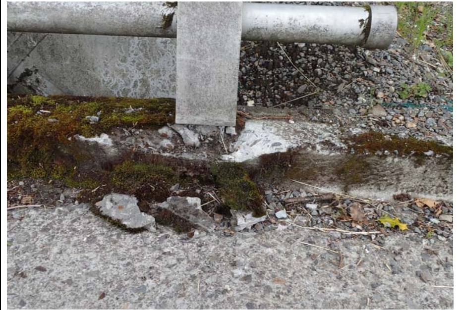
Bridge No. 0725 Br. Name Hoadley Creek Date 06/21/17 Inspector Manning / McRae Frame 14 Damage and spall at NE US rail post
