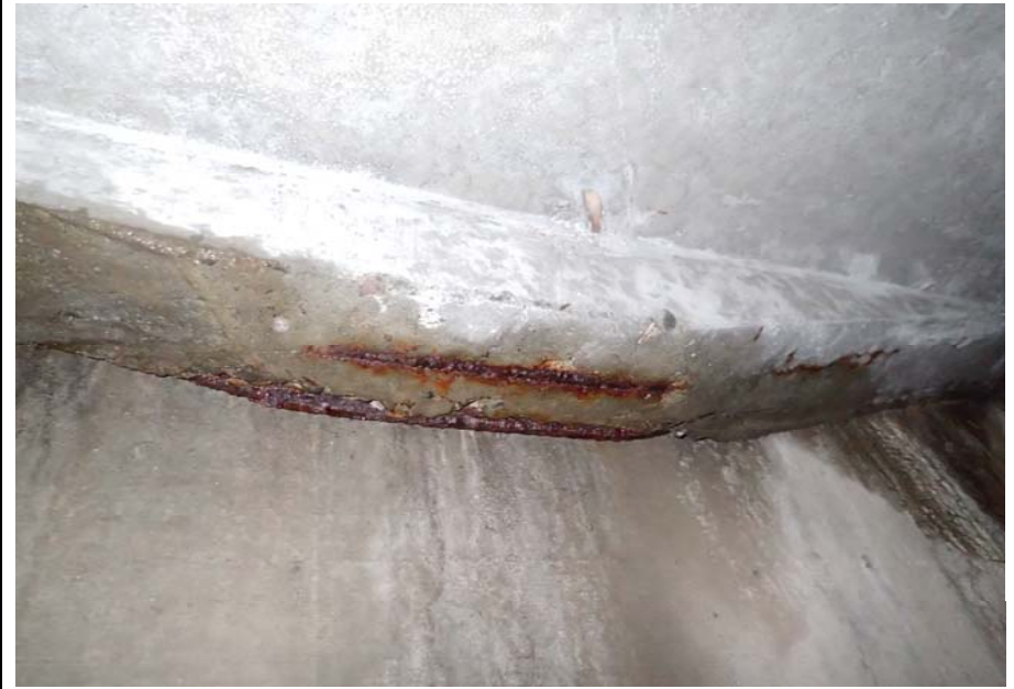
Bridge No. 0725 Br. Name Hoadley Creek Date 06/21/17 Inspector Manning / McRae Frame 42 NE abutment, 2nd bay from DS, exposed rebar
