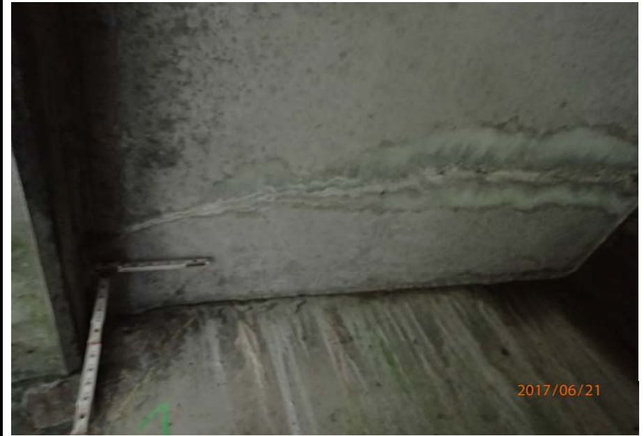
Bridge No. 0725 Br. Name Hoadley Creek Date 06/21/17 Inspector Manning / McRae Frame 22 US cantilever support side 1 crack in soffit
