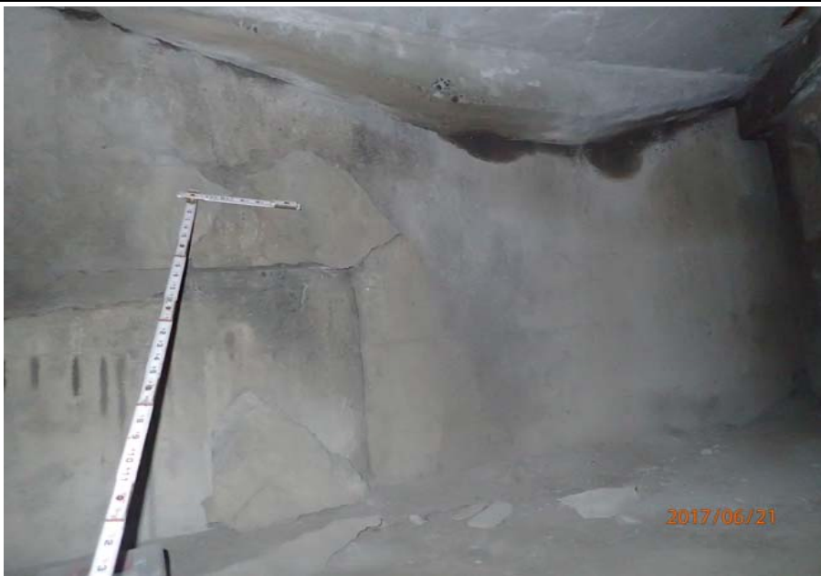
Bridge No. 0725 Br. Name Hoadley Creek Date 06/21/17 Inspector Manning / McRae Frame 39 FE backwall cracks, 3rd bay from US
