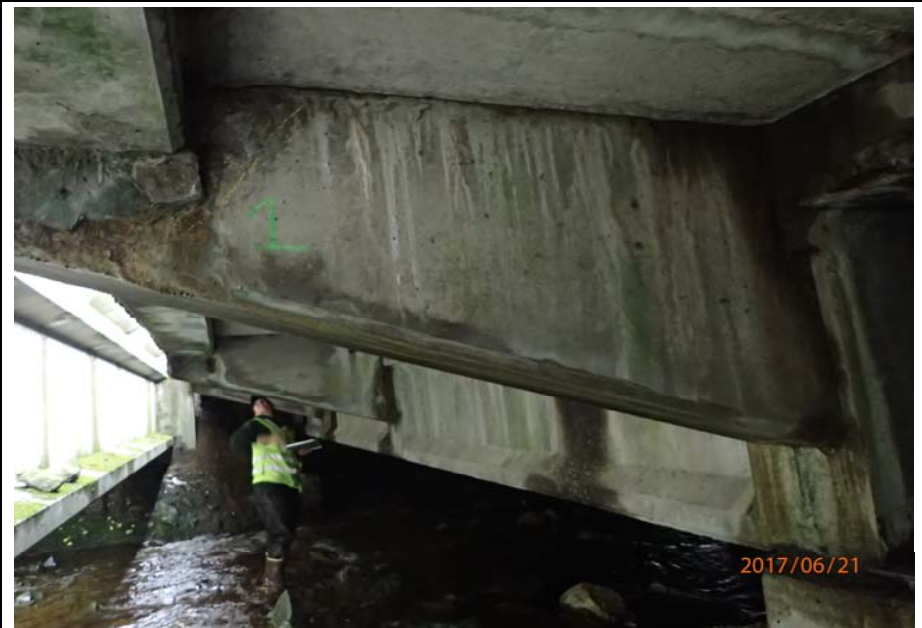
Bridge No. 0725 Br. Name Hoadley Creek Date 06/21/17 Inspector Manning / McRae Frame 20 US cantilever support side 1 overview
