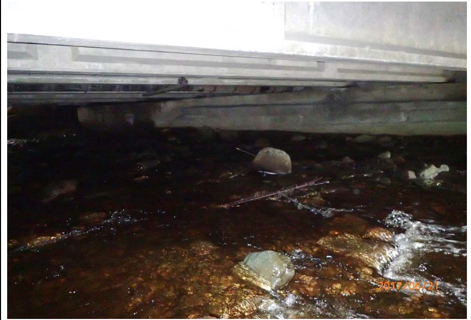
Bridge No. 0725 Br. Name Hoadley Creek Date 06/21/17 Inspector Manning / McRae Frame 10 NE abutment (US)
