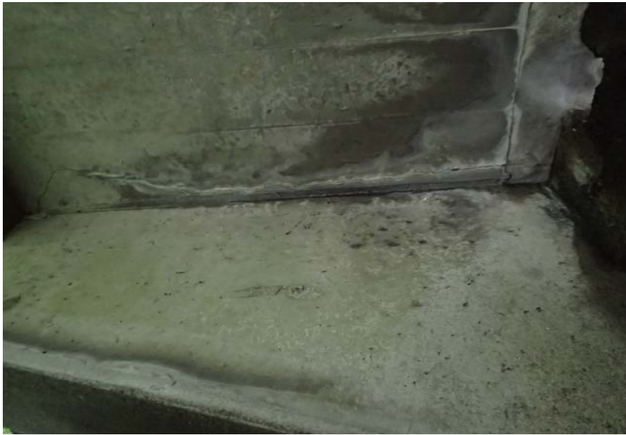
Bridge No. 0725 Br. Name Hoadley Creek Date 06/21/17 Inspector Manning / McRae Frame 37 Crack full width of cantilever support
