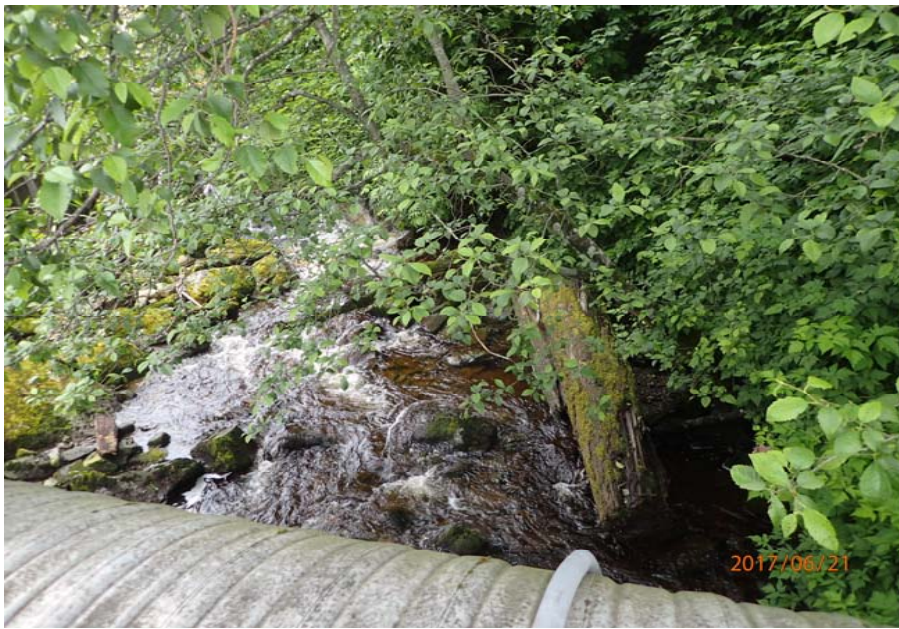
Bridge No. 0725 Br. Name Hoadley Creek Date 06/21/17 Inspector Manning / McRae Frame 3 Looking US
