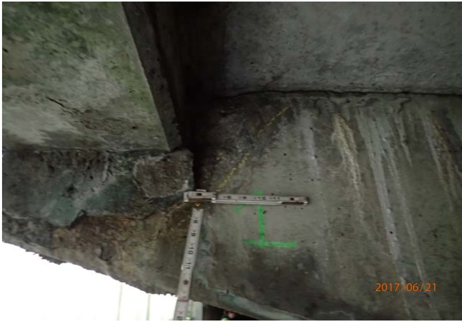
Bridge No. 0725 Br. Name Hoadley Creek Date 06/21/17 Inspector Manning / McRae Frame 21 US cantilever support side 1 spall
