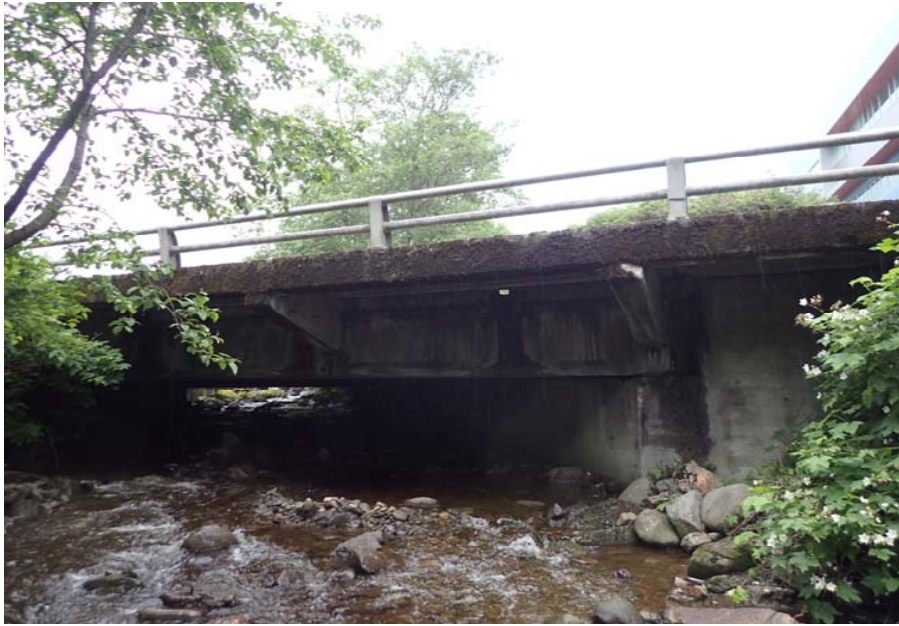
Bridge No. 0725 Br. Name Hoadley Creek Date 06/21/17 Inspector Manning / McRae Frame 5 Elevation Looking US
