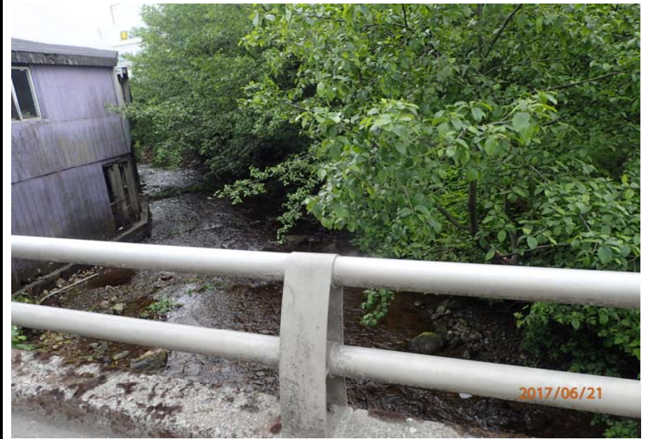
Bridge No. 0725 Br. Name Hoadley Creek Date 06/21/17 Inspector Manning / McRae Frame 4 Looking DS
