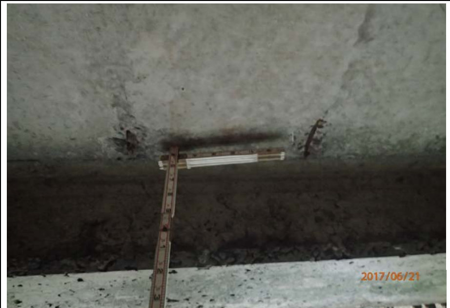
Bridge No. 0725 Br. Name Hoadley Creek Date 06/21/17 Inspector Manning / McRae Frame 16 FE US abutment spalls with exposed rebar
