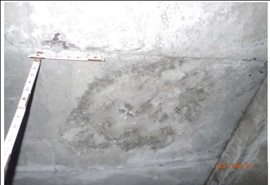
Bridge No. 0725 Br. Name Hoadley Creek Date 06/21/17 Inspector Manning / McRae Frame 40 Spall near FE backwall, 3rd bay from US
