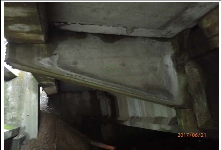
Bridge No. 0725 Br. Name Hoadley Creek Date 06/21/17 Inspector Manning / McRae Frame 32 US cantilever support side 5 overview
