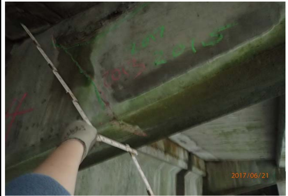
Bridge No. 0725 Br. Name Hoadley Creek Date 06/21/17 Inspector Manning / McRae Frame 30 US cantilever support side 4 crack
