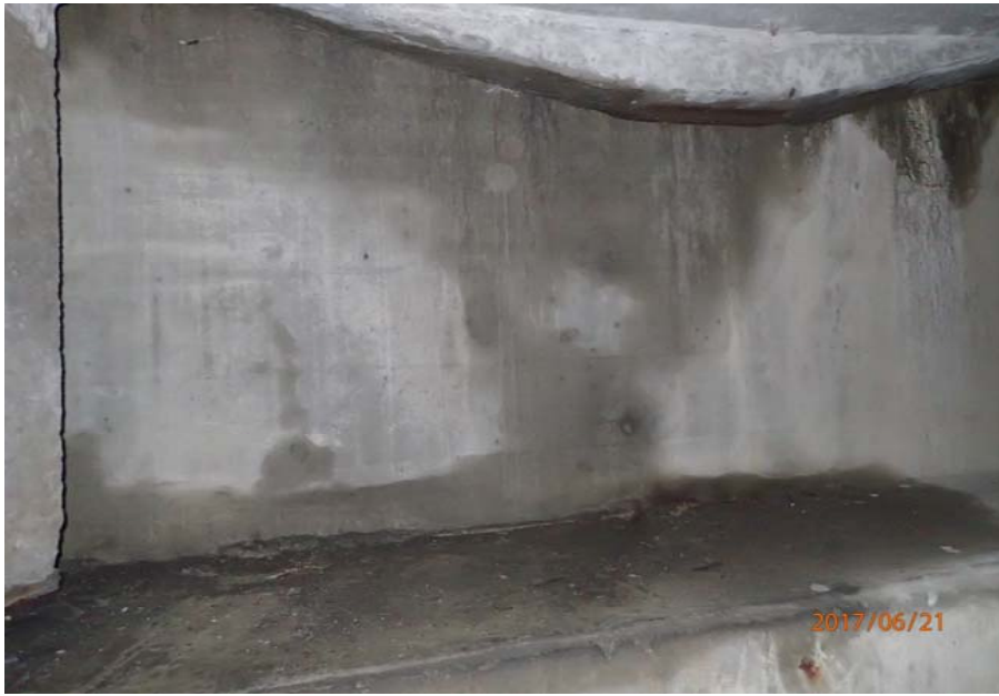
Bridge No. 0725 Br. Name Hoadley Creek Date 06/21/17 Inspector Manning / McRae Frame 9 Backwall typical
