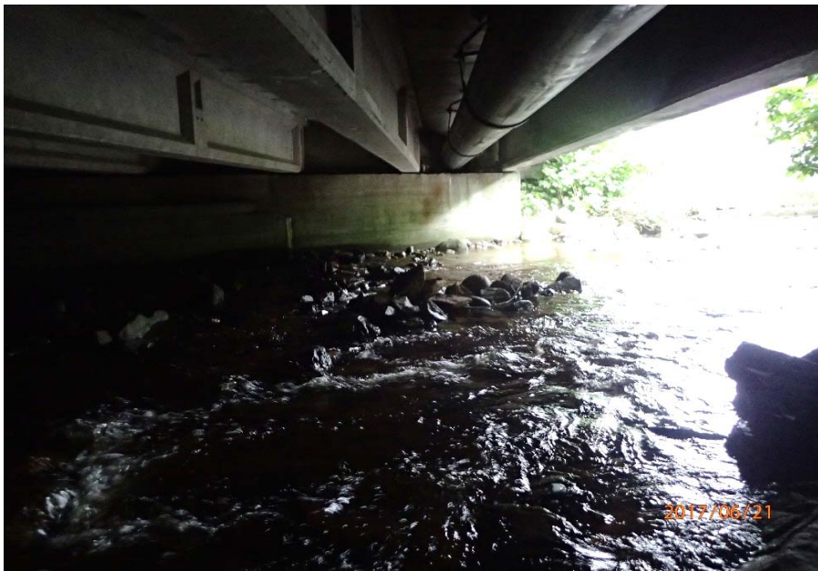
Bridge No. 0725 Br. Name Hoadley Creek Date 06/21/17 Inspector Manning / McRae Frame 11 NE abutment (DS)
