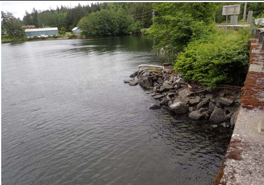
Bridge No. 0253 Br. Name Herring Cove Date 06/25/17 Inspector Manning / Escamilla Frame 7 Looking RT NE
