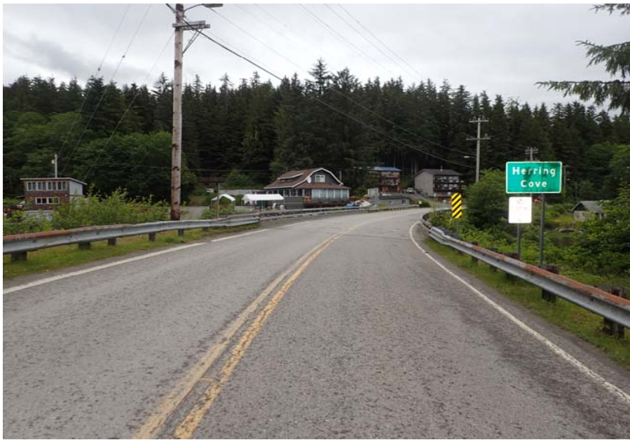
Bridge No. 0253 Br. Name Herring Cove Date 06/25/17 Inspector Manning / Escamilla Frame 1 Ahead at bridge
