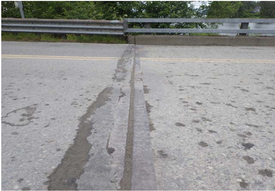
Bridge No. 0253 Br. Name Herring Cove Date 06/25/17 Inspector Manning / Escamilla Frame 17 FE joint
