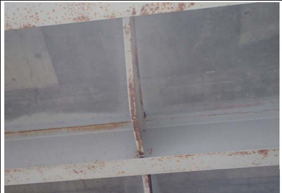
Bridge No. 0253 Br. Name Herring Cove Date 06/25/17 Inspector Manning / Escamilla Frame 24 Span 2 Bay 3 diaphragm near Pier 2 bowed
