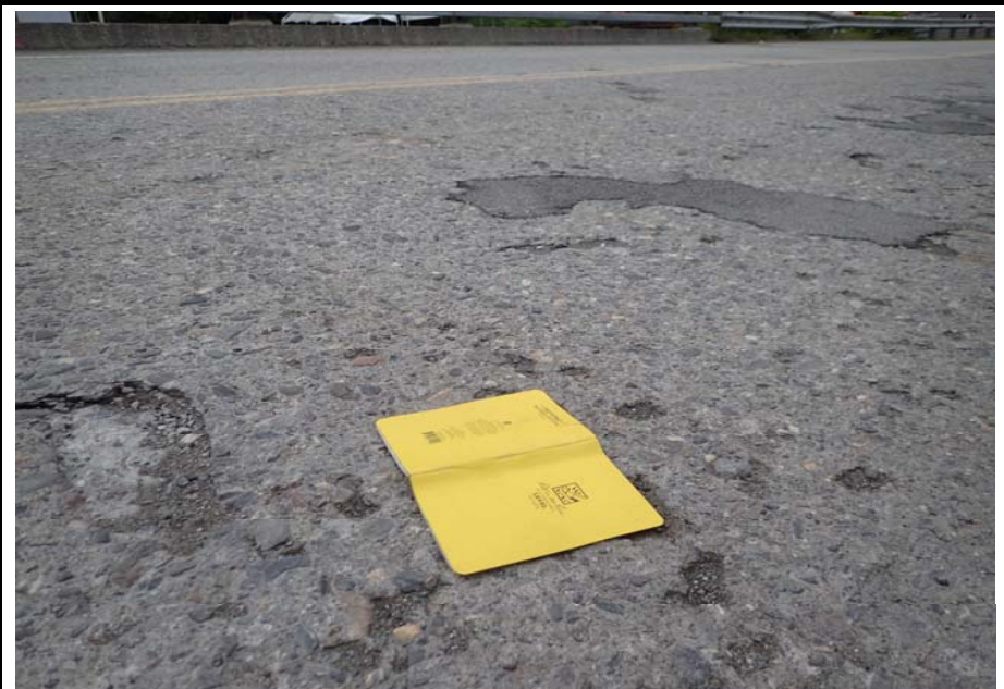
Bridge No. 0253 Br. Name Herring Cove Date 06/25/17 Inspector Manning / Escamilla Frame 12 Deck typical
