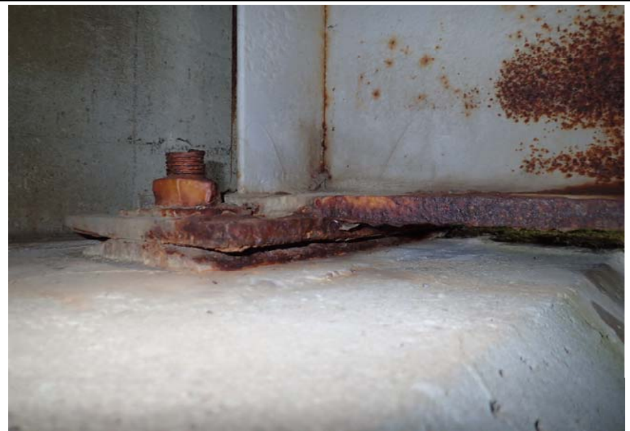
Bridge No. 0253 Br. Name Herring Cove Date 06/25/17 Inspector Manning / Escamilla Frame 20 NE bearing typical
