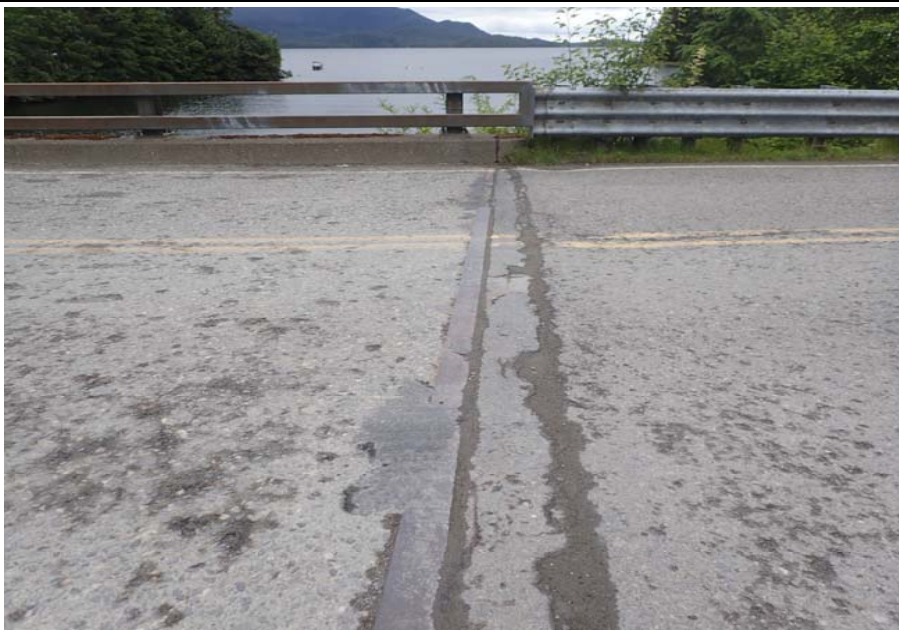
Bridge No. 0253 Br. Name Herring Cove Date 06/25/17 Inspector Manning / Escamilla Frame 15 NE joint
