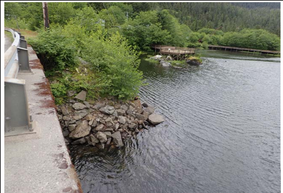
Bridge No. 0253 Br. Name Herring Cove Date 06/25/17 Inspector Manning / Escamilla Frame 8 Looking LT NE
