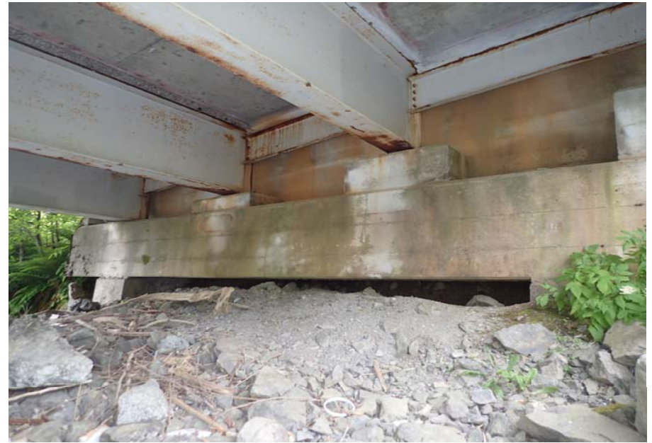
Bridge No. 0253 Br. Name Herring Cove Date 06/25/17 Inspector Manning / Escamilla Frame 18 NE abutment up to 3' undermined
