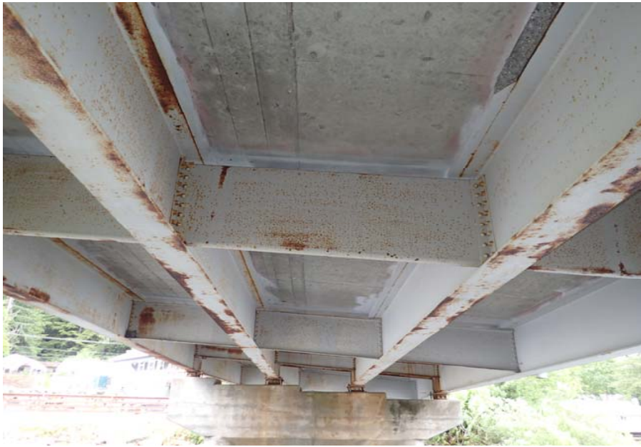
Bridge No. 0253 Br. Name Herring Cove Date 06/25/17 Inspector Manning / Escamilla Frame 21 Underside of deck typical
