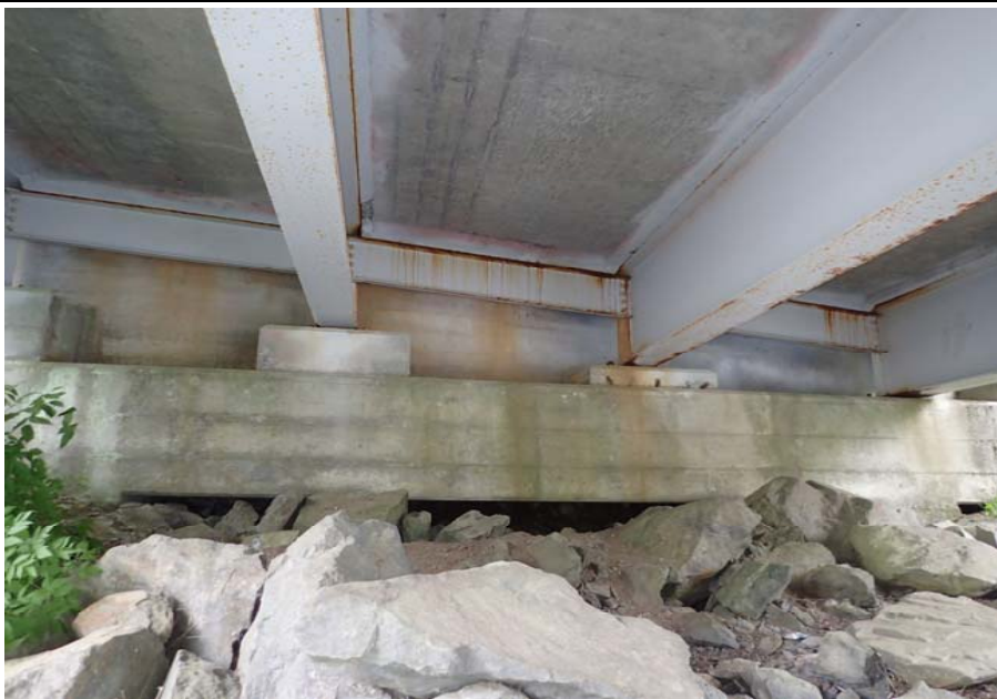
Bridge No. 0253 Br. Name Herring Cove Date 06/25/17 Inspector Manning / Escamilla Frame 19 FE abutment
