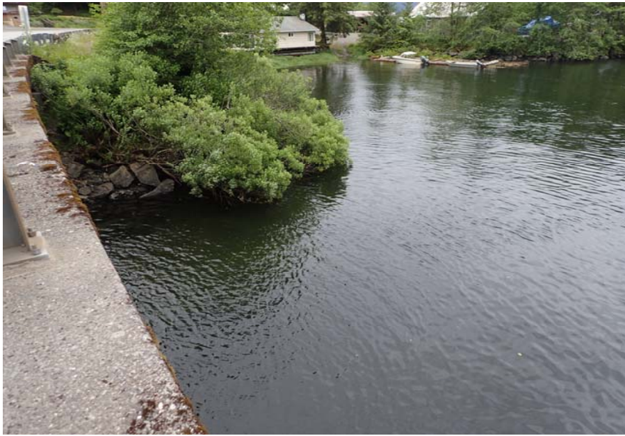
Bridge No. 0253 Br. Name Herring Cove Date 06/25/17 Inspector Manning / Escamilla Frame 5 Looking RT FE
