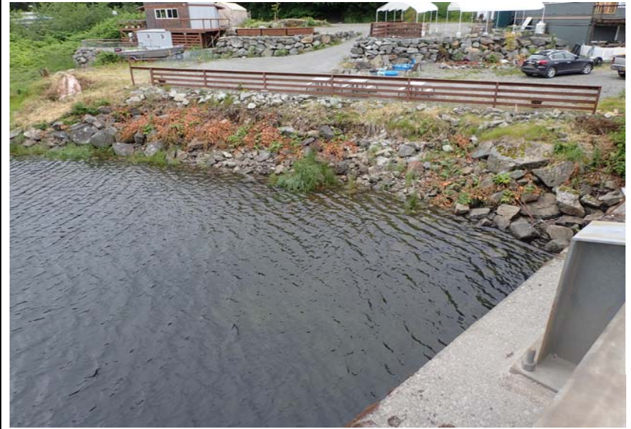
Bridge No. 0253 Br. Name Herring Cove Date 06/25/17 Inspector Manning / Escamilla Frame 10 Looking LT FE
