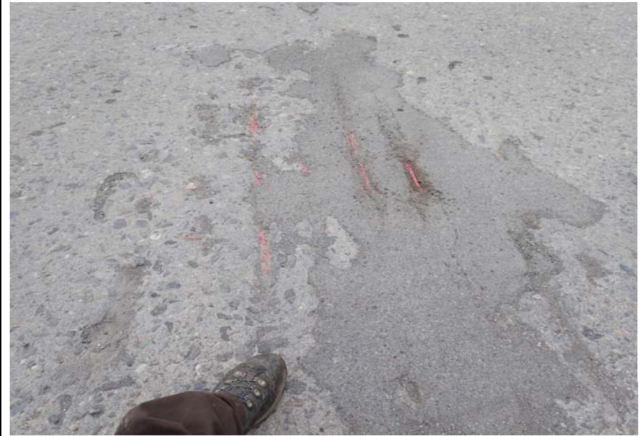
Bridge No. 0253 Br. Name Herring Cove Date 06/25/17 Inspector Manning / Escamilla Frame 14 Exposed deck bar
