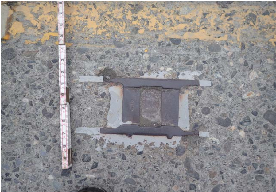
Bridge No. 0253 Br. Name Herring Cove Date 06/25/17 Inspector Manning / Escamilla Frame 13 Deck embedded hardware
