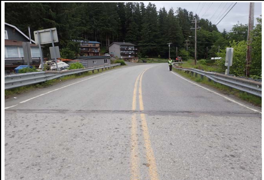
Bridge No. 0253 Br. Name Herring Cove Date 06/25/17 Inspector Manning / Escamilla Frame 4 FE looking away from bridge
