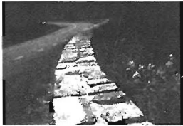
Top: crash tested and approved concrete-core barrier wall under construction. Bottom: completed concrete-core barrier wall.
