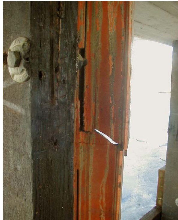
Figure 3. Fractured Pile from Slana River Bridge Earthquake Damage
