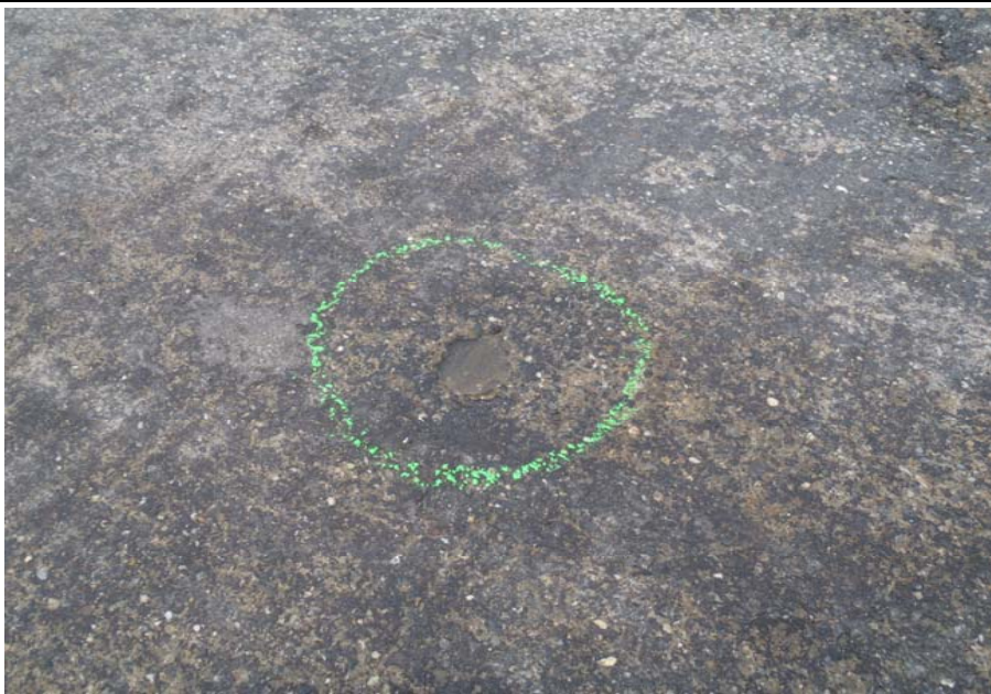
Bridge No. 1141 Br. Name Antler Creek Date 07/16/17 Inspector Murray / Knapp Frame 11 FE Approach Slab
