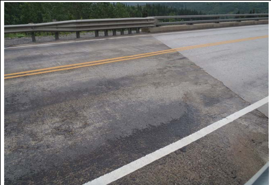
Bridge No. 1141 Br. Name Antler Creek Date 07/16/17 Inspector Murray / Knapp Frame 8 FE Approach Slab
