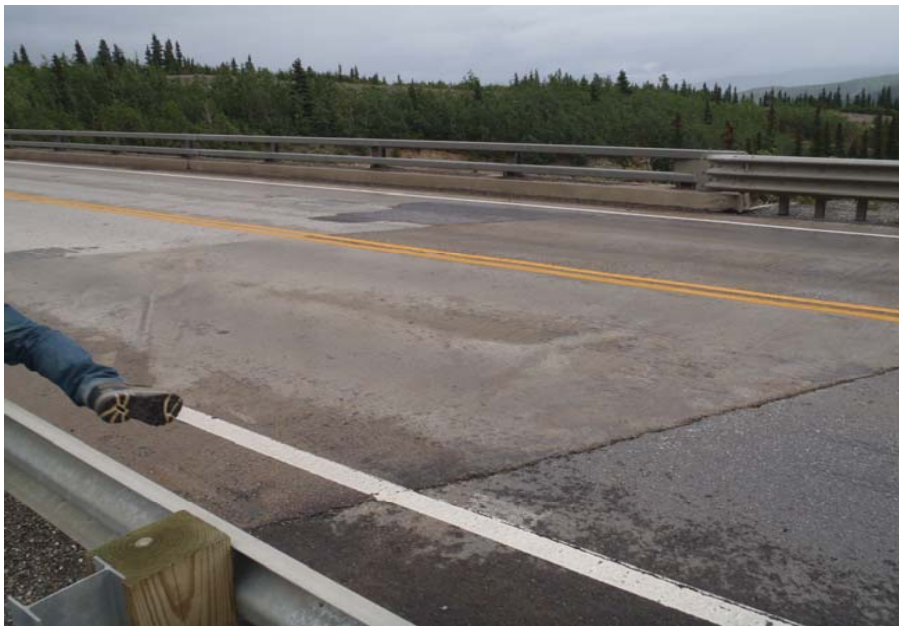
Bridge No. 1141 Br. Name Antler Creek Date 07/16/17 Inspector Murray / Knapp Frame 1 NE Approach Slab
