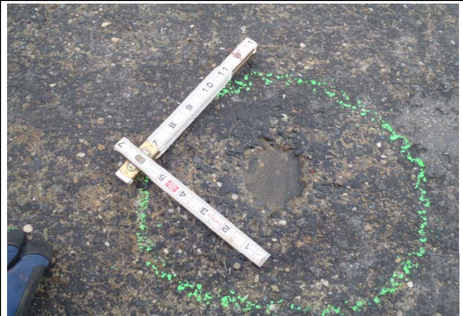
Bridge No. 1141 Br. Name Antler Creek Date 07/16/17 Inspector Murray / Knapp Frame 12 FE Approach Slab
