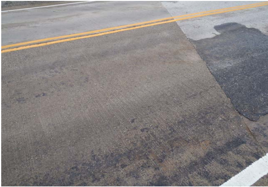
Bridge No. 1141 Br. Name Antler Creek Date 07/16/17 Inspector Murray / Knapp Frame 5 NE Approach Slab
