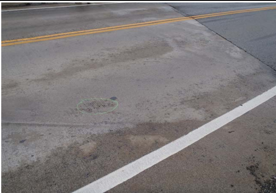
Bridge No. 1141 Br. Name Antler Creek Date 07/16/17 Inspector Murray / Knapp Frame 3 NE Approach Slab
