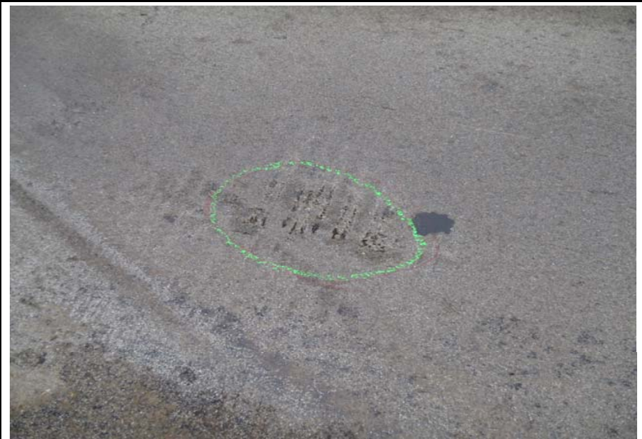
Bridge No. 1141 Br. Name Antler Creek Date 07/16/17 Inspector Murray / Knapp Frame 4 NE Approach Slab
