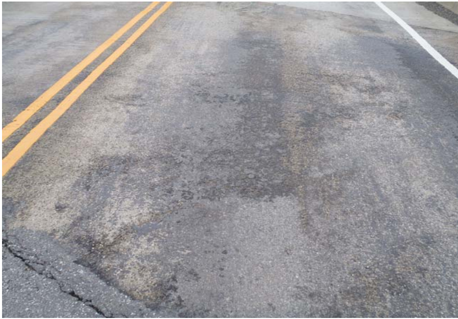
Bridge No. 1141 Br. Name Antler Creek Date 07/16/17 Inspector Murray / Knapp Frame 9 FE Approach Slab
