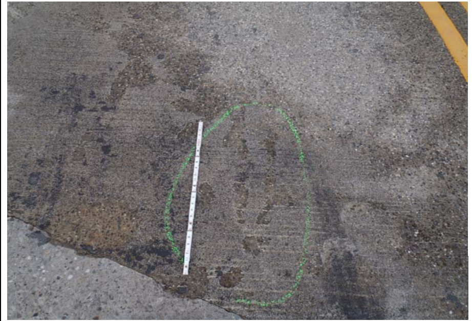
Bridge No. 1141 Br. Name Antler Creek Date 07/16/17 Inspector Murray / Knapp Frame 10 FE Approach Slab
