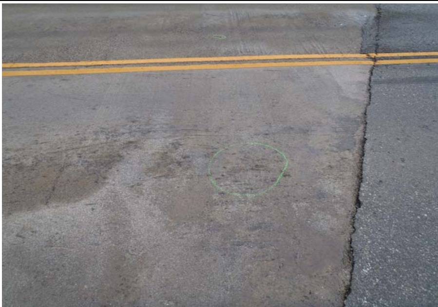
Bridge No. 1141 Br. Name Antler Creek Date 07/16/17 Inspector Murray / Knapp Frame 7 NE Approach Slab
