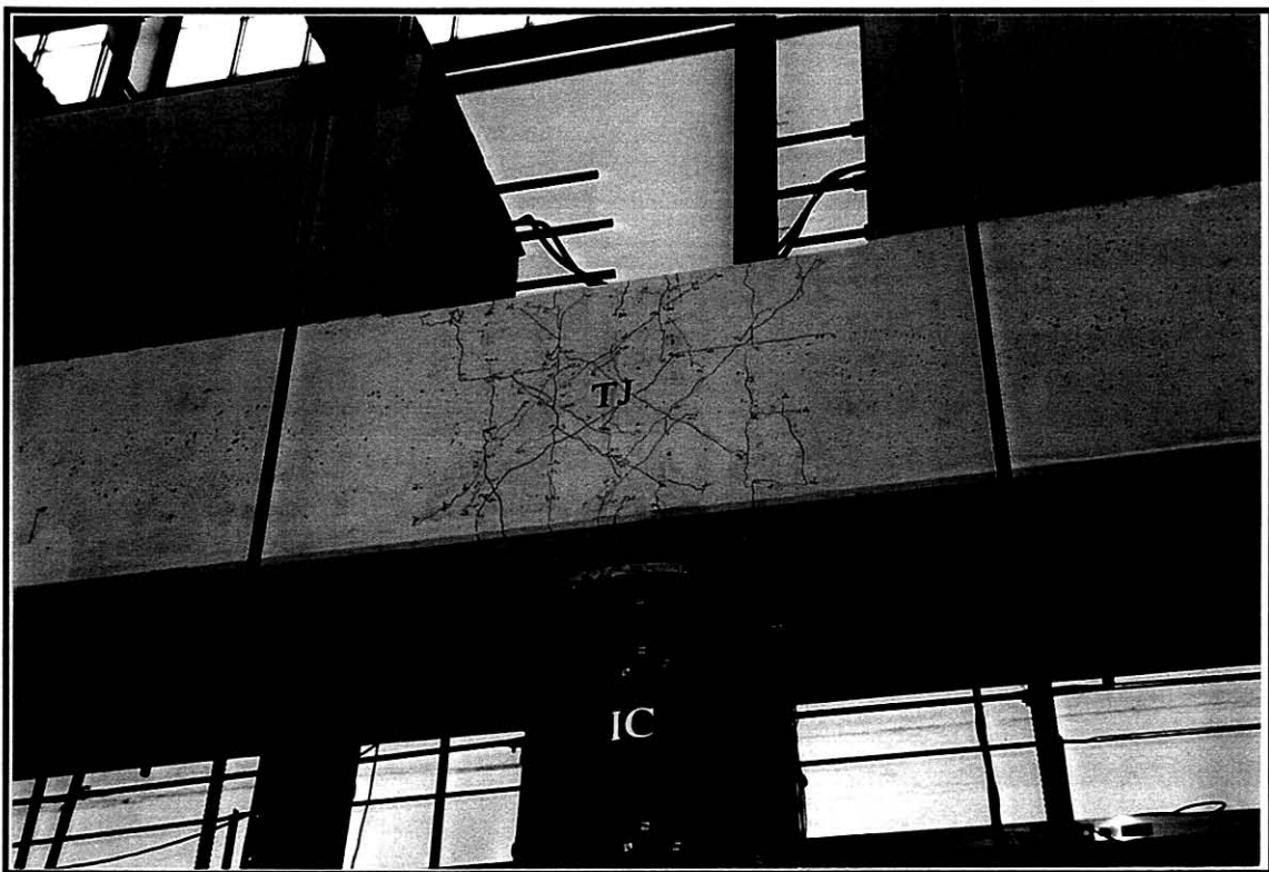
Fig.7-21 Joint Region Cracking at \mu_d = \pm 6x3 - Interior Joint TJ
