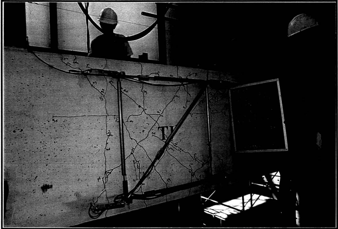
Fig.7-18 Joint Region Cracking at \mu_d = \pm 4x3 - Interior Joint TJ
