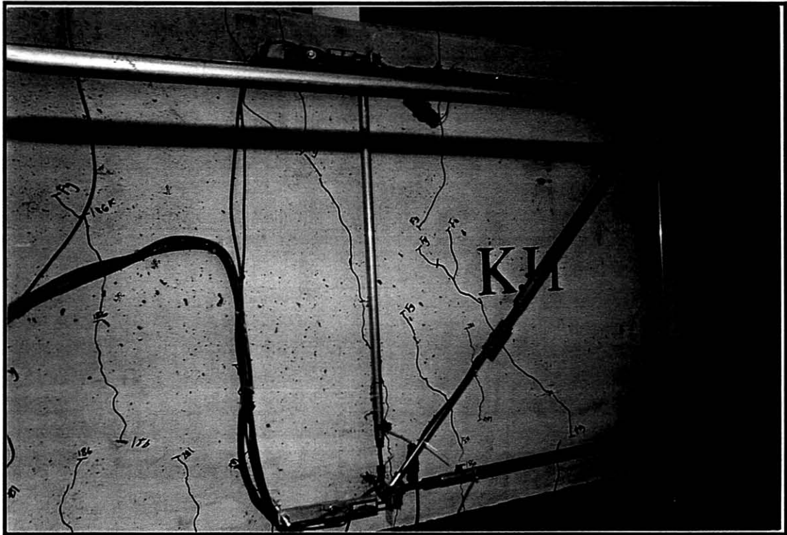
Fig.7-8 Joint Shear Cracking at \pm V_y - Exterior Joint KJI
