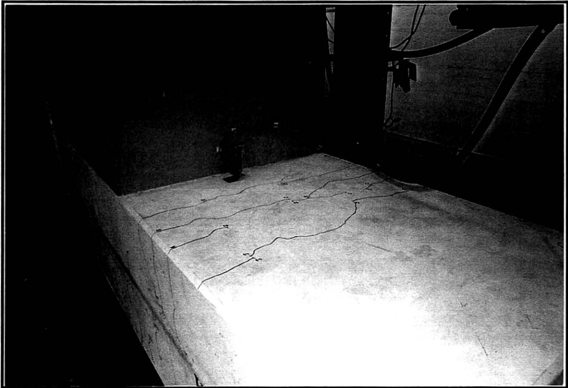
Fig.7-11 Cap Beam Flexural Cracking at \pm V_y - Exterior Joint KJ2
