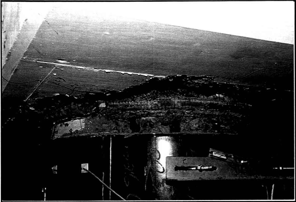
Fig.7-32 Extent of Spalling - Typical at Top of All Three Columns
