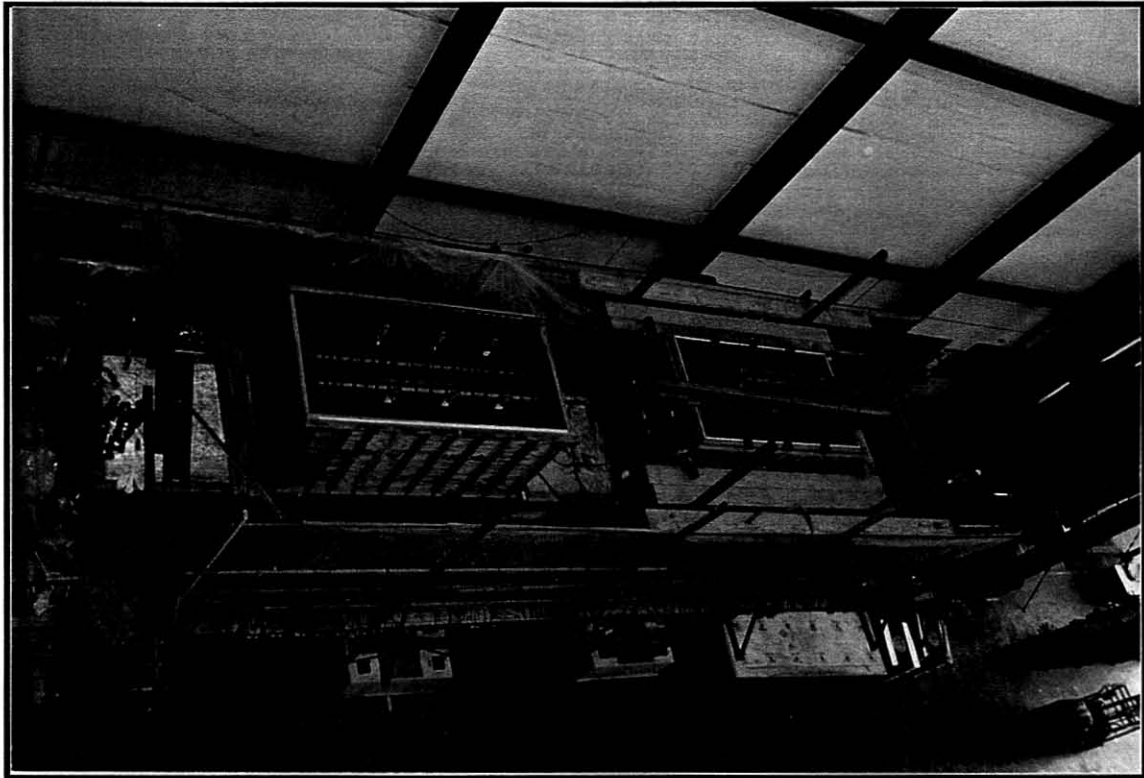
Fig.5-13 Construction of the Load Transfer Blocks After Casting of the Cap Beam
