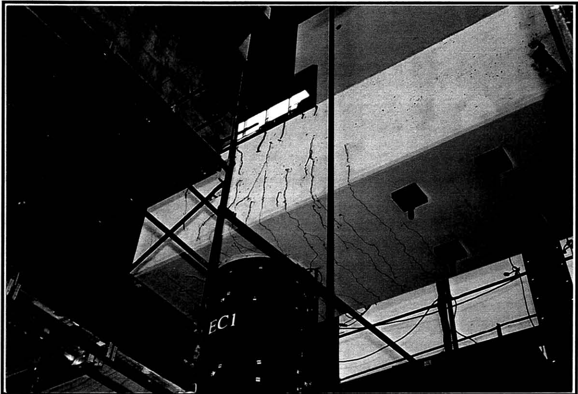
Fig.7-15 Cap Beam Cracking at \mu_d = \pm 1x1 - Exterior Joint KJ1
