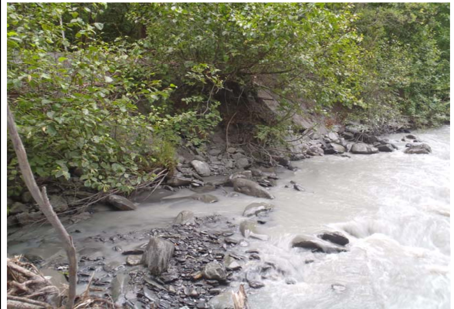
Bridge No. 0607 Br. Name Victor Creek Date 08/09/17 Inspector Murray / Murph Frame 8 Looking FE US
