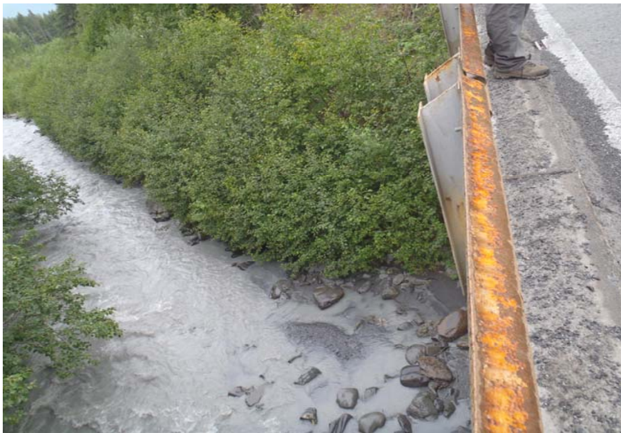
Bridge No. 0607 Br. Name Victor Creek Date 08/09/17 Inspector Murray / Murph Frame 7 Looking FE DS
