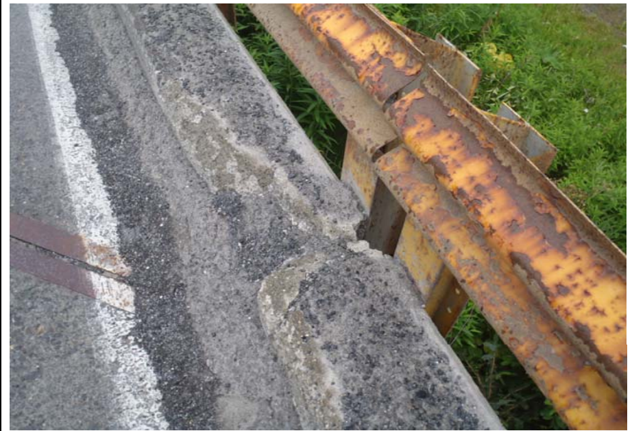
Bridge No. 0607 Br. Name Victor Creek Date 08/09/17 Inspector Murray / Murph Frame 14 DS NE rail spall
