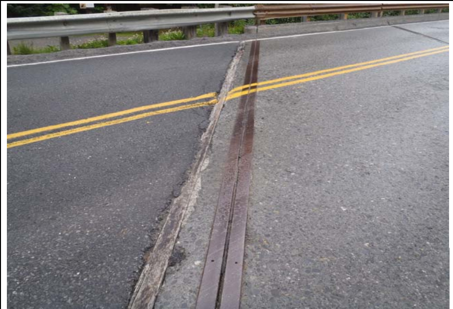
Bridge No. 0607 Br. Name Victor Creek Date 08/09/17 Inspector Murray / Murph Frame 20 DS FE expansion joint
