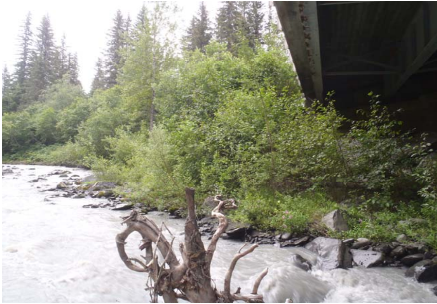
Bridge No. 0607 Br. Name Victor Creek Date 08/09/17 Inspector Murray / Murph Frame 5 Looking NE US
