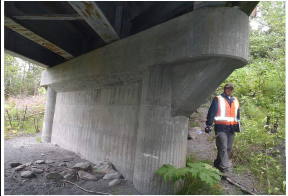
Bridge No. 0607 Br. Name Victor Creek Date 08/09/17 Inspector Murray / Murph Frame 34 NE face pier 4
