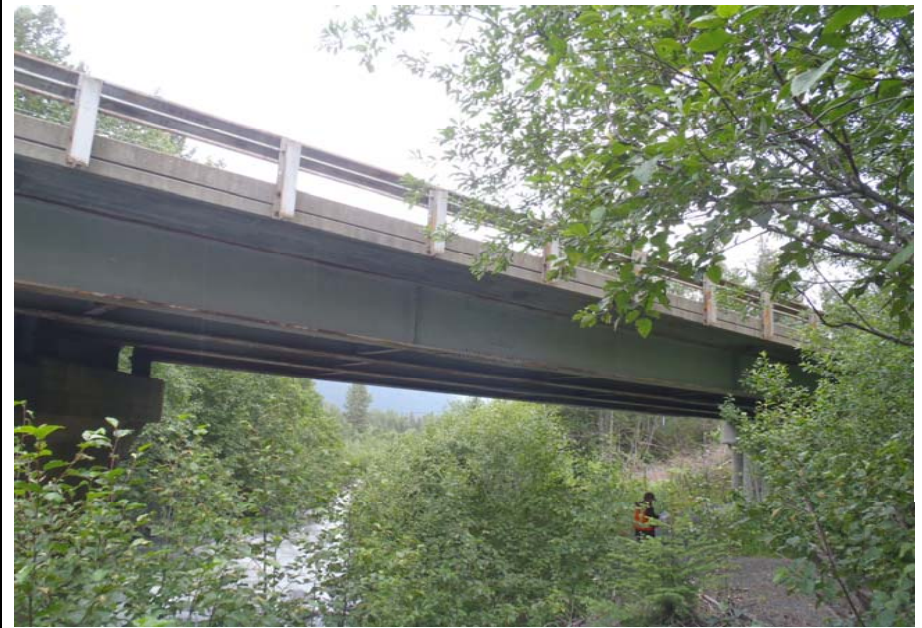
Bridge No. 0607 Br. Name Victor Creek Date 08/09/17 Inspector Murray / Murph Frame 10 US FE elevation
