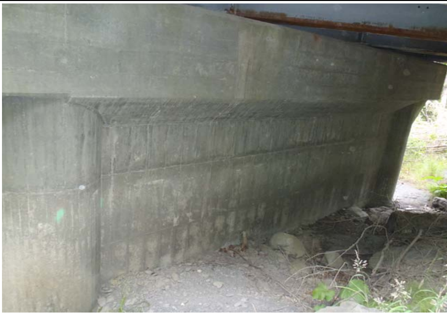
Bridge No. 0607 Br. Name Victor Creek Date 08/09/17 Inspector Murray / Murph Frame 35 FE face pier 4
