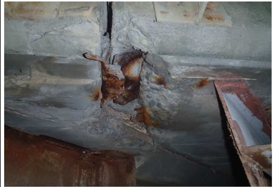
Bridge No. 0607 Br. Name Victor Creek Date 08/09/17 Inspector Murray / Murph Frame 26 US NE spalling along expansion joint
