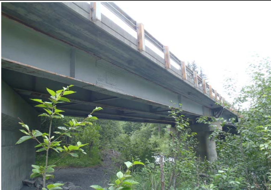
Bridge No. 0607 Br. Name Victor Creek Date 08/09/17 Inspector Murray / Murph Frame 11 DS elevation
