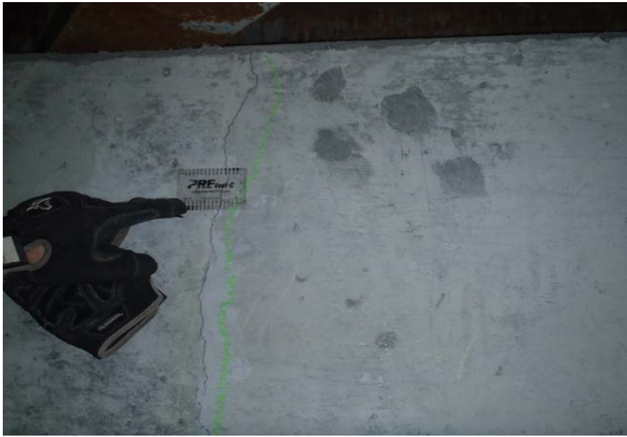
Bridge No. 0607 Br. Name Victor Creek Date 08/09/17 Inspector Murray / Murph Frame 29 NE face Pier 2 crack 10' from DS
