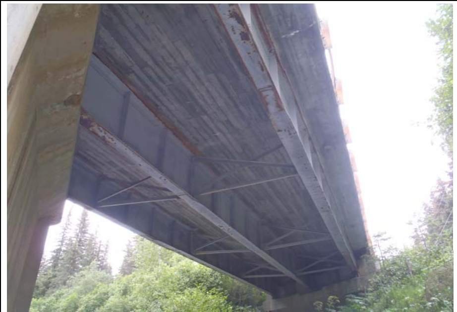
Bridge No. 0607 Br. Name Victor Creek Date 08/09/17 Inspector Murray / Murph Frame 24 NE underside, typ.
