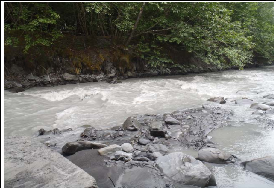
Bridge No. 0607 Br. Name Victor Creek Date 08/09/17 Inspector Murray / Murph Frame 12 DS NE undercutting along bank
