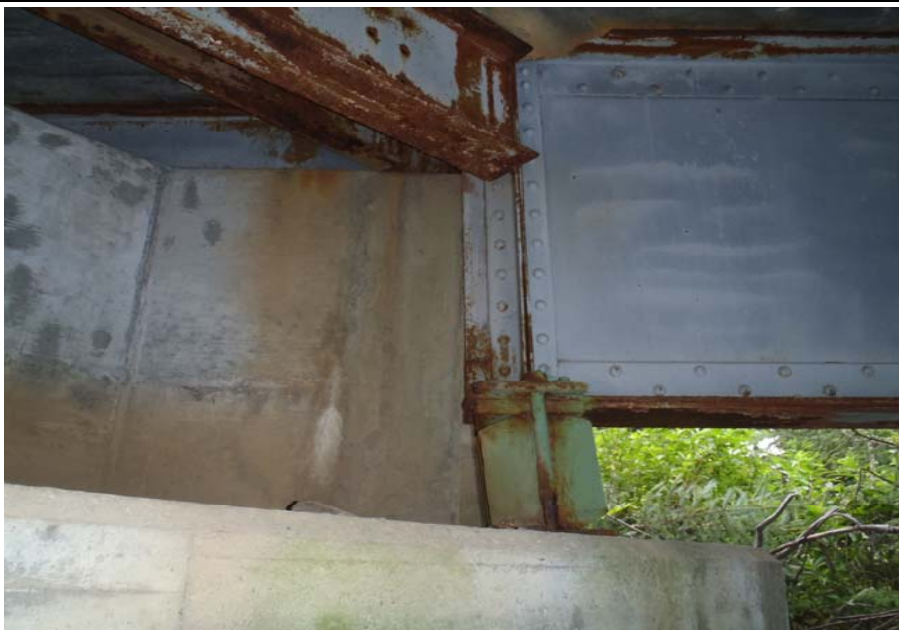
Bridge No. 0607 Br. Name Victor Creek Date 08/09/17 Inspector Murray / Murph Frame 23 DS pier 2 concrete and girder contact
