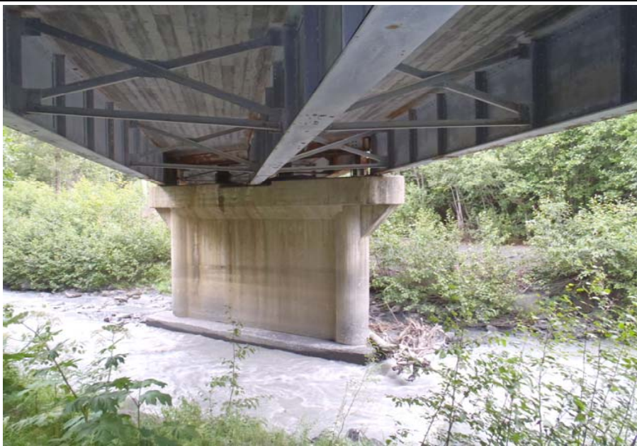
Bridge No. 0607 Br. Name Victor Creek Date 08/09/17 Inspector Murray / Murph Frame 31 NE face Pier 3
