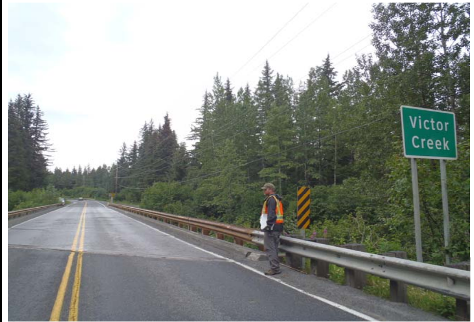
Bridge No. 0607 Br. Name Victor Creek Date 08/09/17 Inspector Murray / Murph Frame 2 Back at bridge
