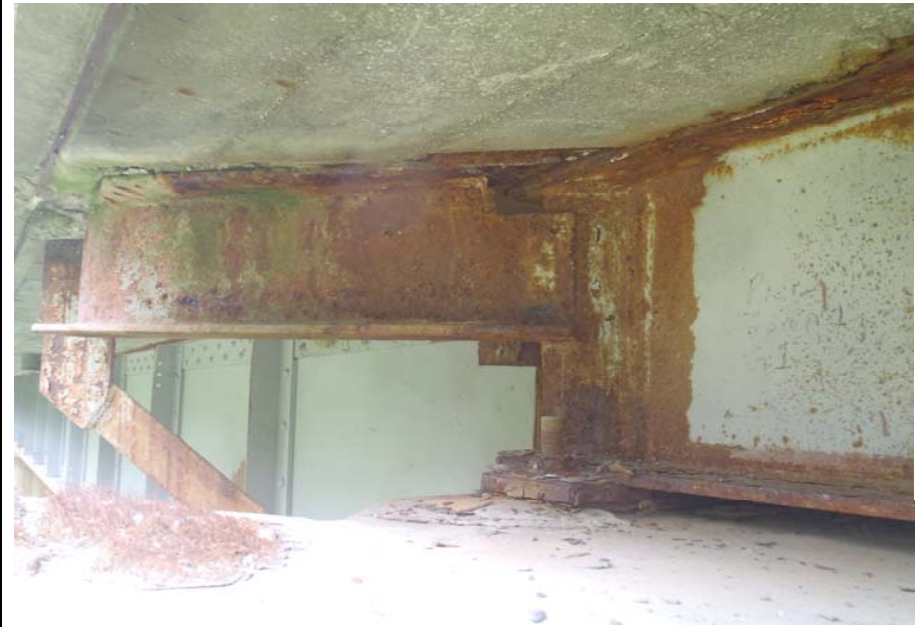
Bridge No. 0607 Br. Name Victor Creek Date 08/09/17 Inspector Murray / Murph Frame 22 Bearing, typ.
