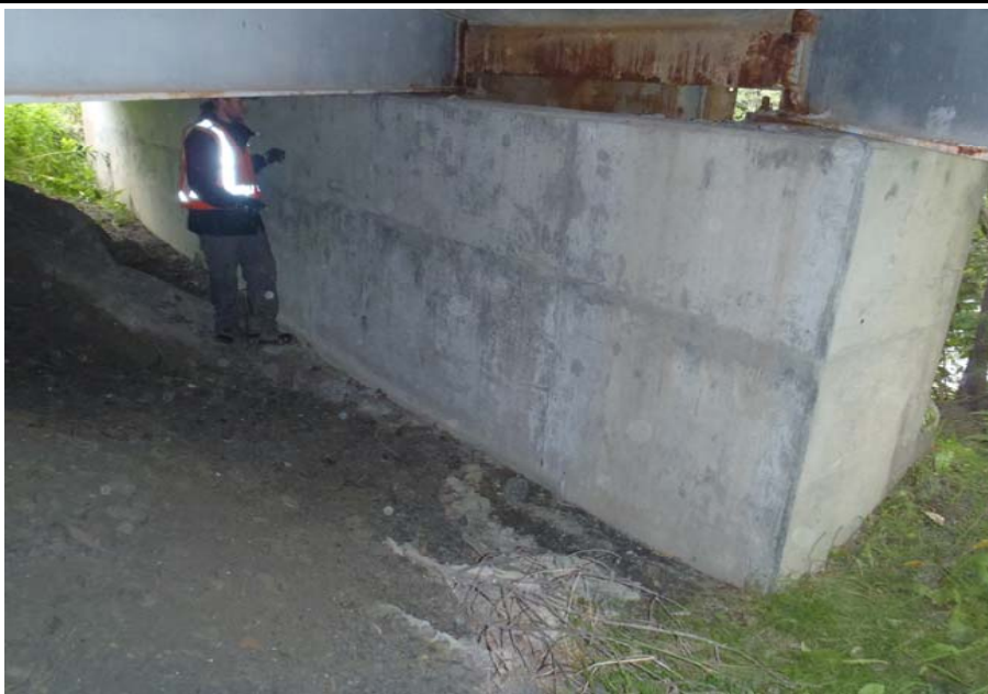
Bridge No. 0607 Br. Name Victor Creek Date 08/09/17 Inspector Murray / Murph Frame 27 NE face Pier 2
