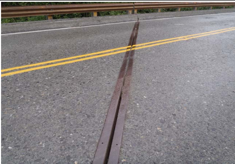
Bridge No. 0607 Br. Name Victor Creek Date 08/09/17 Inspector Murray / Murph Frame 19 DS Pier 4 expansion joint
