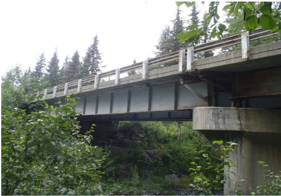
Bridge No. 0607 Br. Name Victor Creek Date 08/09/17 Inspector Murray / Murph Frame 9 US NE elevation
