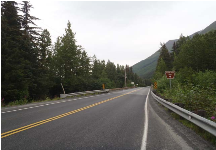
Bridge No. 0607 Br. Name Victor Creek Date 08/09/17 Inspector Murray / Murph Frame 1 Ahead at bridge
