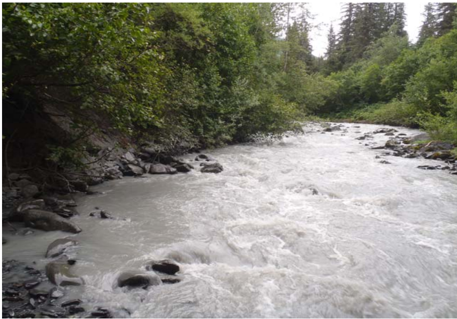
Bridge No. 0607 Br. Name Victor Creek Date 08/09/17 Inspector Murray / Murph Frame 13 FE US undercutting along bank
