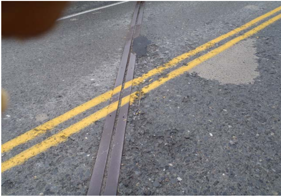
Bridge No. 0607 Br. Name Victor Creek Date 08/09/17 Inspector Murray / Murph Frame 17 Expansion joint 2 exposed rebar at centerline
