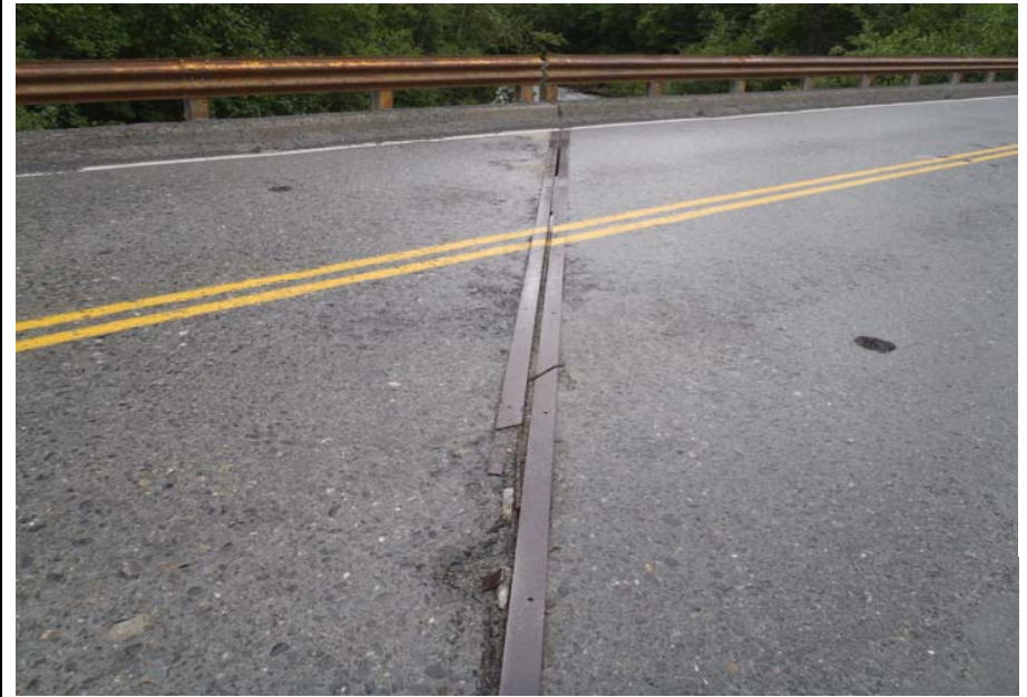
Bridge No. 0607 Br. Name Victor Creek Date 08/09/17 Inspector Murray / Murph Frame 18 DS Pier 3 expansion joint
