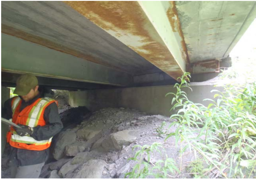
Bridge No. 0607 Br. Name Victor Creek Date 08/09/17 Inspector Murray / Murph Frame 21 DS Abutment 1
