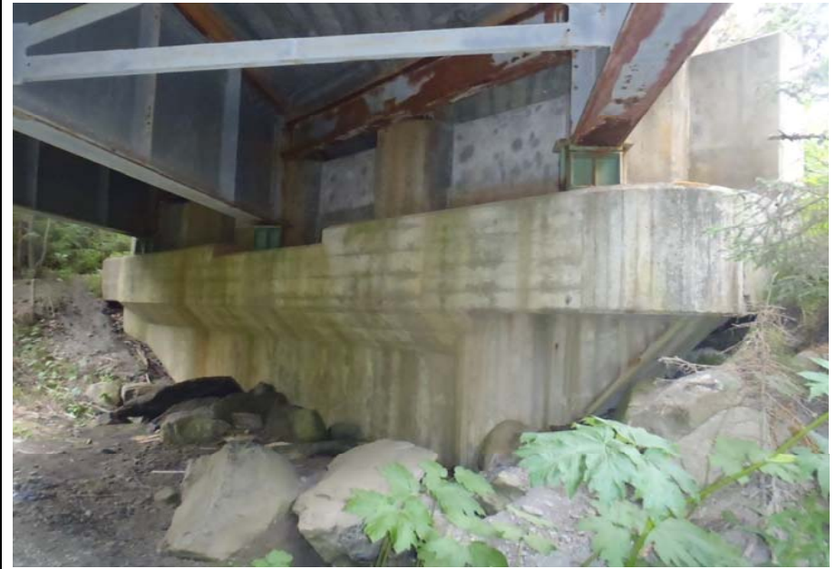
Bridge No. 0607 Br. Name Victor Creek Date 08/09/17 Inspector Murray / Murph Frame 30 DS FE face Pier 2
