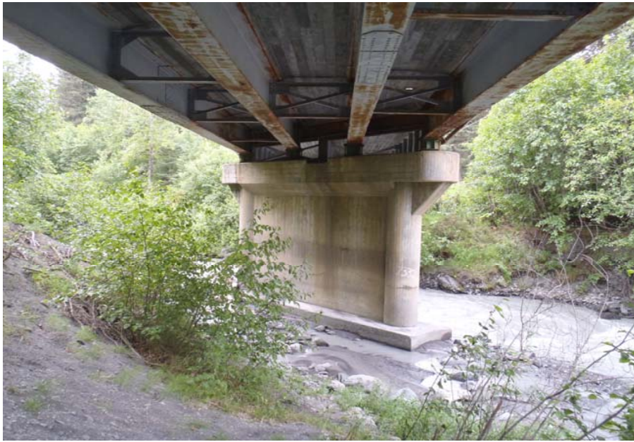
Bridge No. 0607 Br. Name Victor Creek Date 08/09/17 Inspector Murray / Murph Frame 33 FE face pier 3
