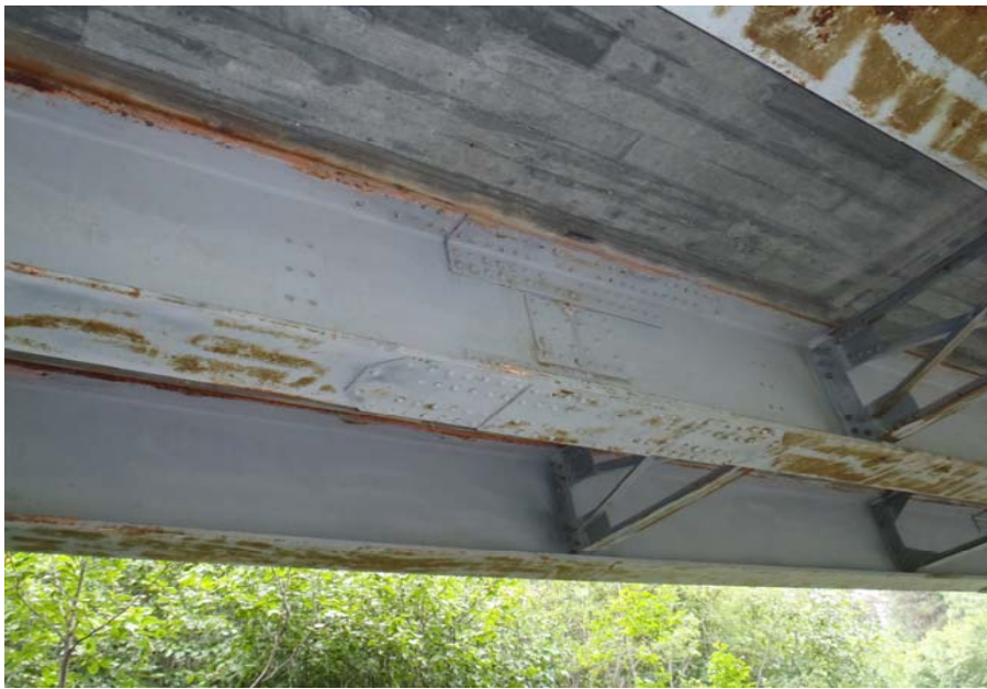
Bridge No. 0607 Br. Name Victor Creek Date 08/09/17 Inspector Murray / Murph Frame 25 Connection joint, typ.
