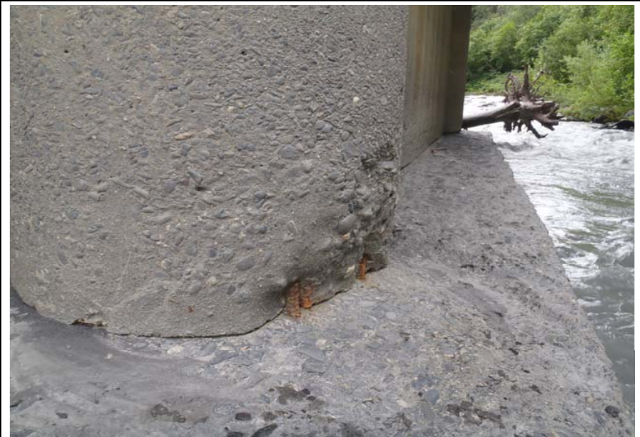
Bridge No. 0607 Br. Name Victor Creek Date 08/09/17 Inspector Murray / Murph Frame 32 DS NE face pier 3 spall with exposed rebar
