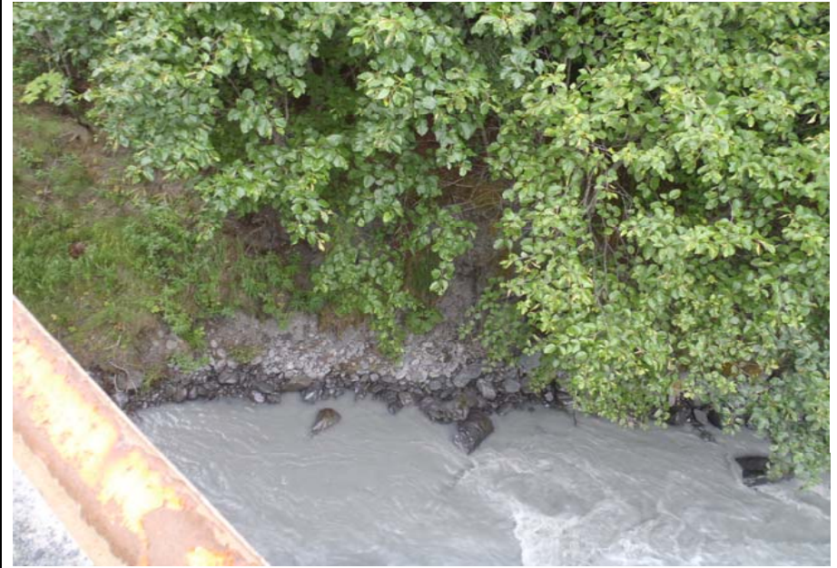
Bridge No. 0607 Br. Name Victor Creek Date 08/09/17 Inspector Murray / Murph Frame 6 Looking NE DS
