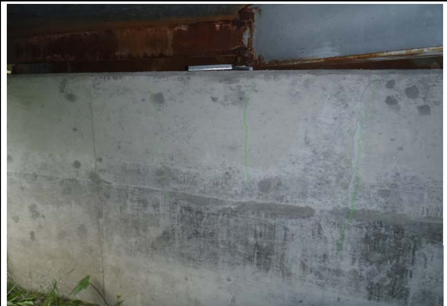
Bridge No. 0607 Br. Name Victor Creek Date 08/09/17 Inspector Murray / Murph Frame 28 NE face Pier 2 cracks
