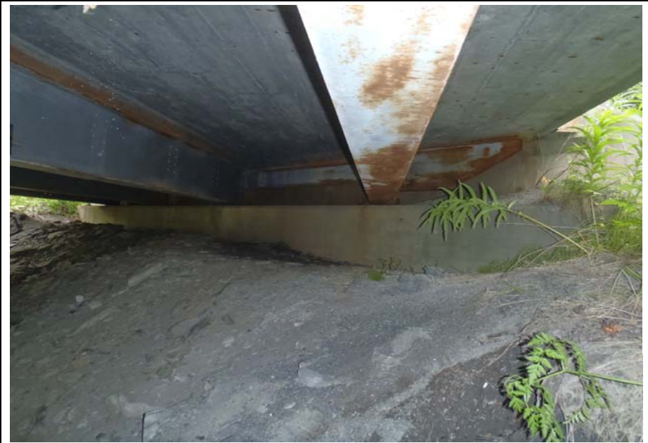
Bridge No. 0607 Br. Name Victor Creek Date 08/09/17 Inspector Murray / Murph Frame 36 Abutment 5
