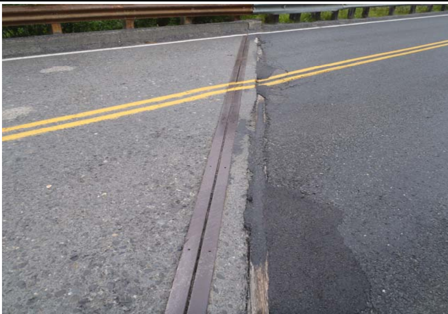
Bridge No. 0607 Br. Name Victor Creek Date 08/09/17 Inspector Murray / Murph Frame 15 DS NE expansion joint
