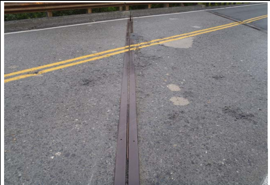
Bridge No. 0607 Br. Name Victor Creek Date 08/09/17 Inspector Murray / Murph Frame 16 DS Pier 2 expansion joint
