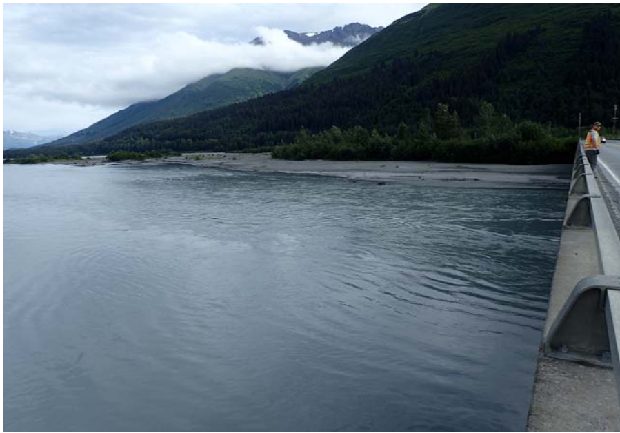
Bridge No. 0605 Br. Name Snow River Cntr Channel Date 08/09/17 Inspector Murray / Murph Frame 13 FE DS island
