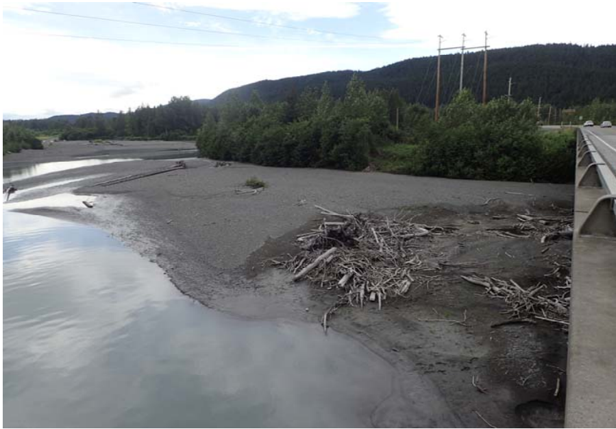
Bridge No. 0605 Br. Name Snow River Cntr Channel Date 08/09/17 Inspector Murray / Murph Frame 9 Looking NE US
