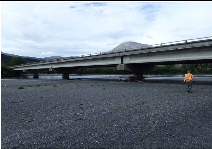
Bridge No. 0605 Br. Name Snow River Cntr Channel Date 08/09/17 Inspector Murray / Murph Frame 3 US elevation
