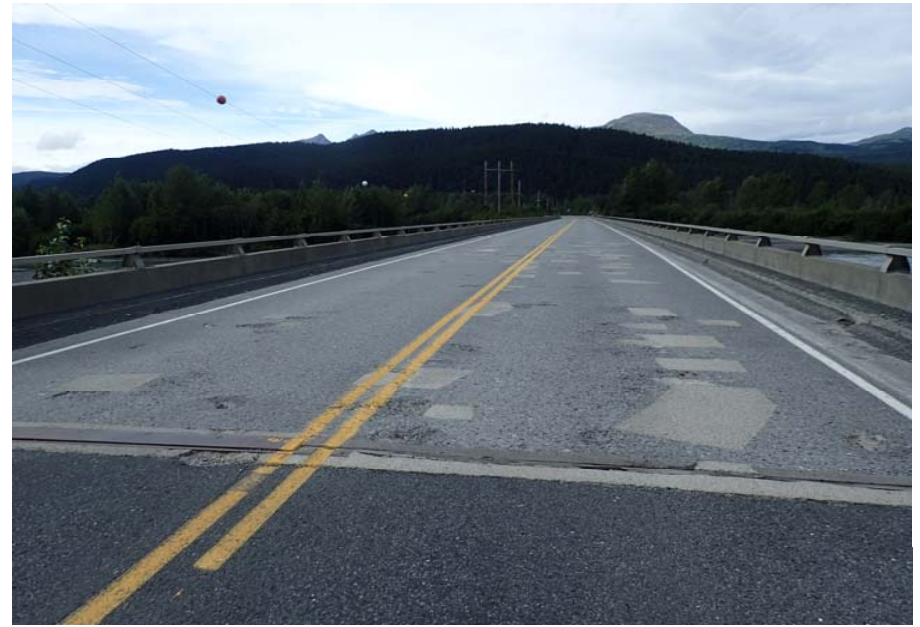
Bridge No. 0605 Br. Name Snow River Cntr Channel Date 08/09/17 Inspector Murray / Murph Frame 2 Back at bridge
