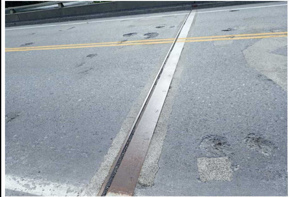
Bridge No. 0605 Br. Name Snow River Cntr Channel Date 08/09/17 Inspector Murray / Murph Frame 22 DS pier 4 expansion joint
