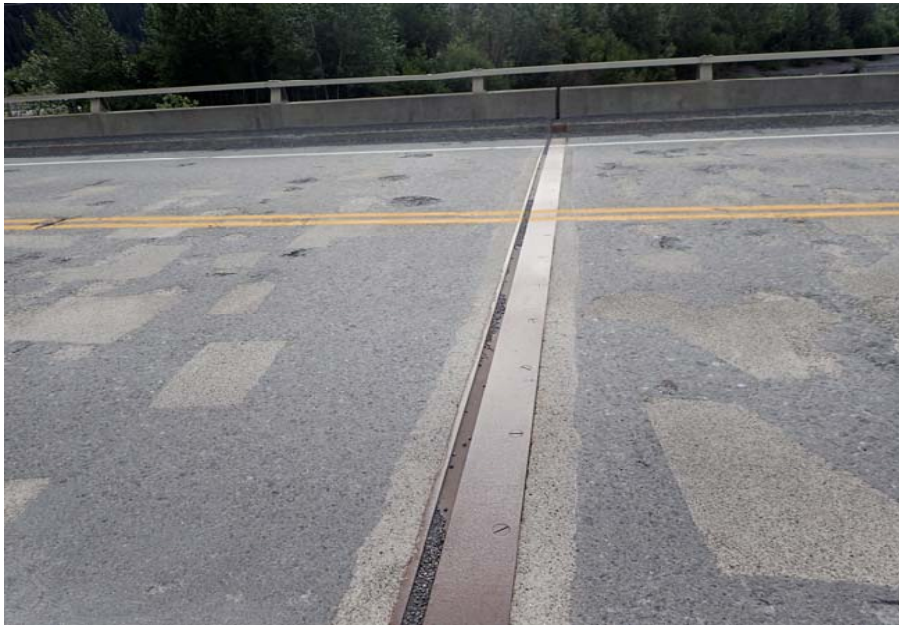
Bridge No. 0605 Br. Name Snow River Cntr Channel Date 08/09/17 Inspector Murray / Murph Frame 21 DS Pier 3 expansion joint
