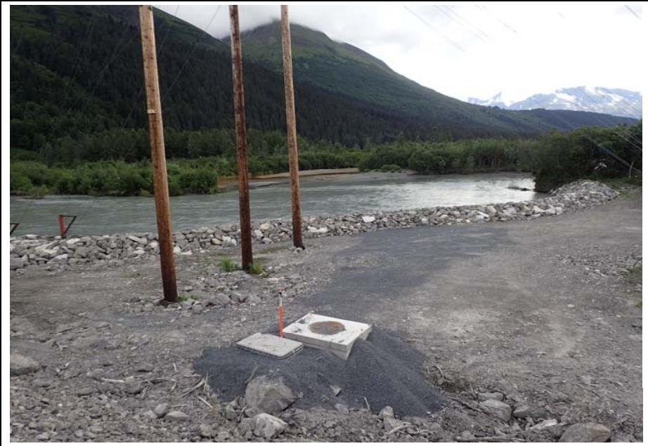
Bridge No. 0605 Br. Name Snow River Cntr Channel Date 08/09/17 Inspector Murray / Murph Frame 40 Looking FE US, note new riprap
