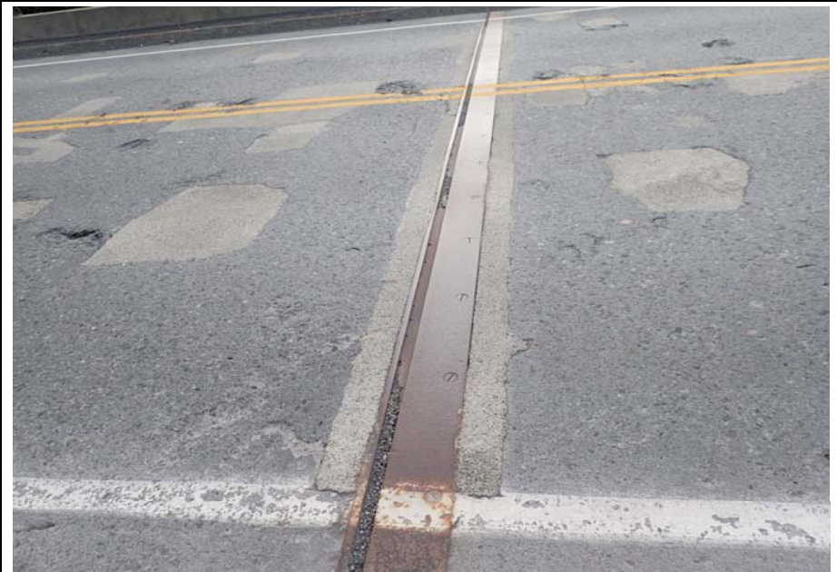
Bridge No. 0605 Br. Name Snow River Cntr Channel Date 08/09/17 Inspector Murray / Murph Frame 20 DS Pier 2 expansion joint
