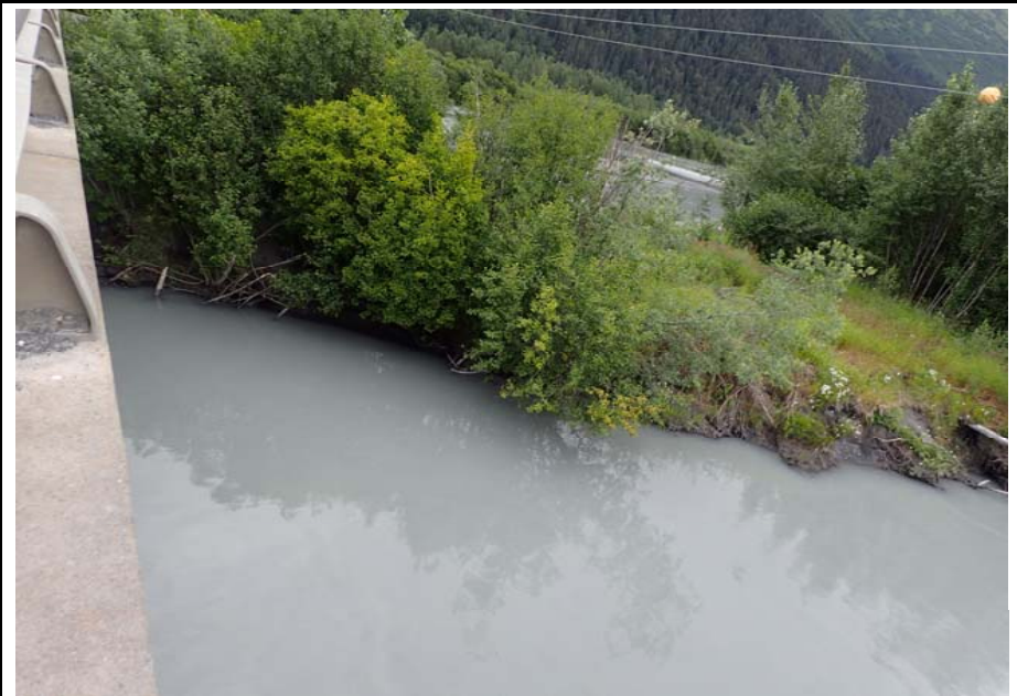
Bridge No. 0605 Br. Name Snow River Cntr Channel Date 08/09/17 Inspector Murray / Murph Frame 12 FE US island
