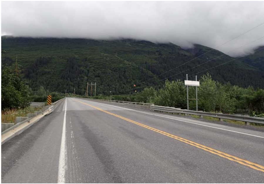
Bridge No. 0605 Br. Name Snow River Cntr Channel Date 08/09/17 Inspector Murray / Murph Frame 1 Ahead at bridge
