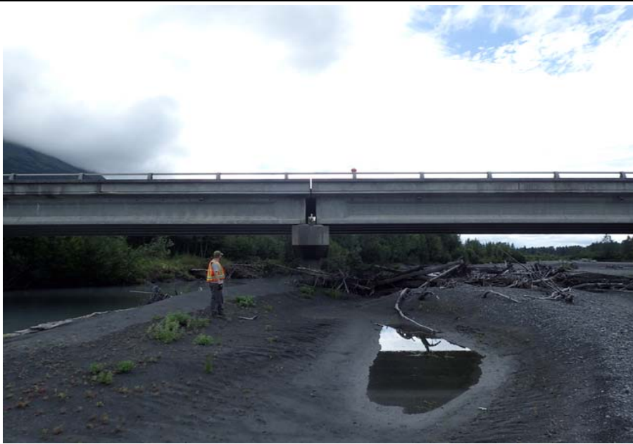
Bridge No. 0605 Br. Name Snow River Cntr Channel Date 08/09/17 Inspector Murray / Murph Frame 31 DS Pier 3 end view
