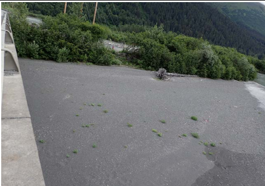
Bridge No. 0605 Br. Name Snow River Cntr Channel Date 08/09/17 Inspector Murray / Murph Frame 15 Looking FE US
