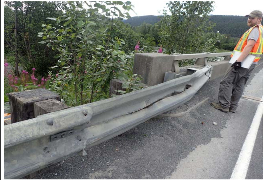
Bridge No. 0605 Br. Name Snow River Cntr Channel Date 08/09/17 Inspector Murray / Murph Frame 18 FE US damaged rail
