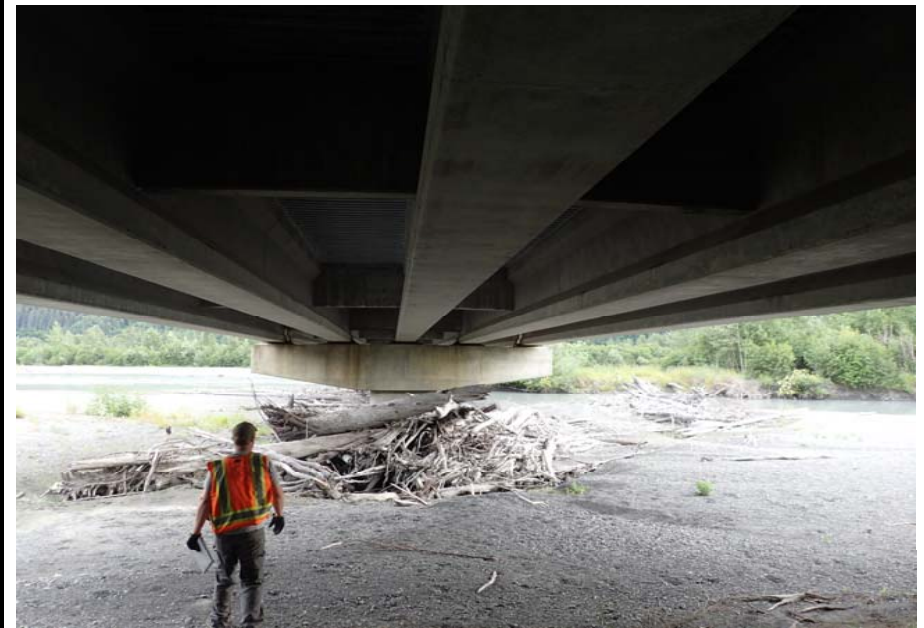
Bridge No. 0605 Br. Name Snow River Cntr Channel Date 08/09/17 Inspector Murray / Murph Frame 28 Pier 2 NE face
