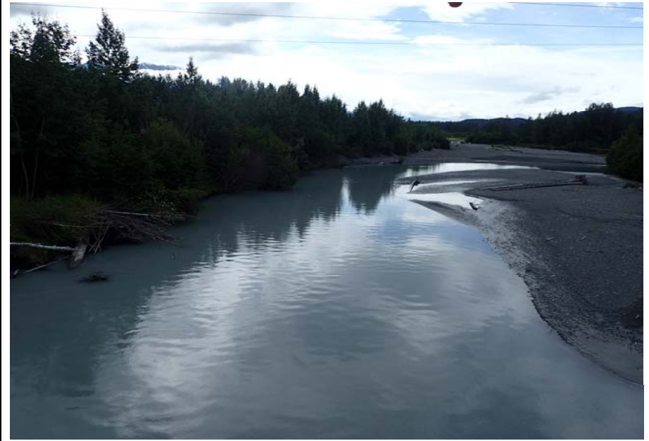
Bridge No. 0605 Br. Name Snow River Cntr Channel Date 08/09/17 Inspector Murray / Murph Frame 6 Looking US 2
