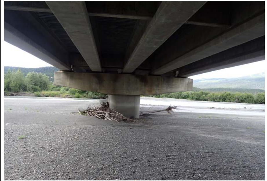
Bridge No. 0605 Br. Name Snow River Cntr Channel Date 08/09/17 Inspector Murray / Murph Frame 34 FE Pier 7
