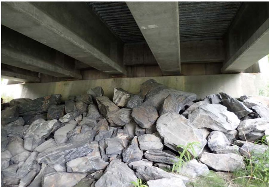
Bridge No. 0605 Br. Name Snow River Cntr Channel Date 08/09/17 Inspector Murray / Murph Frame 27 Abutment 1
