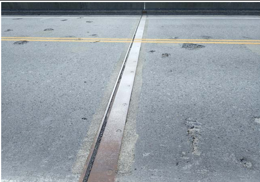
Bridge No. 0605 Br. Name Snow River Cntr Channel Date 08/09/17 Inspector Murray / Murph Frame 23 DS pier 5 expansion joint
