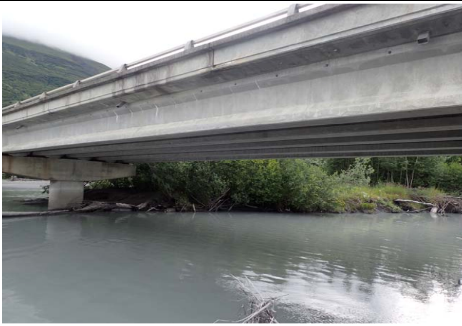
Bridge No. 0605 Br. Name Snow River Cntr Channel Date 08/09/17 Inspector Murray / Murph Frame 39 DS span 3 girder efflorescence
