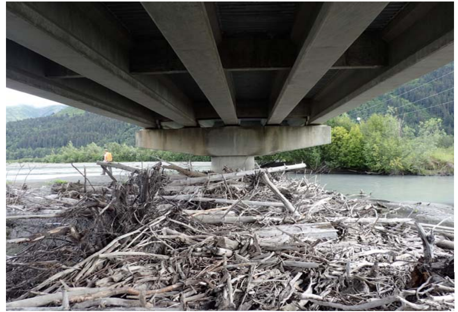
Bridge No. 0605 Br. Name Snow River Cntr Channel Date 08/09/17 Inspector Murray / Murph Frame 30 Pier 3 NE face
