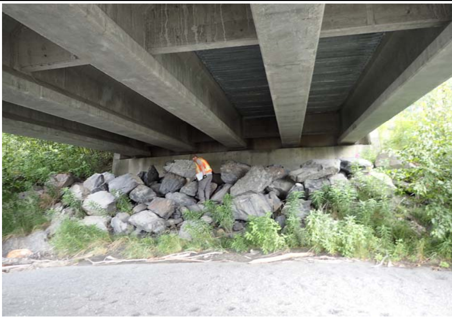
Bridge No. 0605 Br. Name Snow River Cntr Channel Date 08/09/17 Inspector Murray / Murph Frame 35 Abutment 8
