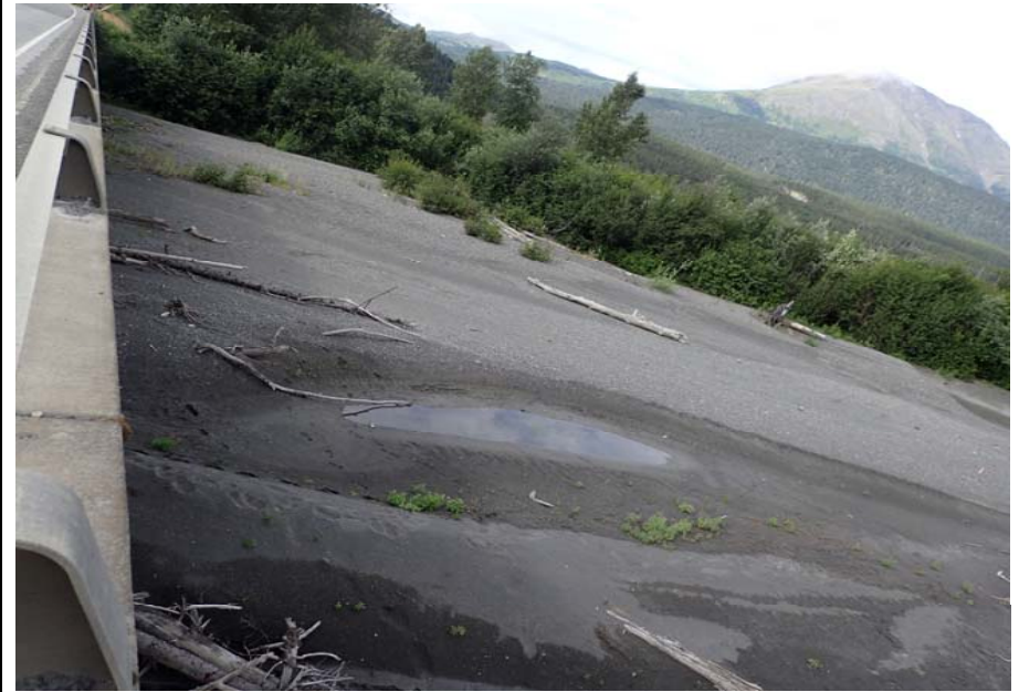
Bridge No. 0605 Br. Name Snow River Cntr Channel Date 08/09/17 Inspector Murray / Murph Frame 10 Looking NE DS
