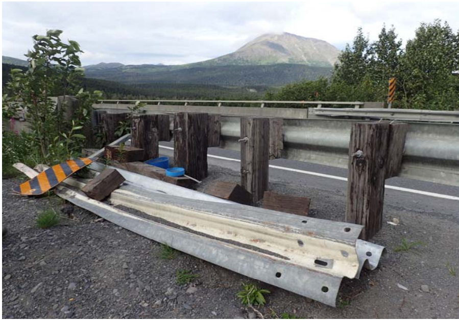
Bridge No. 0605 Br. Name Snow River Cntr Channel Date 08/09/17 Inspector Murray / Murph Frame 17 US FE replacement rail
