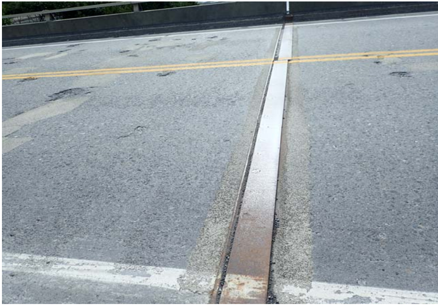
Bridge No. 0605 Br. Name Snow River Cntr Channel Date 08/09/17 Inspector Murray / Murph Frame 25 DS pier 7 expansion joint
