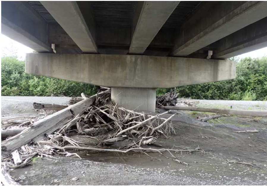
Bridge No. 0605 Br. Name Snow River Cntr Channel Date 08/09/17 Inspector Murray / Murph Frame 29 Pier 2 FE face
