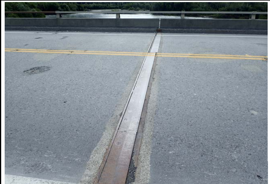
Bridge No. 0605 Br. Name Snow River Cntr Channel Date 08/09/17 Inspector Murray / Murph Frame 24 DS pier 6 expansion joint
