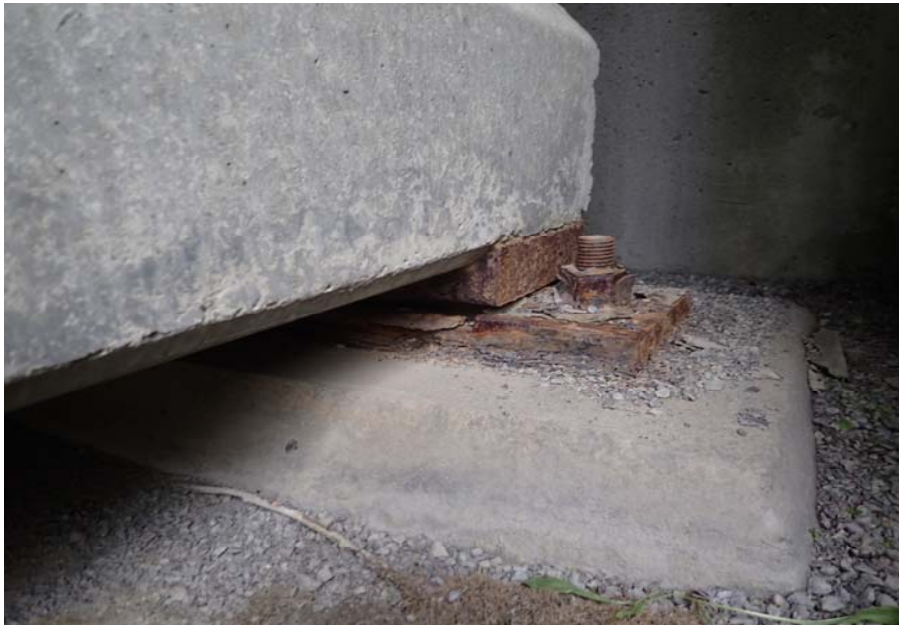
Bridge No. 0605 Br. Name Snow River Cntr Channel Date 08/09/17 Inspector Murray / Murph Frame 37 NE DS bearing, typ.
