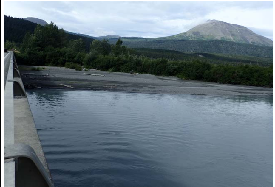
Bridge No. 0605 Br. Name Snow River Cntr Channel Date 08/09/17 Inspector Murray / Murph Frame 14 NE DS island
