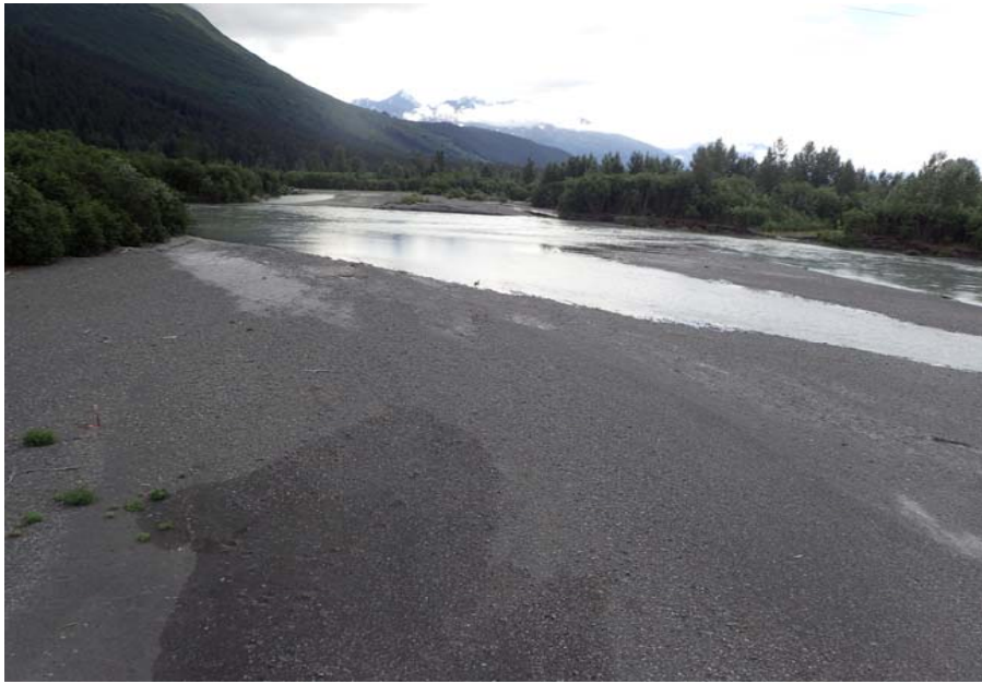
Bridge No. 0605 Br. Name Snow River Cntr Channel Date 08/09/17 Inspector Murray / Murph Frame 5 Looking US 1
