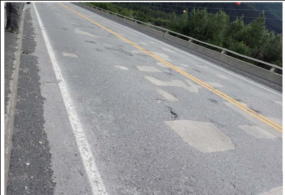
Bridge No. 0605 Br. Name Snow River Cntr Channel Date 08/09/17 Inspector Murray / Murph Frame 16 Wearing surface, typ.
