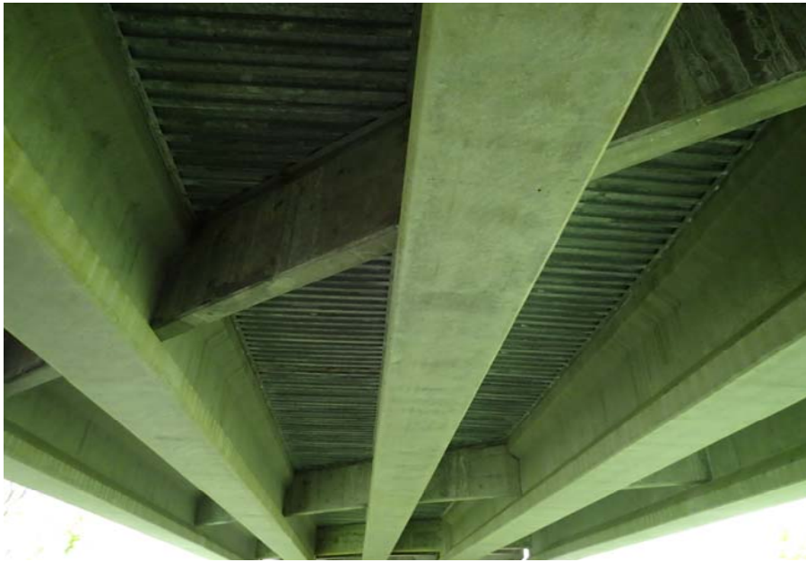
Bridge No. 0603 Br. Name Snow River West Channel Date 08/09/17 Inspector Murray / Murph Frame 17 FE underside, typ.
