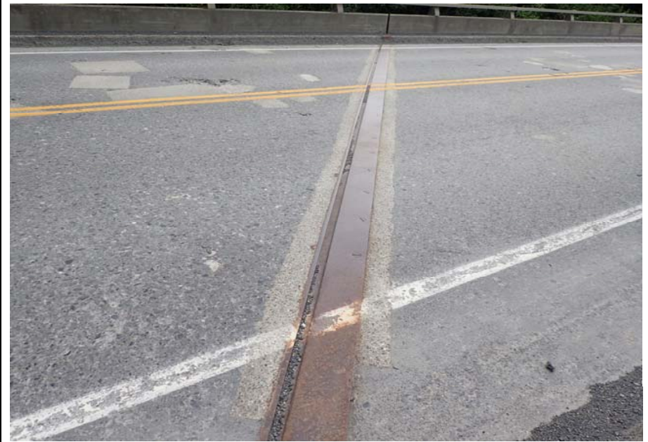
Bridge No. 0603 Br. Name Snow River West Channel Date 08/09/17 Inspector Murray / Murph Frame 12 DS pier 2 expansion joint
