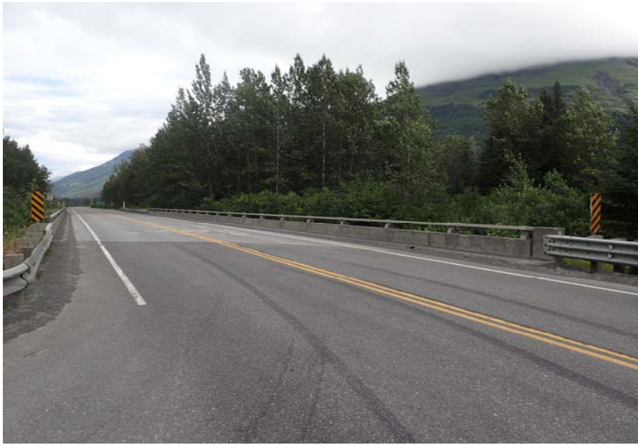
Bridge No. 0603 Br. Name Snow River West Channel Date 08/09/17 Inspector Murray / Murph Frame 1 Ahead at bridge
