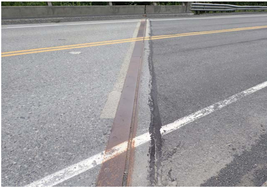
Bridge No. 0603 Br. Name Snow River West Channel Date 08/09/17 Inspector Murray / Murph Frame 11 DS NE expansion joint
