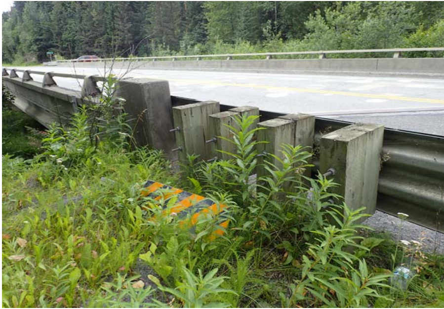
Bridge No. 0603 Br. Name Snow River West Channel Date 08/09/17 Inspector Murray / Murph Frame 9 FE US broken object marker
