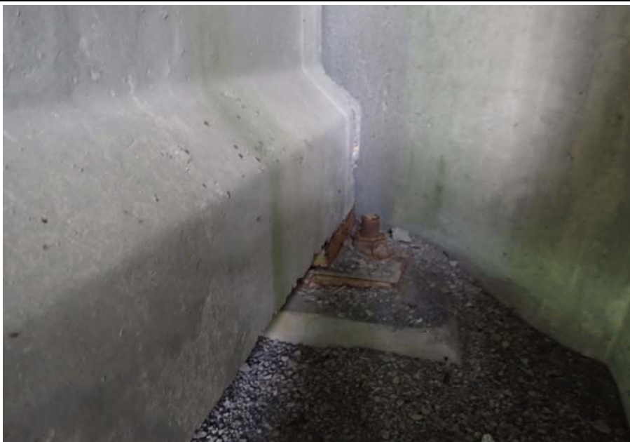
Bridge No. 0603 Br. Name Snow River West Channel Date 08/09/17 Inspector Murray / Murph Frame 19 FE bearing, typ.
