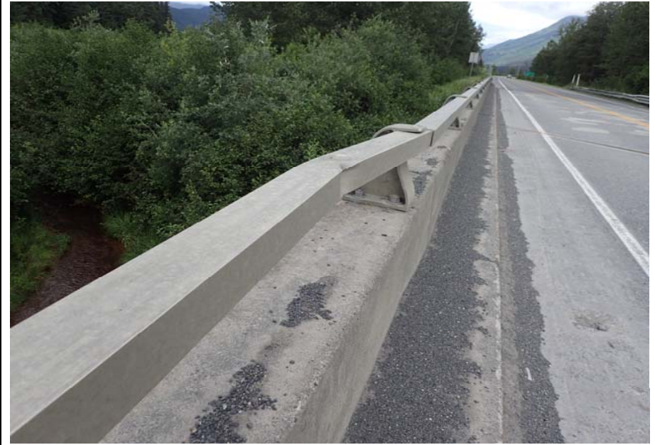
Bridge No. 0603 Br. Name Snow River West Channel Date 08/09/17 Inspector Murray / Murph Frame 10 DS rail dented
