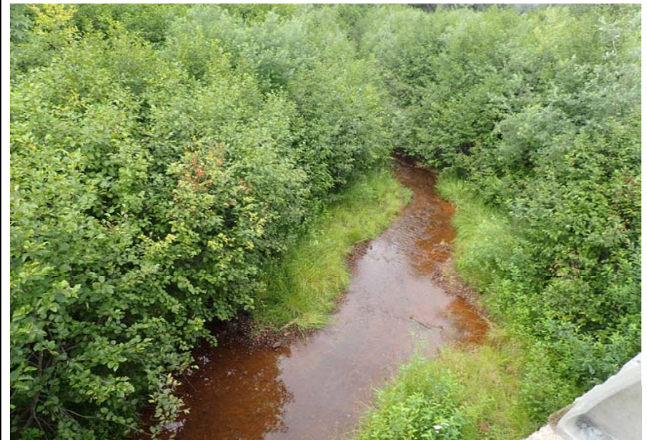
Bridge No. 0603 Br. Name Snow River West Channel Date 08/09/17 Inspector Murray / Murph Frame 4 Looking DS
