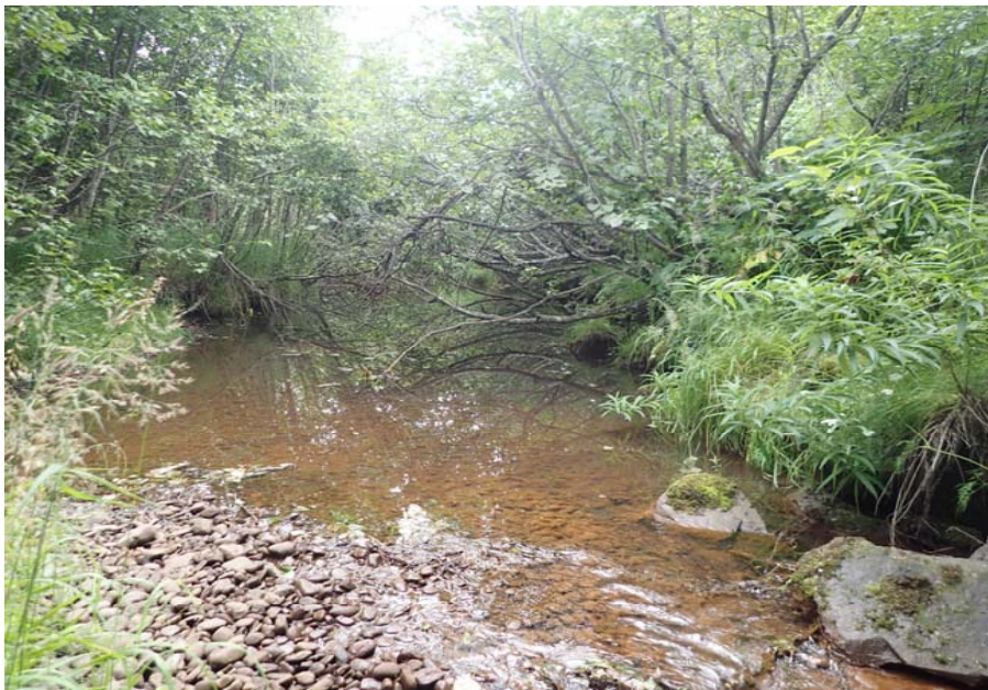
Bridge No. 0603 Br. Name Snow River West Channel Date 08/09/17 Inspector Murray / Murph Frame 3 Looking US
