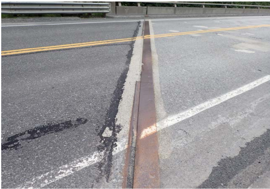
Bridge No. 0603 Br. Name Snow River West Channel Date 08/09/17 Inspector Murray / Murph Frame 13 DS FE expansion joint
