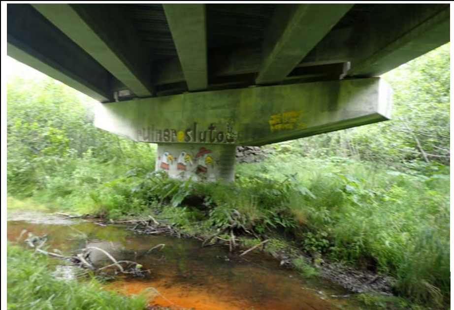
Bridge No. 0603 Br. Name Snow River West Channel Date 08/09/17 Inspector Murray / Murph Frame 16 Pier 2 FE face
