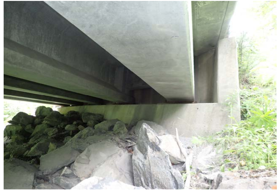
Bridge No. 0603 Br. Name Snow River West Channel Date 08/09/17 Inspector Murray / Murph Frame 18 Abutment 3
