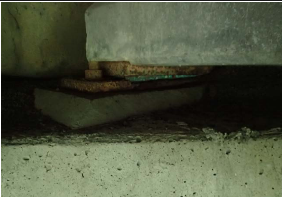
Bridge No. 0603 Br. Name Snow River West Channel Date 08/09/17 Inspector Murray / Murph Frame 15 NE bearing, typ.
