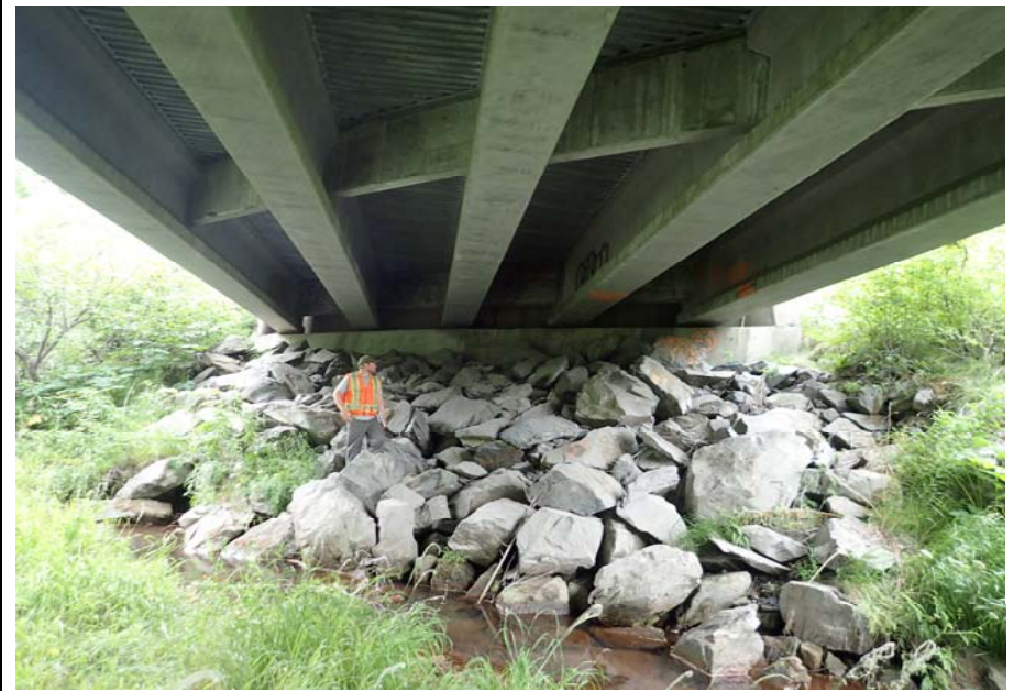
Bridge No. 0603 Br. Name Snow River West Channel Date 08/09/17 Inspector Murray / Murph Frame 14 Abutment 1
