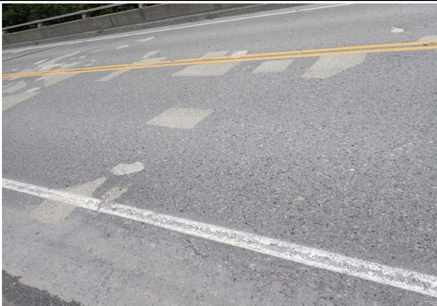
Bridge No. 0603 Br. Name Snow River West Channel Date 08/09/17 Inspector Murray / Murph Frame 7 Wearing surface, typ.
