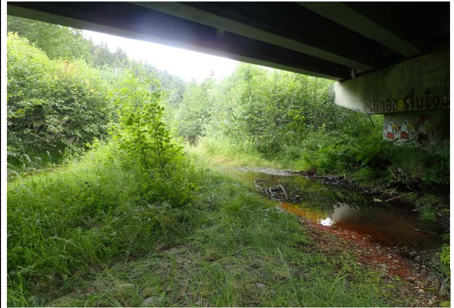
Bridge No. 0603 Br. Name Snow River West Channel Date 08/09/17 Inspector Murray / Murph Frame 6 Looking DS from below
