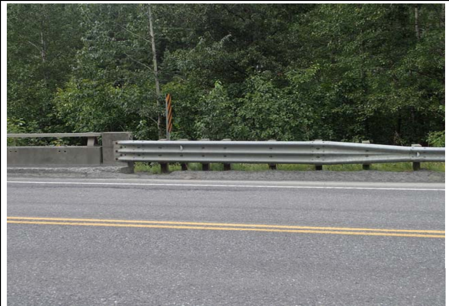
Bridge No. 0603 Br. Name Snow River West Channel Date 08/09/17 Inspector Murray / Murph Frame 8 Transition rail, typ.
