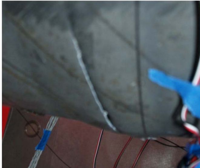
Figure 3-97: Rupture on underside of pile, \Delta = 8.98 in
