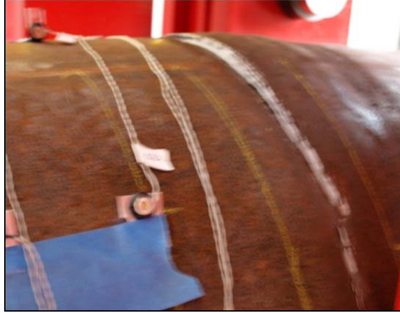
Figure 3-51: Pile Rupture, ductility five ( \Delta = 15 inches)
