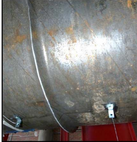
Figure 3-164: Crack on underside of the pile closing, first pull of ductility 5, \Delta=11.5 in
