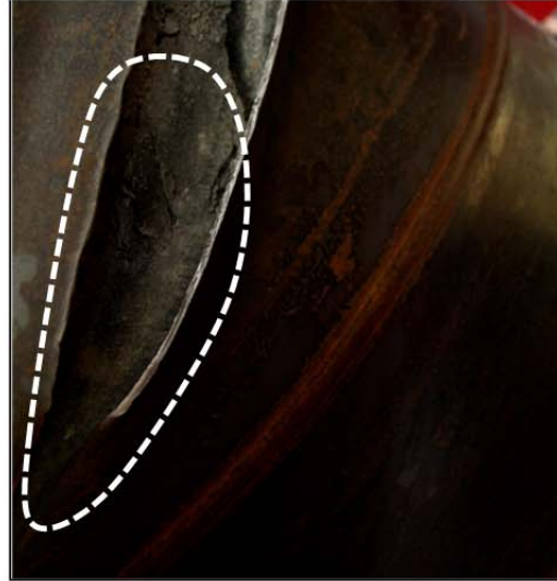
Figure 3-32: Concrete is still intact after rupture occurred where buckling had not
