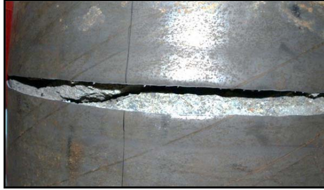
Figure 3-161: Crack opening on the pile at ductility 5, \Delta=11.5 in
