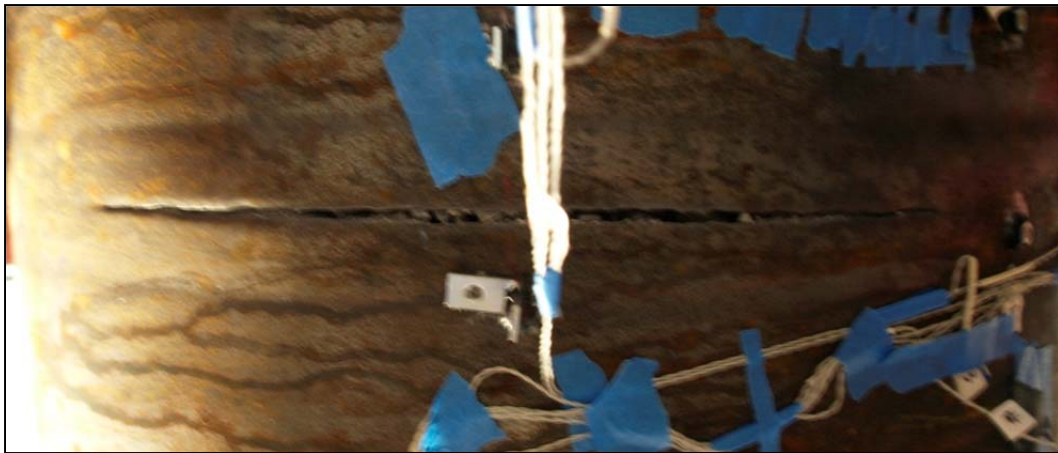
Figure 3-30: Rupture during the second push of ductility six, at a displacement of 12.5 inches
