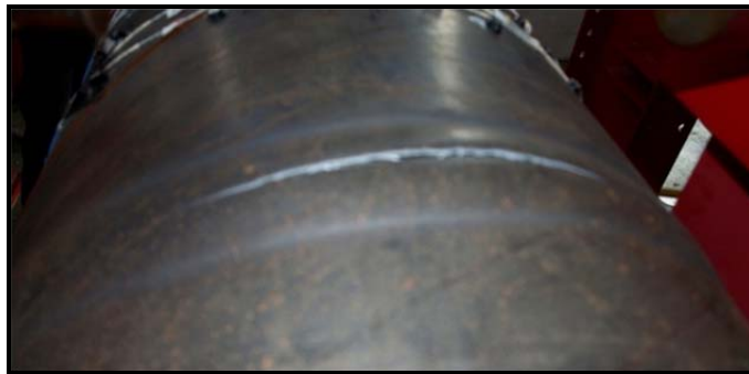
Figure 3-186: Rupture of the steel pile, en route ductility 6-1st pull
