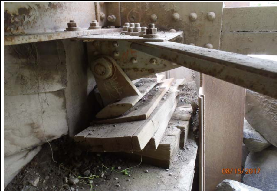
Bridge No. 1193 Br. Name Chokosna River Date 08/15/17 Inspector Levings / Henry Frame 16 NE US bearing, rotated approximately 14 degrees
