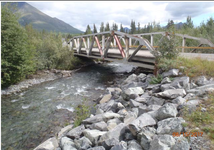
Bridge No. 1193 Br. Name Chokosna River Date 08/15/17 Inspector Levings / Henry Frame 3 Elevation looking DS
