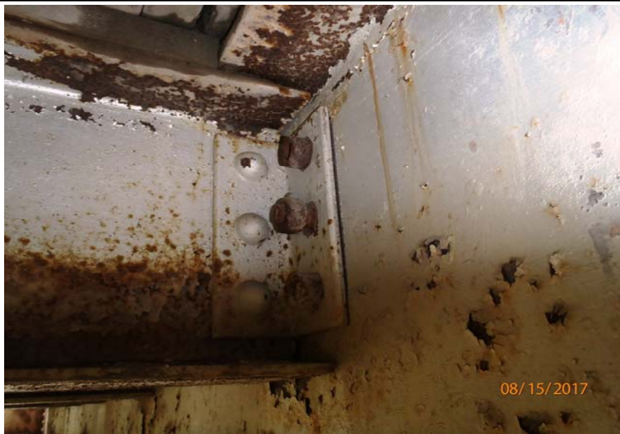
Bridge No. 1193 Br. Name Chokosna River Date 08/15/17 Inspector Levings / Henry Frame 31 Loose bolt at floorbeam 2', NE, stringer 3
