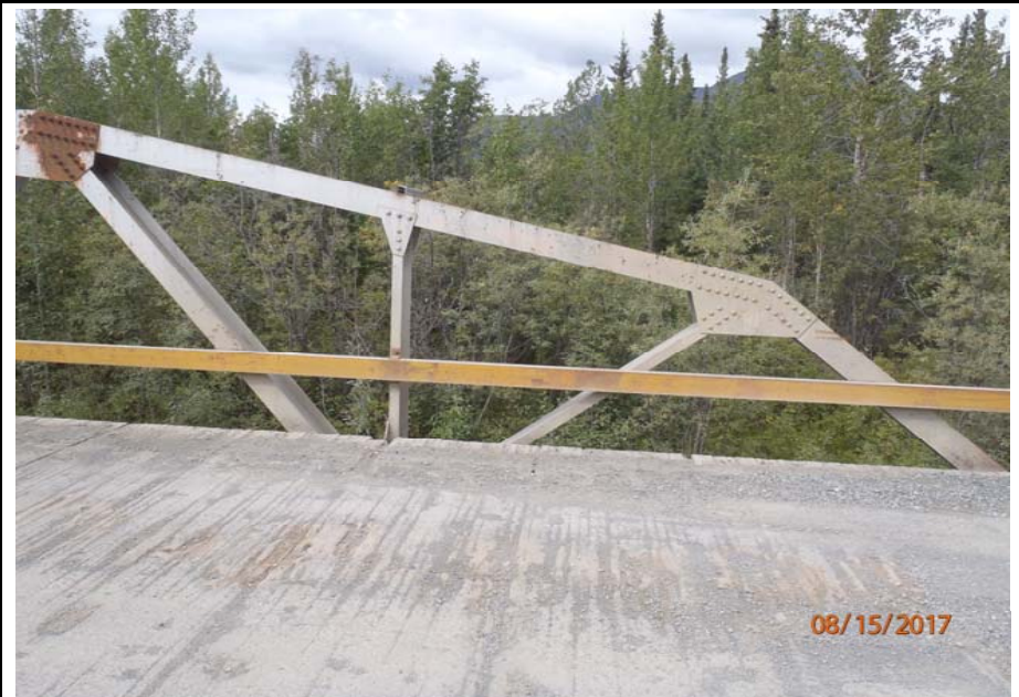
Bridge No. 1193 Br. Name Chokosna River Date 08/15/17 Inspector Levings / Henry Frame 24 US truss, 4 of 4, NE to FE
