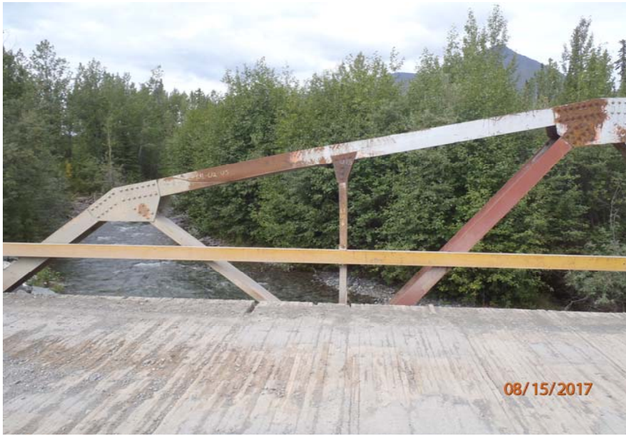
Bridge No. 1193 Br. Name Chokosna River Date 08/15/17 Inspector Levings / Henry Frame 21 US truss, 1 of 4, NE to FE
