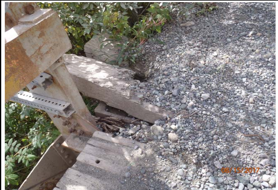
Bridge No. 1193 Br. Name Chokosna River Date 08/15/17 Inspector Levings / Henry Frame 12 NE DS transition, broken timber plank
