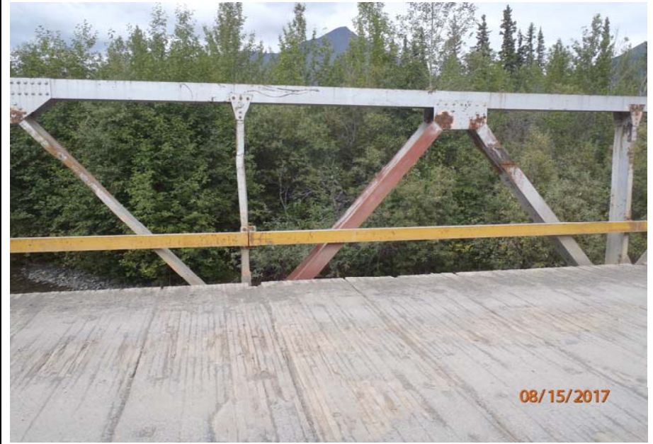
Bridge No. 1193 Br. Name Chokosna River Date 08/15/17 Inspector Levings / Henry Frame 22 US truss, 2 of 4, NE to FE
