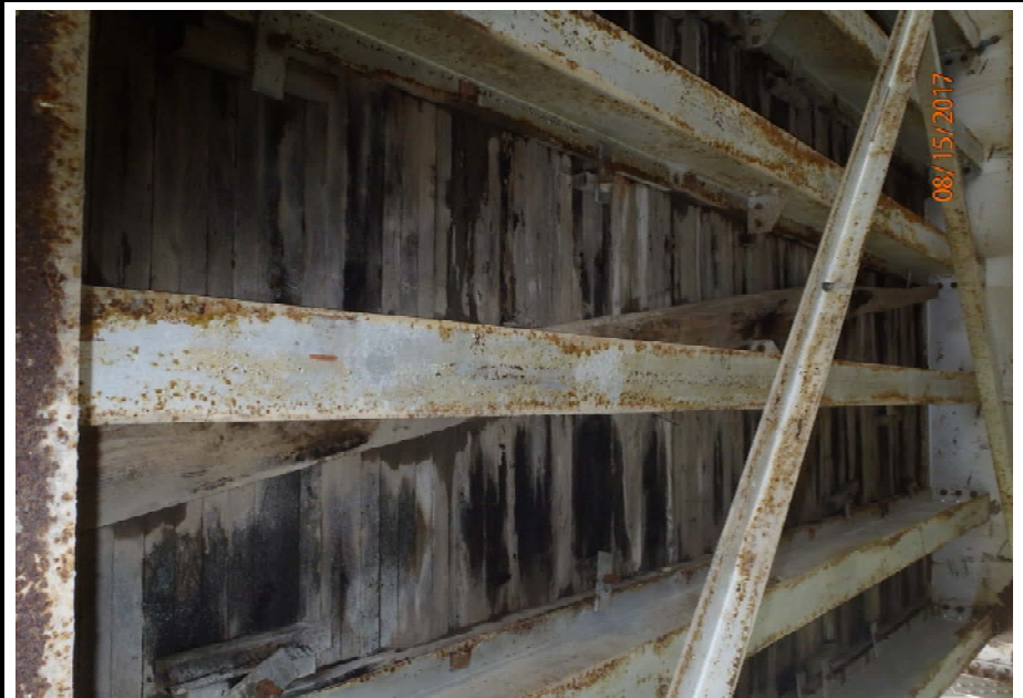
Bridge No. 1193 Br. Name Chokosna River Date 08/15/17 Inspector Levings / Henry Frame 32 Deck nailer board displaced between floorbeam 2'-1', stringer 3
