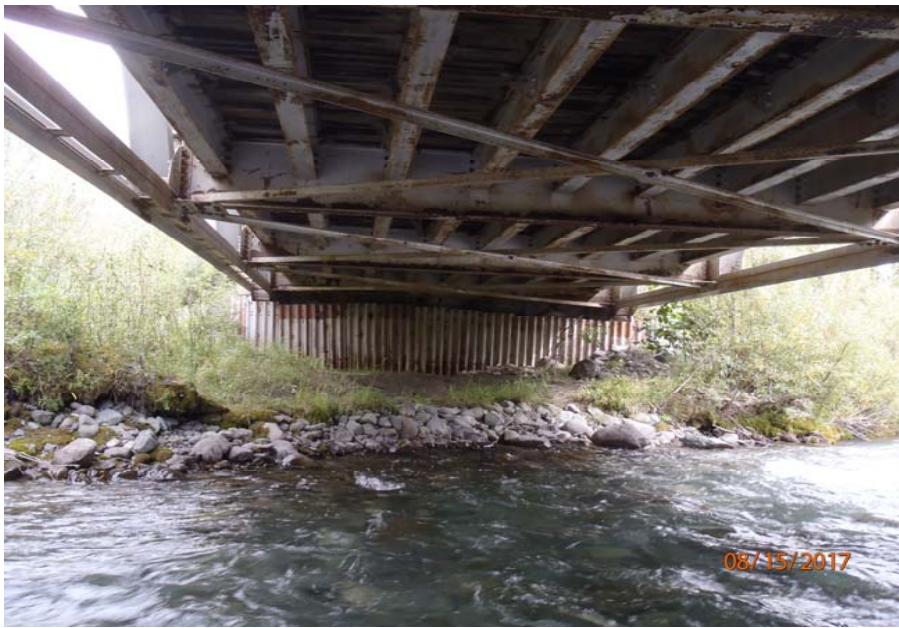
Bridge No. 1193 Br. Name Chokosna River Date 08/15/17 Inspector Levings / Henry Frame 17 FE abutment and US low chord with vertical bends
