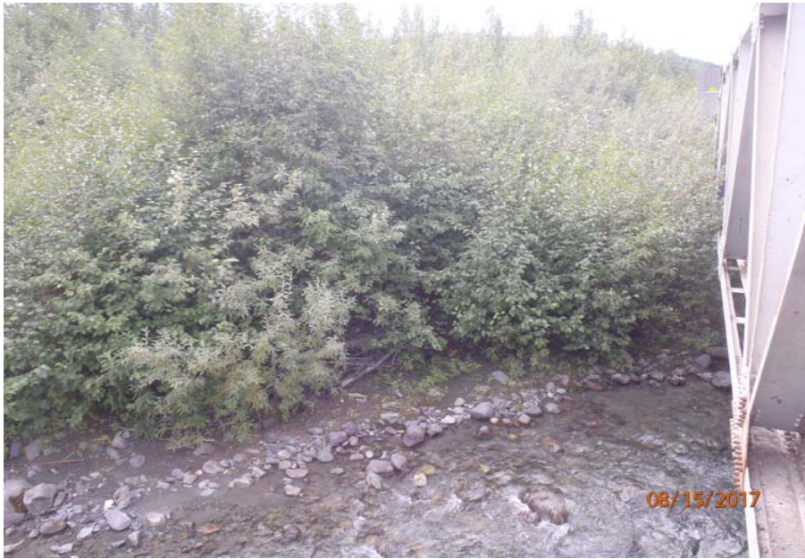
Bridge No. 1193 Br. Name Chokosna River Date 08/15/17 Inspector Levings / Henry Frame 5 NE DS bank
