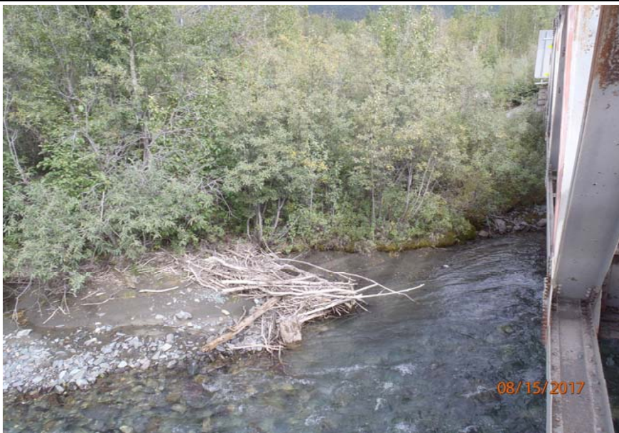
Bridge No. 1193 Br. Name Chokosna River Date 08/15/17 Inspector Levings / Henry Frame 7 FE US bank
