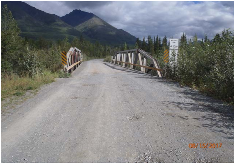
Bridge No. 1193 Br. Name Chokosna River Date 08/15/17 Inspector Levings / Henry Frame 1 NE approach
