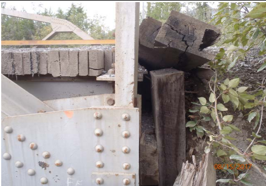
Bridge No. 1193 Br. Name Chokosna River Date 08/15/17 Inspector Levings / Henry Frame 11 FE DS corner, broken timber at approach transition
