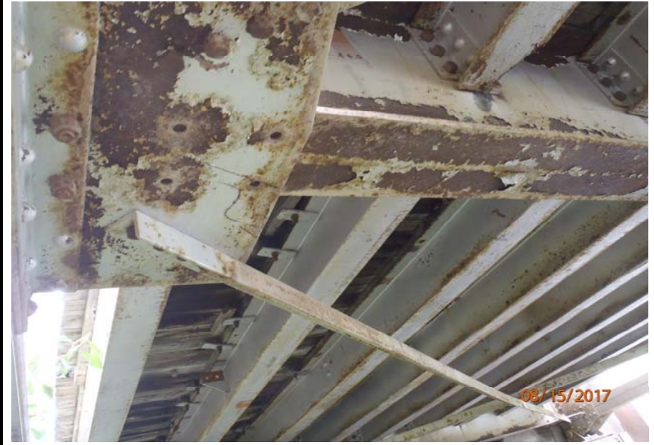
Bridge No. 1193 Br. Name Chokosna River Date 08/15/17 Inspector Levings / Henry Frame 30 Floorbeam at L1, missing 4 bolts
