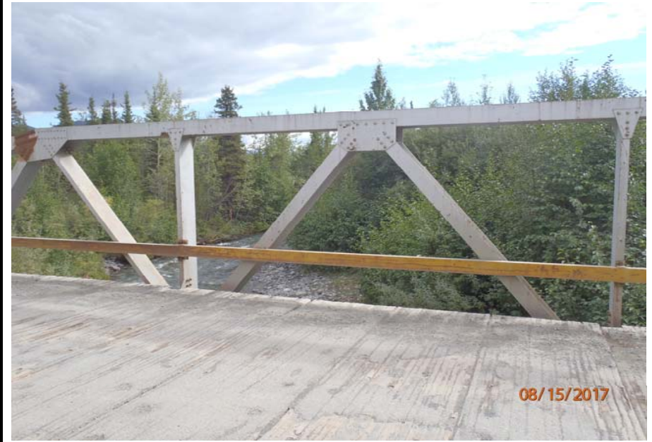
Bridge No. 1193 Br. Name Chokosna River Date 08/15/17 Inspector Levings / Henry Frame 26 DS truss, 3 of 4, FE to NE
