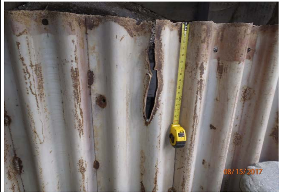
Bridge No. 1193 Br. Name Chokosna River Date 08/15/17 Inspector Levings / Henry Frame 18 FE abutment sheet pile wall, torn
