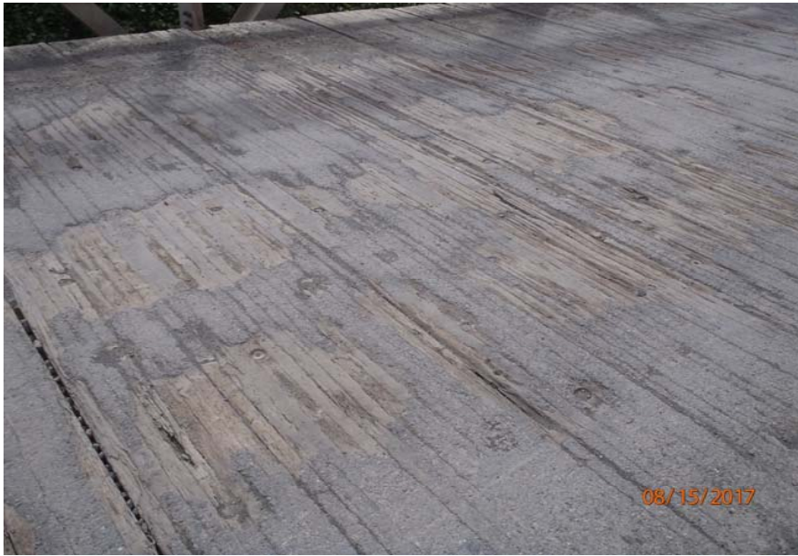
Bridge No. 1193 Br. Name Chokosna River Date 08/15/17 Inspector Levings / Henry Frame 9 Deck condition, typical
