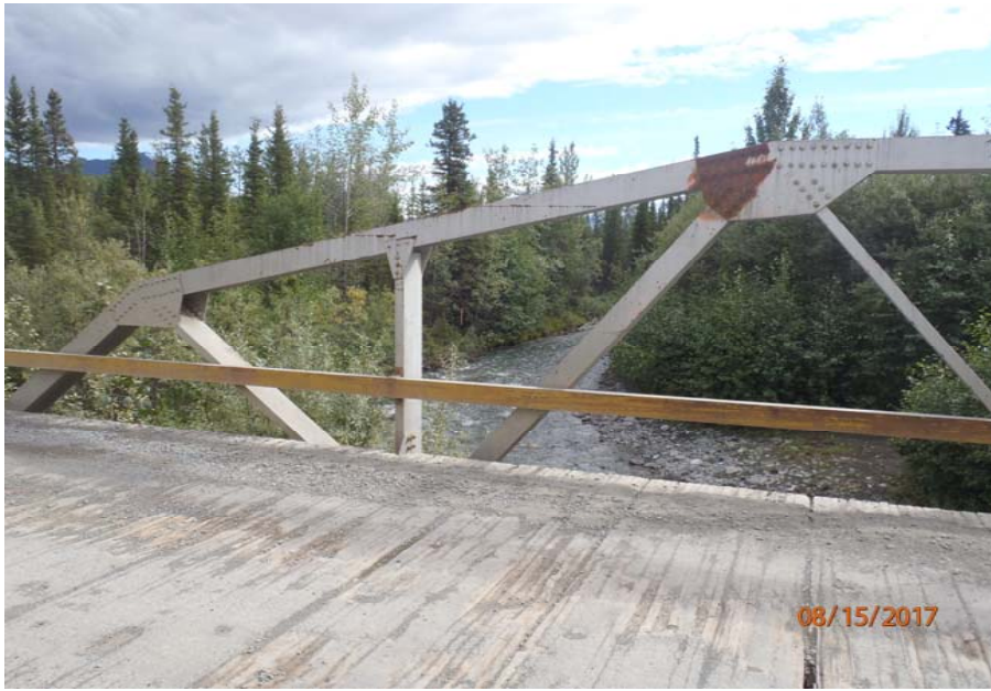
Bridge No. 1193 Br. Name Chokosna River Date 08/15/17 Inspector Levings / Henry Frame 25 DS truss, 4 of 4, FE to NE
