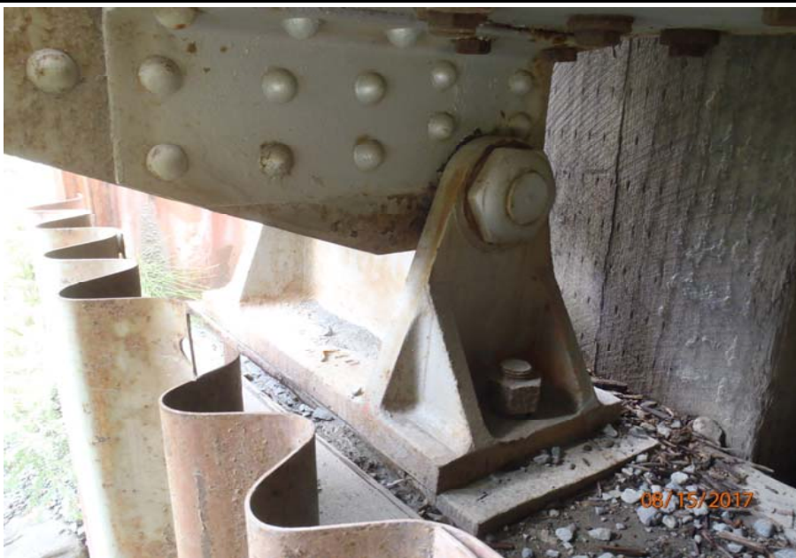
Bridge No. 1193 Br. Name Chokosna River Date 08/15/17 Inspector Levings / Henry Frame 19 FE abutment, bearing 1
