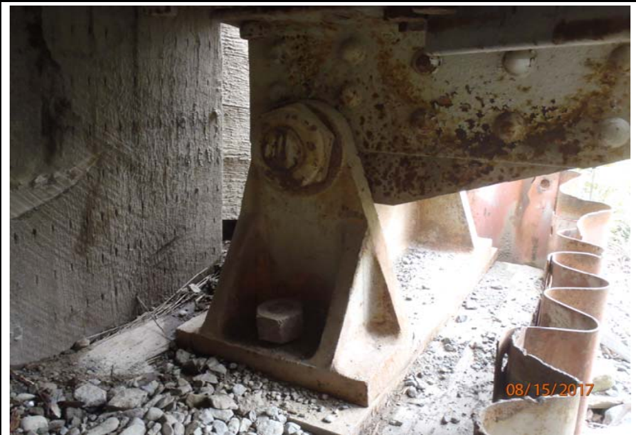
Bridge No. 1193 Br. Name Chokosna River Date 08/15/17 Inspector Levings / Henry Frame 20 FE abutment, bearing 2
