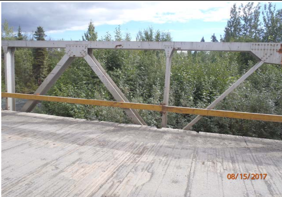
Bridge No. 1193 Br. Name Chokosna River Date 08/15/17 Inspector Levings / Henry Frame 27 DS truss, 2 of 4, FE to NE
