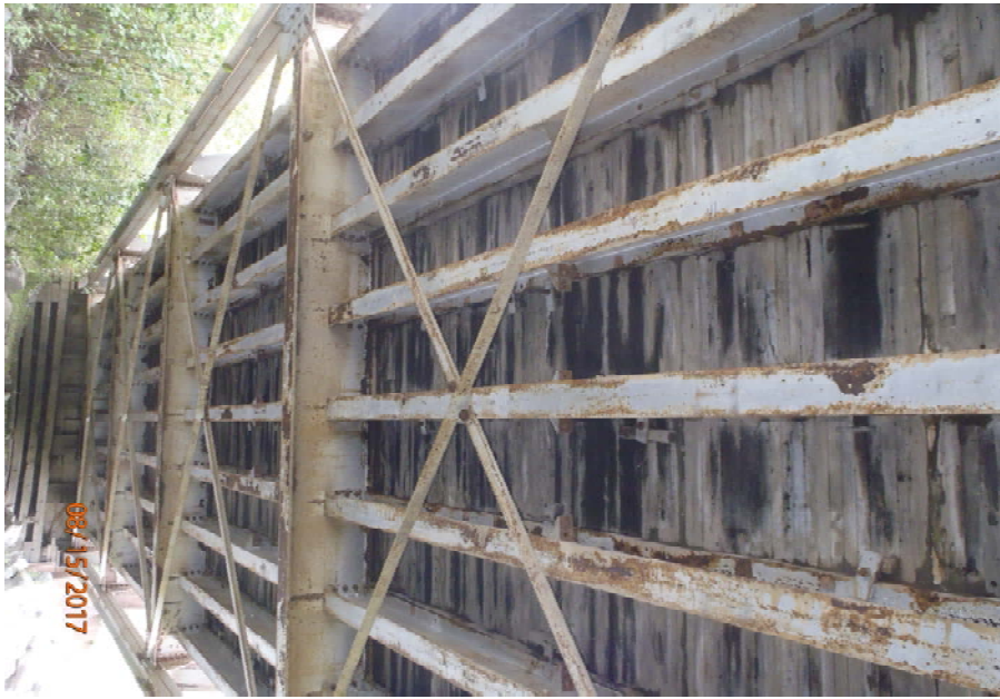
Bridge No. 1193 Br. Name Chokosna River Date 08/15/17 Inspector Levings / Henry Frame 29 Underside, typical, looking towards NE
