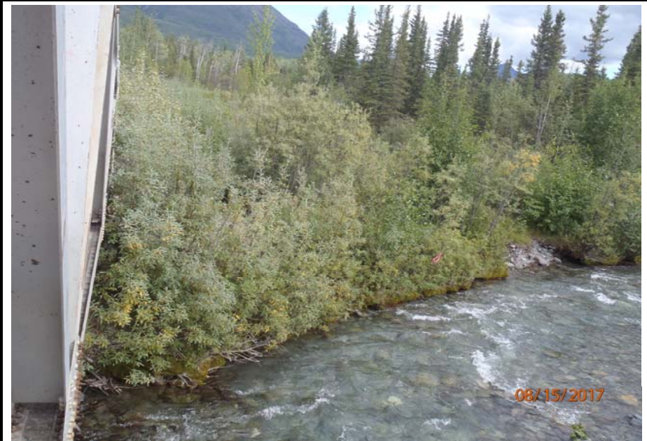
Bridge No. 1193 Br. Name Chokosna River Date 08/15/17 Inspector Levings / Henry Frame 8 NE DS bank
