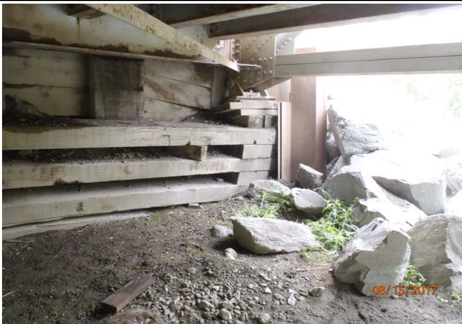
Bridge No. 1193 Br. Name Chokosna River Date 08/15/17 Inspector Levings / Henry Frame 15 NE abutment and US bearing
