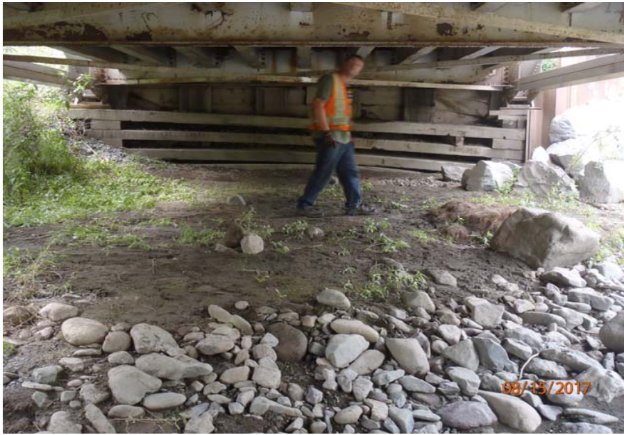
Bridge No. 1193 Br. Name Chokosna River Date 08/15/17 Inspector Levings / Henry Frame 13 NE abutment with settlement of US corner
