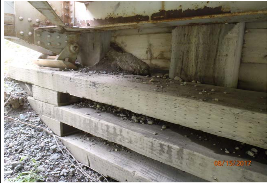
Bridge No. 1193 Br. Name Chokosna River Date 08/15/17 Inspector Levings / Henry Frame 14 NE abutment and DS bearing
