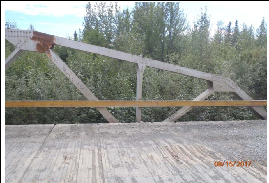
Bridge No. 1193 Br. Name Chokosna River Date 08/15/17 Inspector Levings / Henry Frame 28 DS truss, 1 of 4, FE to NE
