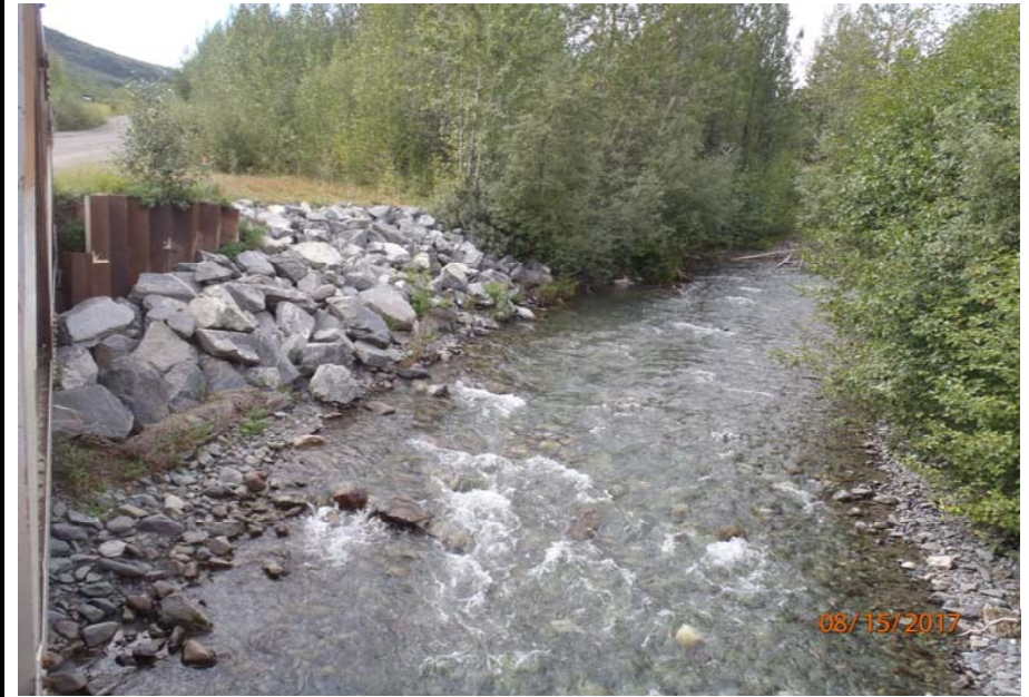
Bridge No. 1193 Br. Name Chokosna River Date 08/15/17 Inspector Levings / Henry Frame 6 Looking US at NE US bank
