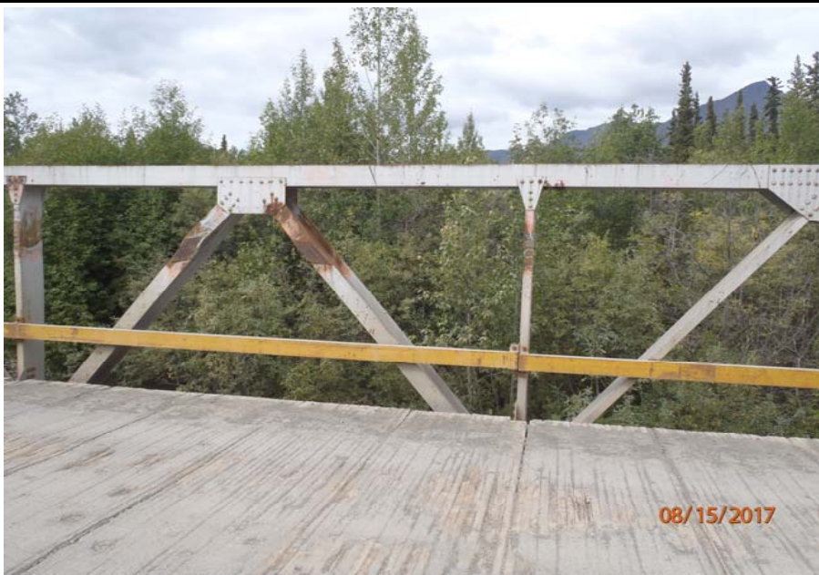
Bridge No. 1193 Br. Name Chokosna River Date 08/15/17 Inspector Levings / Henry Frame 23 US truss, 3 of 4, NE to FE
