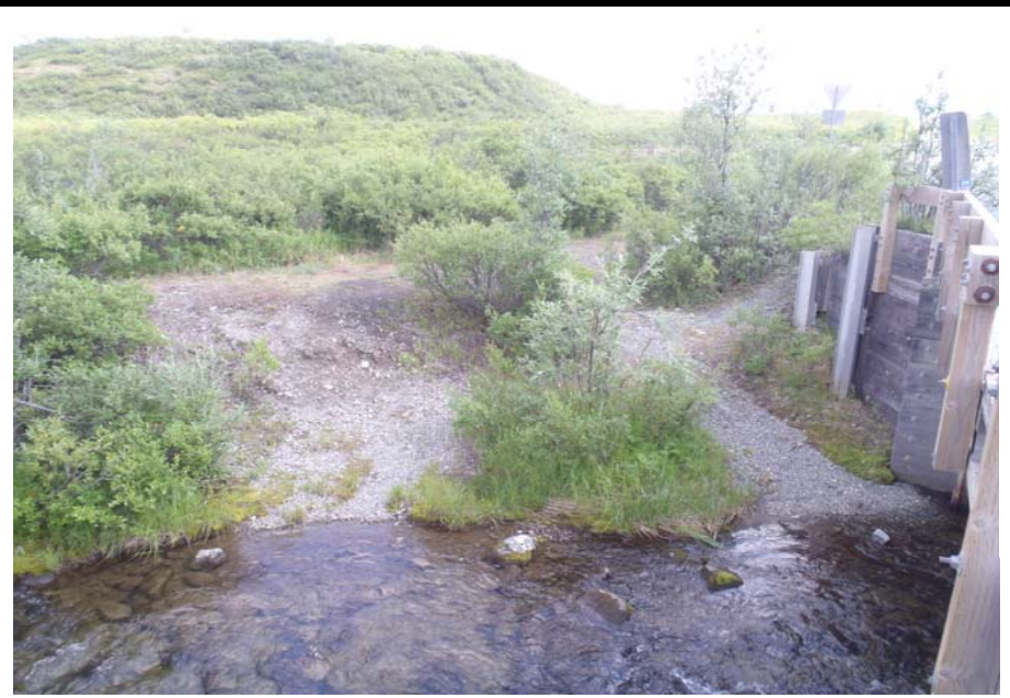
Bridge No. 0684 Br. Name Rock Creek Date 07/14/17 Inspector Murray / Knapp Frame 8 US FE Bank
