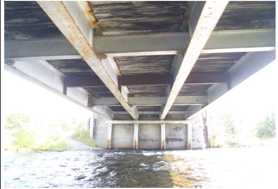
Bridge No. 0684 Br. Name Rock Creek Date 07/14/17 Inspector Murray / Knapp Frame 10 Underside view from NE, FE abutment
