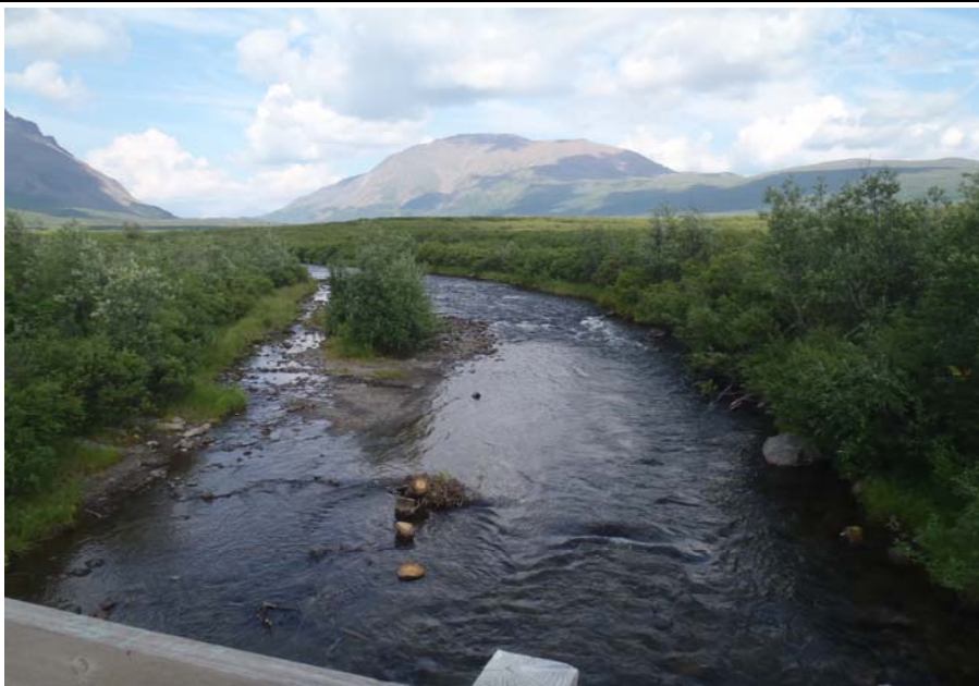
Bridge No. 0684 Br. Name Rock Creek Date 07/14/17 Inspector Murray / Knapp Frame 3 Looking US
