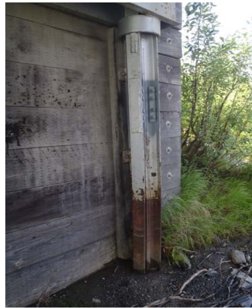
Bridge No. 0684 Br. Name Rock Creek Date 07/14/17 Inspector Murray / Knapp Frame 14 Abutment 1, repaired pile
