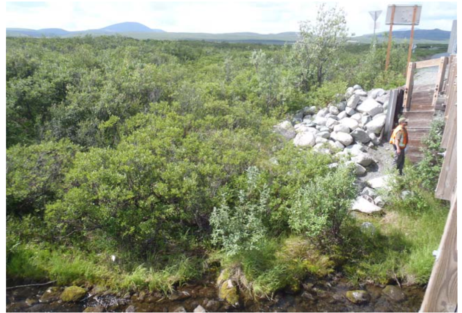
Bridge No. 0684 Br. Name Rock Creek Date 07/14/17 Inspector Murray / Knapp Frame 6 DS NE Bank
