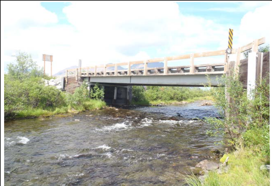
Bridge No. 0684 Br. Name Rock Creek Date 07/14/17 Inspector Murray / Knapp Frame 12 FE DS elevation
