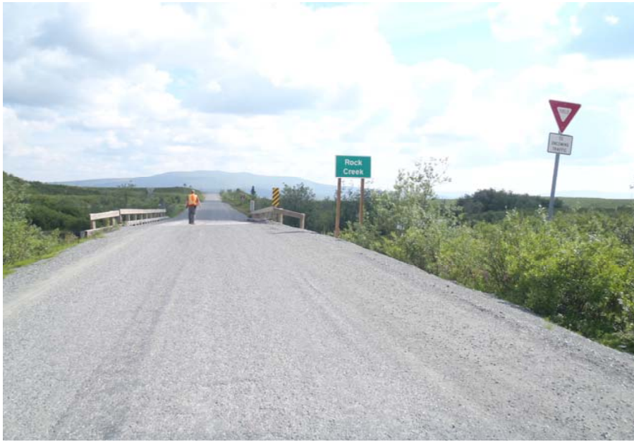
Bridge No. 0684 Br. Name Rock Creek Date 07/14/17 Inspector Murray / Knapp Frame 1 Ahead at bridge
