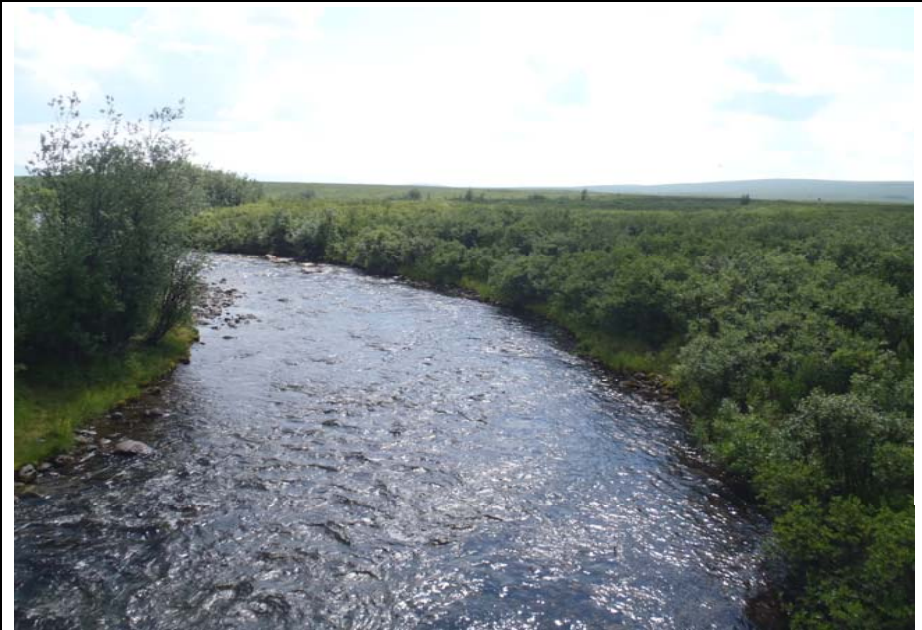
Bridge No. 0684 Br. Name Rock Creek Date 07/14/17 Inspector Murray / Knapp Frame 4 Looking DS
