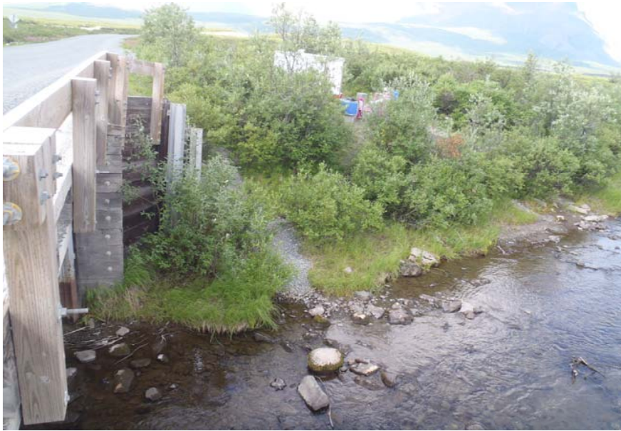
Bridge No. 0684 Br. Name Rock Creek Date 07/14/17 Inspector Murray / Knapp Frame 5 US NE Bank
