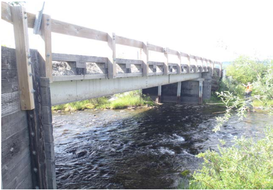
Bridge No. 0684 Br. Name Rock Creek Date 07/14/17 Inspector Murray / Knapp Frame 13 FE US elevation, delete
