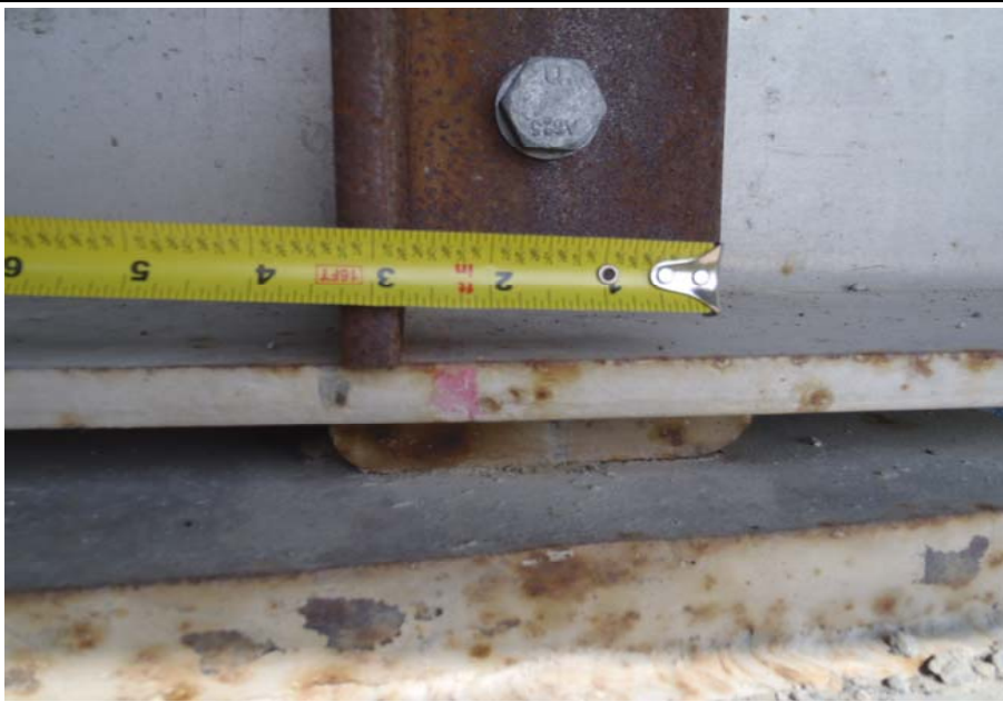
Bridge No. 0684 Br. Name Rock Creek Date 07/14/17 Inspector Murray / Knapp Frame 15 NE DS bearing movement
