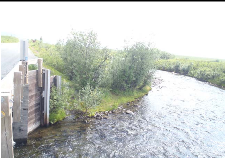
Bridge No. 0684 Br. Name Rock Creek Date 07/14/17 Inspector Murray / Knapp Frame 7 DS FE Bank
