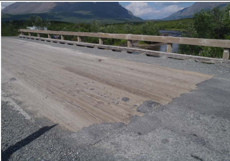
Bridge No. 0684 Br. Name Rock Creek Date 07/14/17 Inspector Murray / Knapp Frame 11 Running planks
