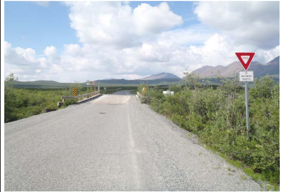
Bridge No. 0684 Br. Name Rock Creek Date 07/14/17 Inspector Murray / Knapp Frame 2 Back at bridge
