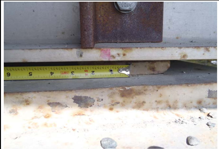
Bridge No. 0684 Br. Name Rock Creek Date 07/14/17 Inspector Murray / Knapp Frame 16 NE DS bearing movement
