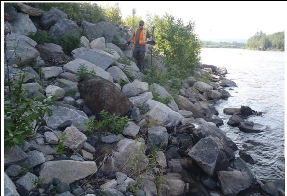
Bridge No. 0574 Br. Name Gulkana River Date 07/14/17 Inspector Murray / Knapp Frame 28 FE riprap slope
