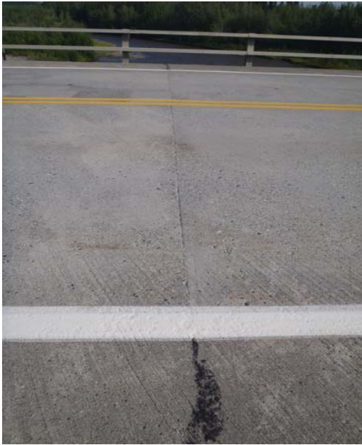
Bridge No. 0574 Br. Name Gulkana River Date 07/14/17 Inspector Murray / Knapp Frame 13 Deck cold joint
