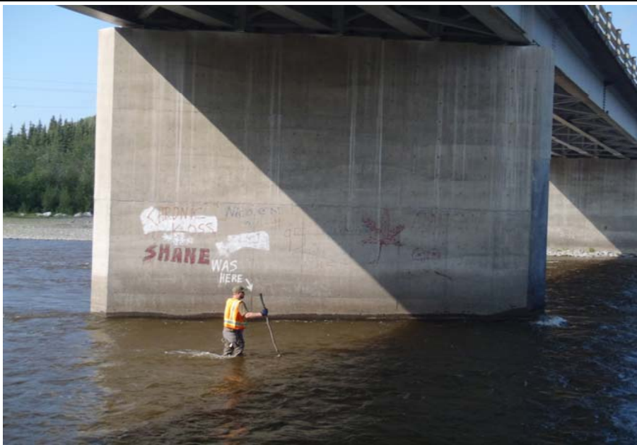
Bridge No. 0574 Br. Name Gulkana River Date 07/14/17 Inspector Murray / Knapp Frame 23 Probing pier 3
