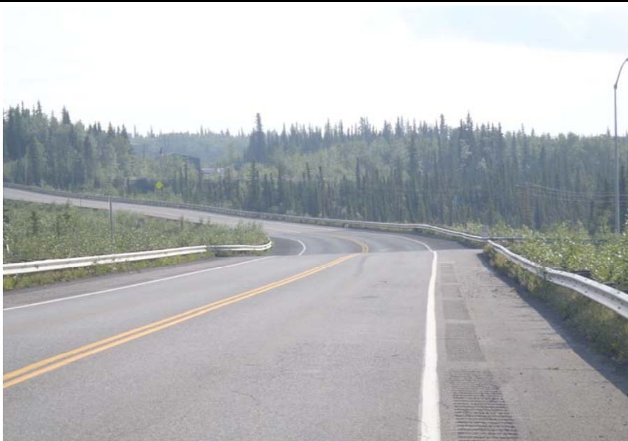
Bridge No. 0574 Br. Name Gulkana River Date 07/14/17 Inspector Murray / Knapp Frame 27 FE rail extends far from bridge
