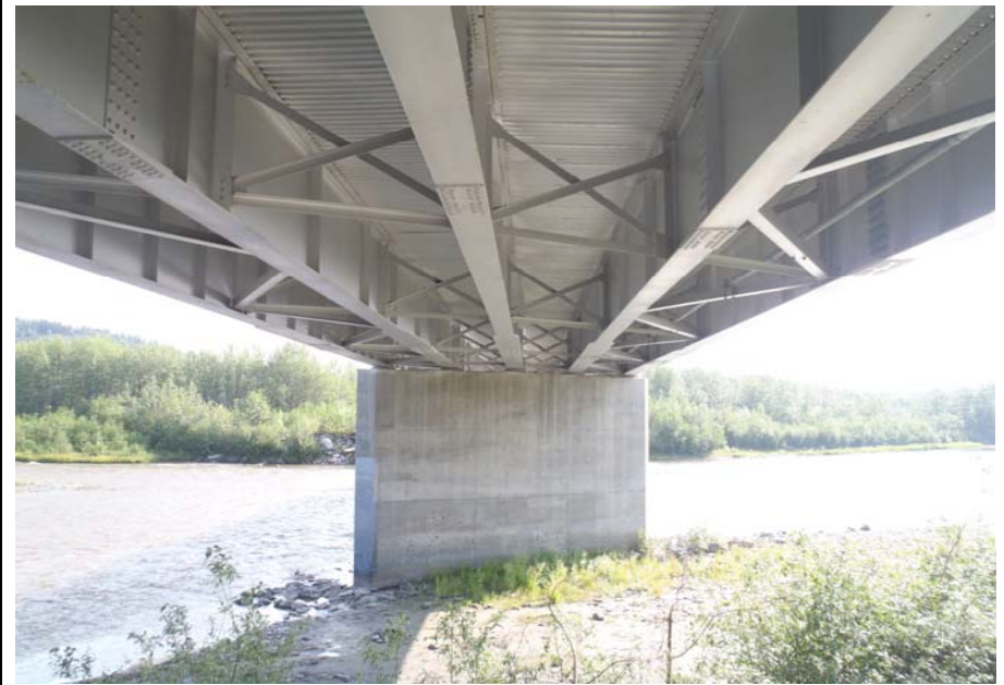
Bridge No. 0574 Br. Name Gulkana River Date 07/14/17 Inspector Murray / Knapp Frame 20 NE Pier 2 underside view
