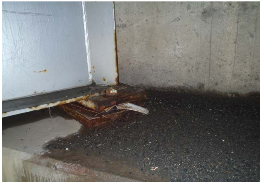
Bridge No. 0574 Br. Name Gulkana River Date 07/14/17 Inspector Murray / Knapp Frame 19 NE bearing, typ.
