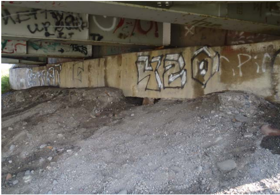
Bridge No. 0574 Br. Name Gulkana River Date 07/14/17 Inspector Murray / Knapp Frame 25 FE abutment with exposed piles
