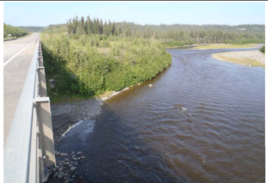
Bridge No. 0574 Br. Name Gulkana River Date 07/14/17 Inspector Murray / Knapp Frame 8 Looking US FE
