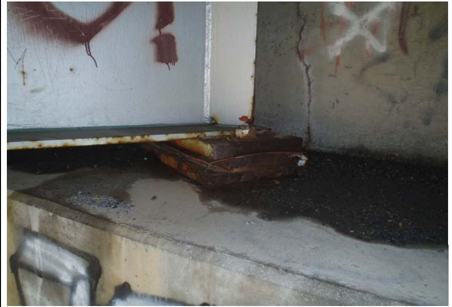
Bridge No. 0574 Br. Name Gulkana River Date 07/14/17 Inspector Murray / Knapp Frame 26 FE bearing, typ.
