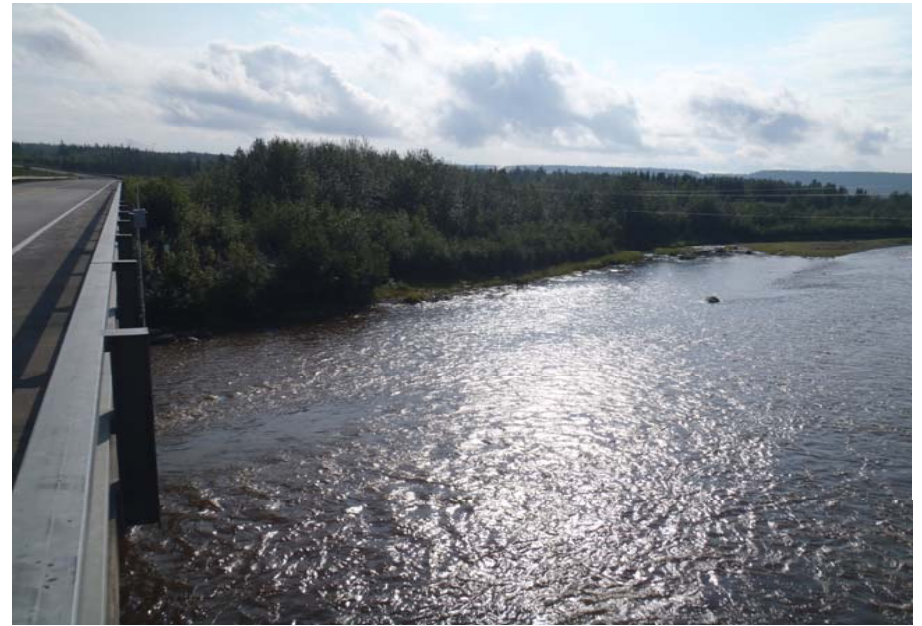
Bridge No. 0574 Br. Name Gulkana River Date 07/14/17 Inspector Murray / Knapp Frame 6 Looking DS NE
