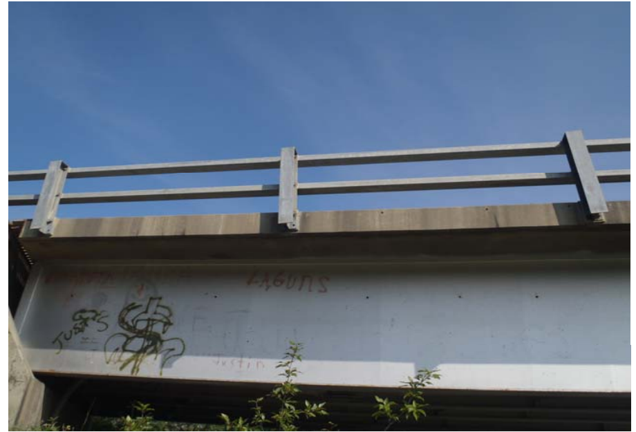
Bridge No. 0574 Br. Name Gulkana River Date 07/14/17 Inspector Murray / Knapp Frame 14 NE DS rail posts tilted
