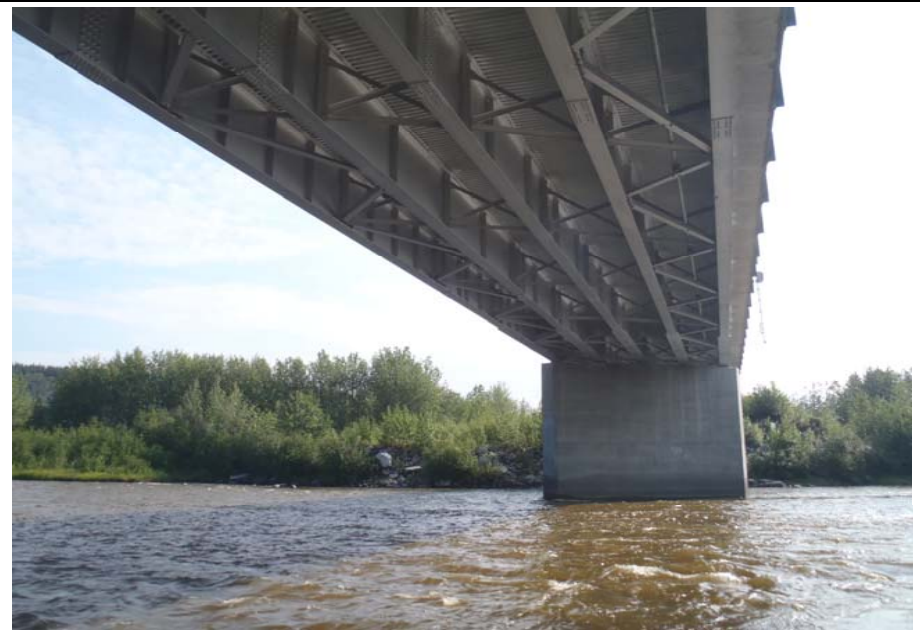
Bridge No. 0574 Br. Name Gulkana River Date 07/14/17 Inspector Murray / Knapp Frame 24 Pier 3
