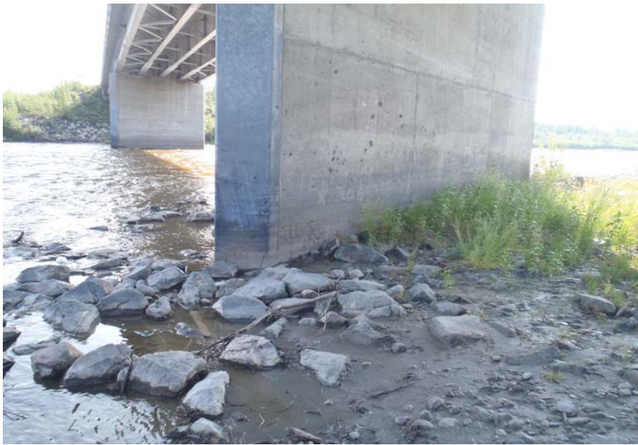
Bridge No. 0574 Br. Name Gulkana River Date 07/14/17 Inspector Murray / Knapp Frame 21 NE US Pier 2
