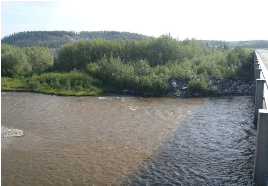
Bridge No. 0574 Br. Name Gulkana River Date 07/14/17 Inspector Murray / Knapp Frame 5 Looking US NE
