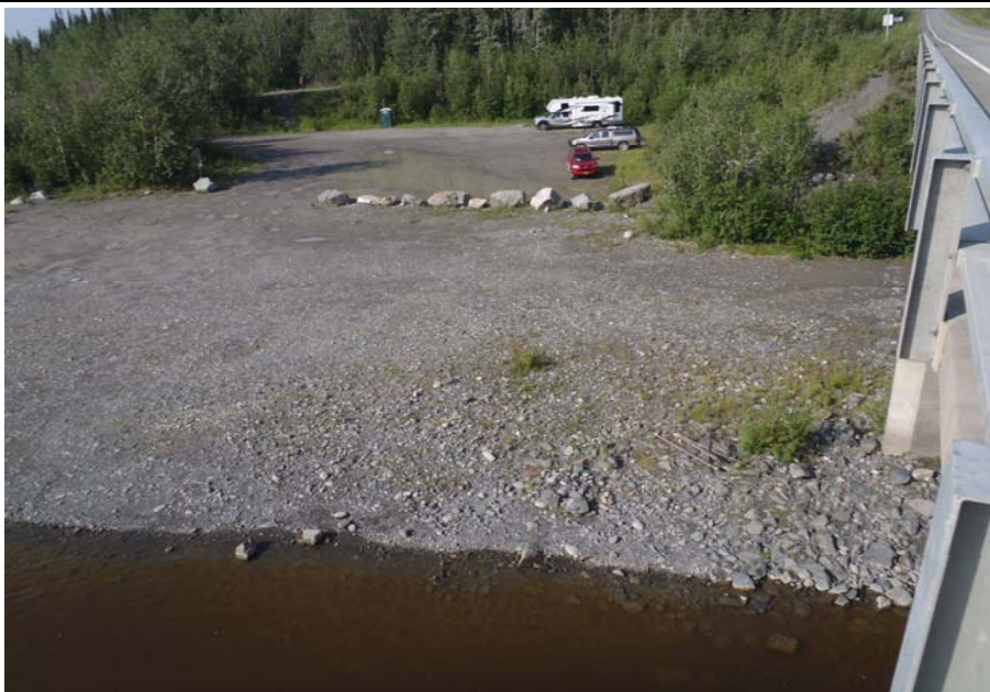
Bridge No. 0574 Br. Name Gulkana River Date 07/14/17 Inspector Murray / Knapp Frame 7 Looking DS FE
