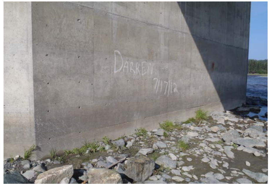
Bridge No. 0574 Br. Name Gulkana River Date 07/14/17 Inspector Murray / Knapp Frame 22 FE Pier 2
