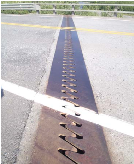
Bridge No. 0574 Br. Name Gulkana River Date 07/14/17 Inspector Murray / Knapp Frame 11 NE joint
