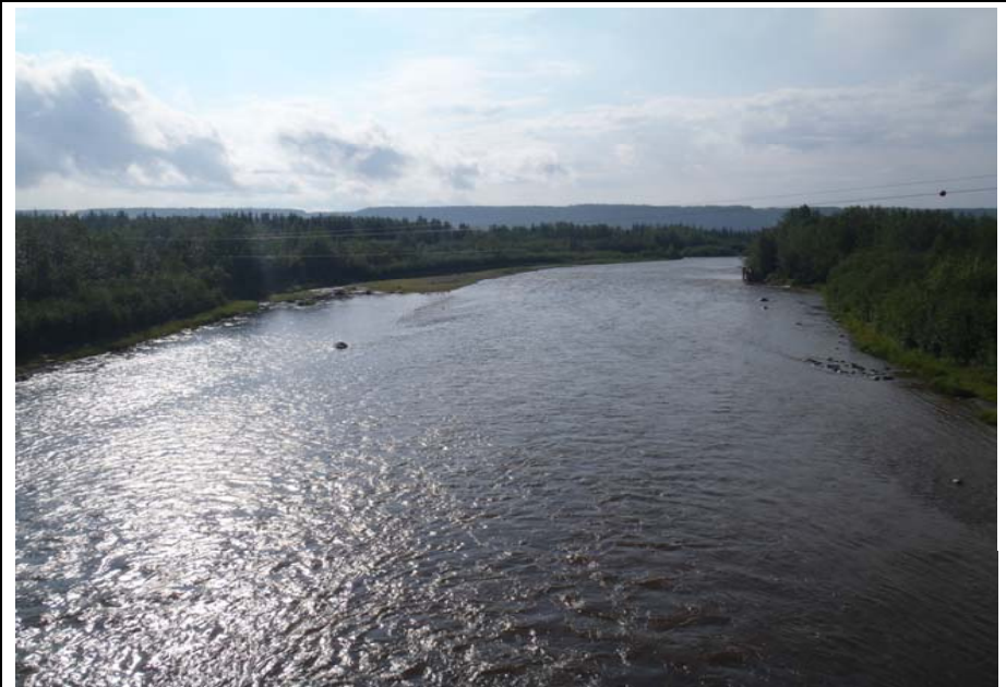
Bridge No. 0574 Br. Name Gulkana River Date 07/14/17 Inspector Murray / Knapp Frame 4 Looking DS
