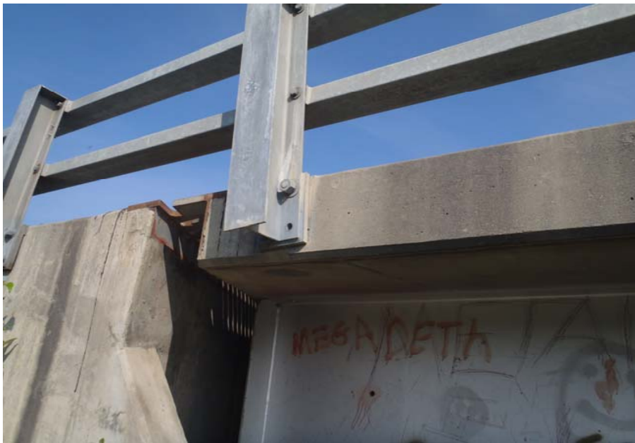
Bridge No. 0574 Br. Name Gulkana River Date 07/14/17 Inspector Murray / Knapp Frame 15 NE DS railing missing bolts
