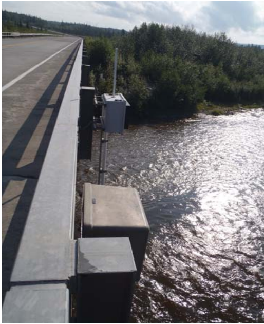
Bridge No. 0574 Br. Name Gulkana River Date 07/14/17 Inspector Murray / Knapp Frame 9 Hydrologic monitoring on bridge
