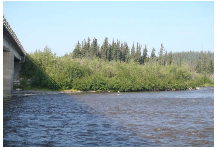
Bridge No. 0574 Br. Name Gulkana River Date 07/14/17 Inspector Murray / Knapp Frame 16 US NE dike
