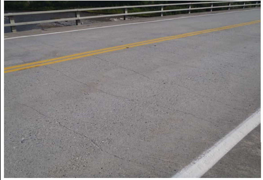
Bridge No. 0574 Br. Name Gulkana River Date 07/14/17 Inspector Murray / Knapp Frame 10 Deck cracks, typ.
