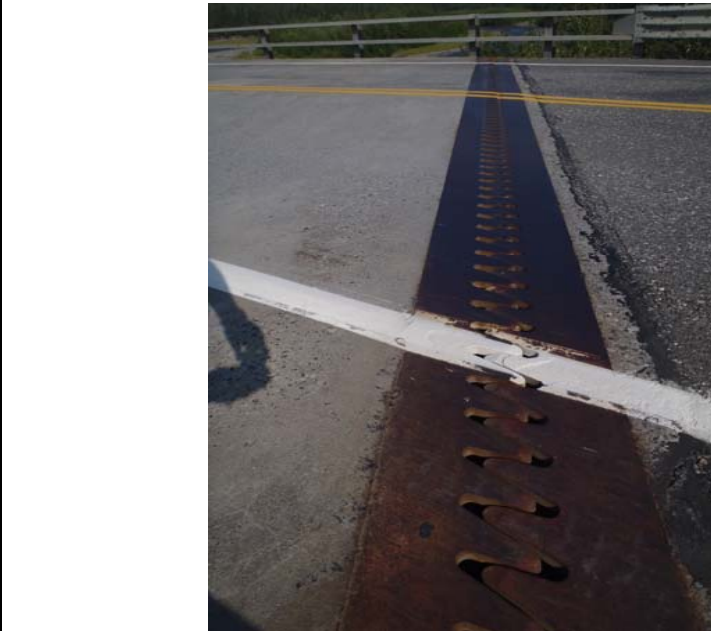
Bridge No. 0574 Br. Name Gulkana River Date 07/14/17 Inspector Murray / Knapp Frame 12 FE joint
