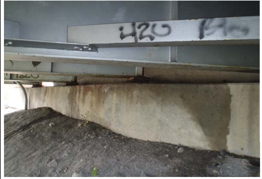
Bridge No. 0574 Br. Name Gulkana River Date 07/14/17 Inspector Murray / Knapp Frame 18 NE abutment
