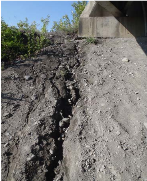
Bridge No. 0574 Br. Name Gulkana River Date 07/14/17 Inspector Murray / Knapp Frame 17 NE Surface drainage causing rill
