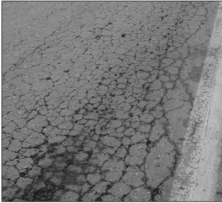
Figure 4-5. Advanced Alligator Cracking of Highway Pavement
