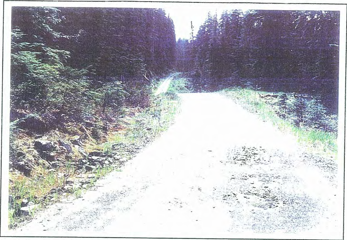
Photo 1 : Typical roadway section to Shelter Cove road system. Note poor vertical roadway alignment.
