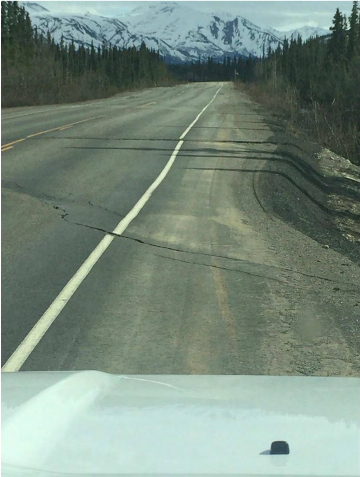
Figure 12 – Drainage issues and damaged pavement around MP 235.5
