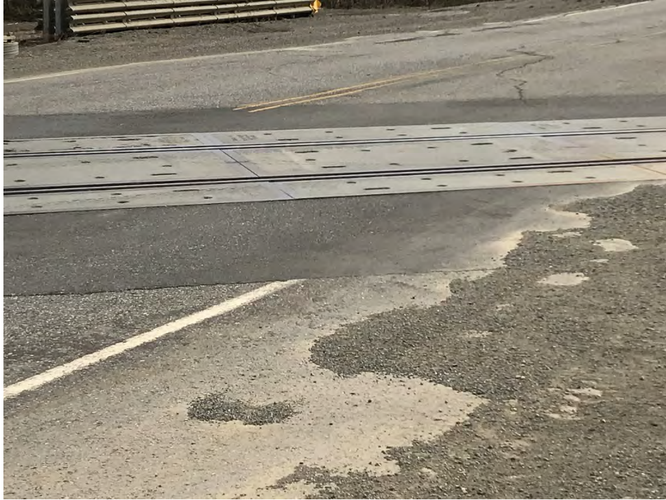
Figure 10 - Surface patches along railroad crossing
