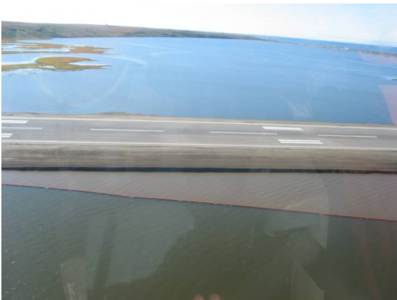
Figure 7 The runway safety area of the existing runway is being widened. Note the silt curtain being used to control the sediment.
