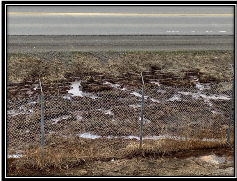
Figure 32: Saturated Land, RW 1 End Looking Southeast
