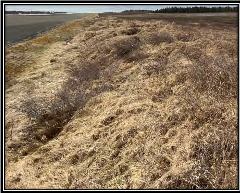
Figure 14: Surface Irregularities in the Tundra Surrounding the Airport Embankment
